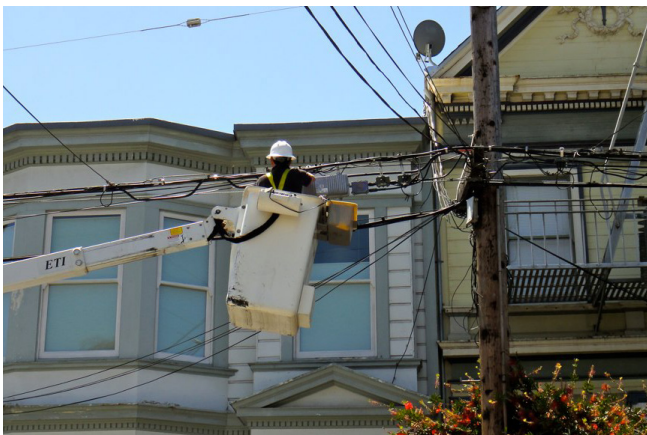
Photo 8.3 PG&E transmission lines. Lynn Friedman (CC BY-NC-ND 2.0)
