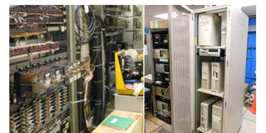
Automatic Train Control System
