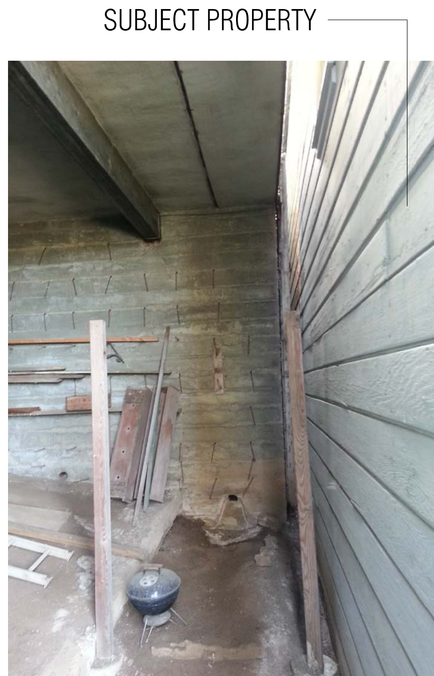
(4) LOOKING WEST AT VOID UNDER 121 MANCHESTER
