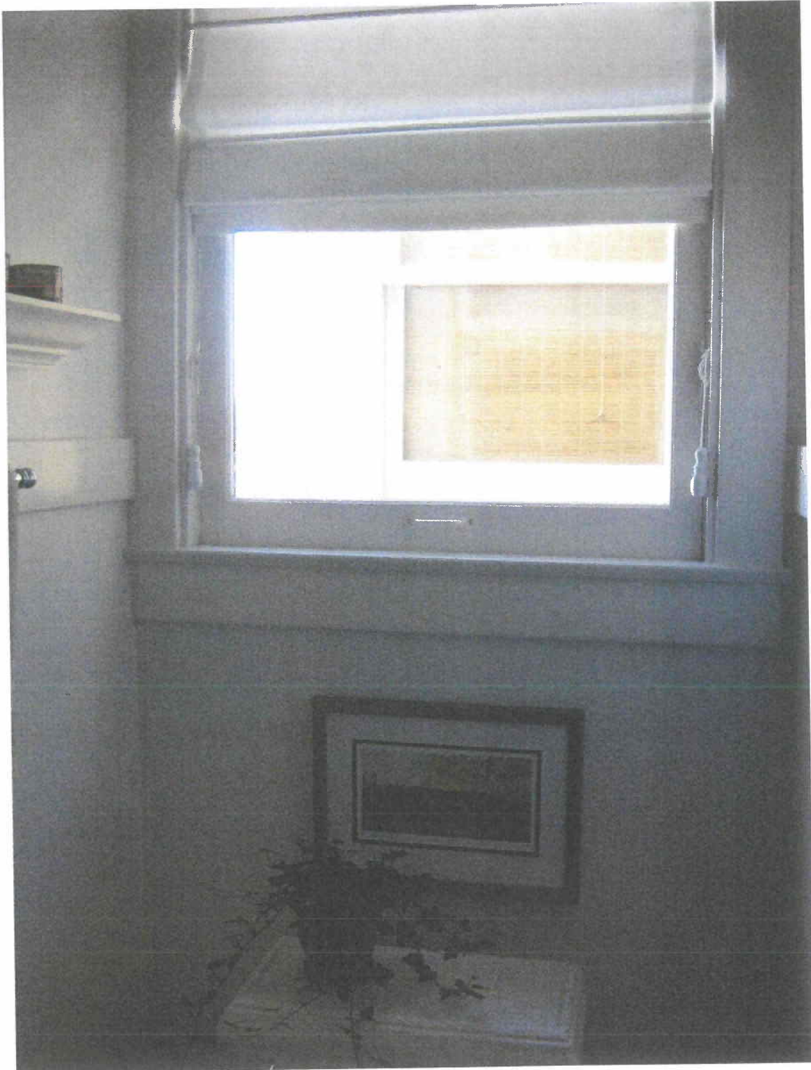
SE view from 33 Sutro Hts bathroom light well to 27-29 Sutro Hts (left side)
