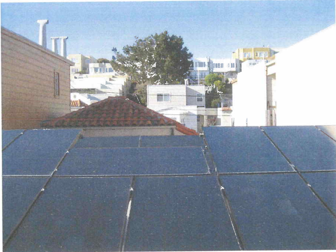
N view of Two Solar Arrays on 33 Sutro Hts roof Between Buildings 27-29 (R) and 39-41 Sutro Hts (L)
