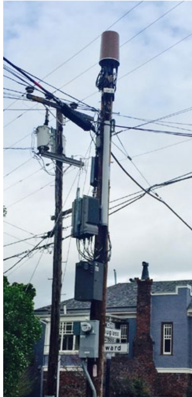
ABOVE: Disfavored example of cabling that is cluttered & tangled. Riser not painted.
