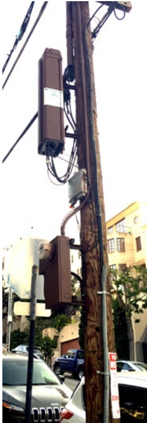
Disfavored wide offset (from pole) of electric meter, unpainted fiber (PBX) node box (green element) and large white RF warning sticker on non-RF emitting equipment enclosure.
