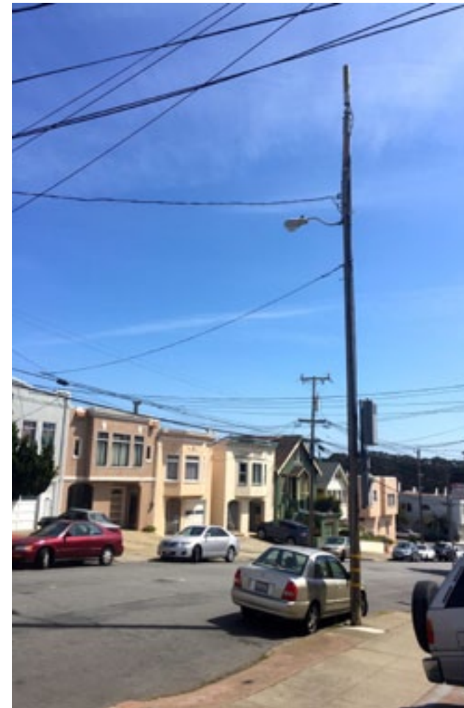
TOP: Preferred installation: 1) Equipment boxes and antennas that are painted gray, and are not bulky in appearance. 2) No cluttered cabling is present, though the cabling near the antenna should be painted gray as well. 3) Relatively slim profile antenna.
