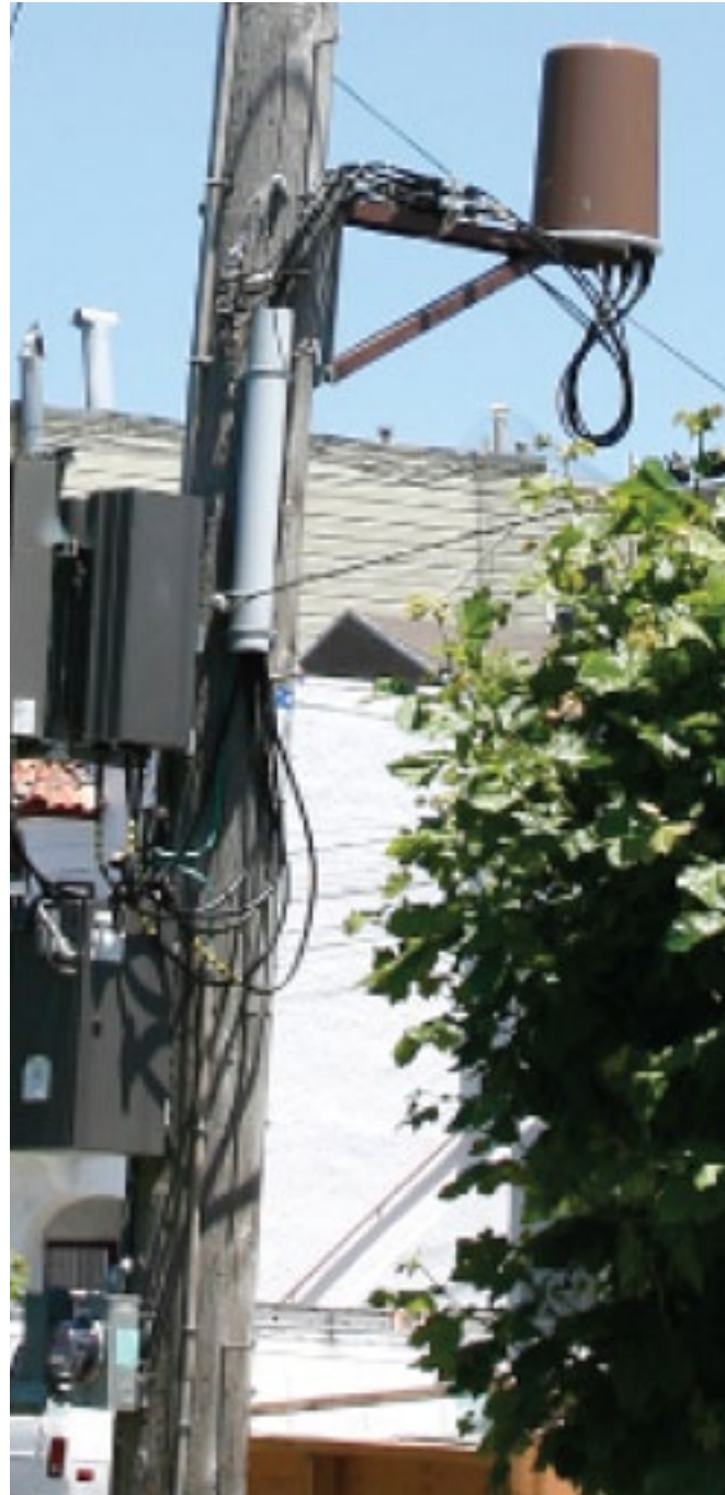
ABOVE: Disfavored excess loose cabling, excess decals/stickers, and cluttered appearance of equipment cabinets.
