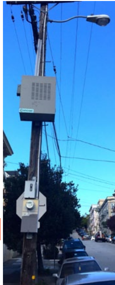
ABOVE: Please note, some of the square boxes mounted on poles in San Francisco, similar to the one shown in the photo above, are also used for non-wireless providers, such as cable television. These boxes are typically used to boost power and increase signal quality for wired communications.
