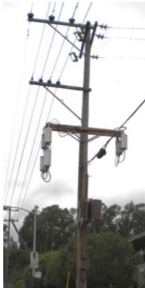
LEFT: Disfavored use of multiple panel antennas with cables looping below each panel.
