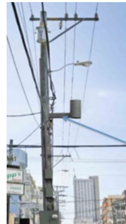
Antenna mounting arm with cabling and other electronic elements screened from view inside bracket
