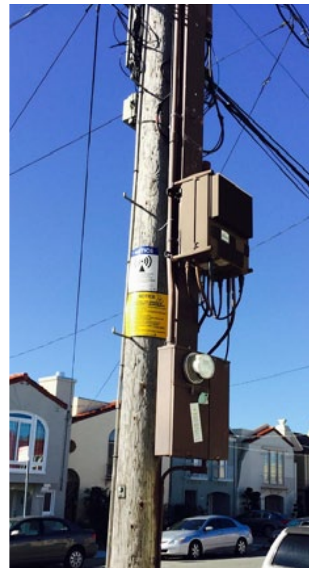
LEFT: Non-recommended, repetitive, and highly visible RF warning stickers, and equipment manufacturer decals located near bottom of pole and visible to pedestrians.
