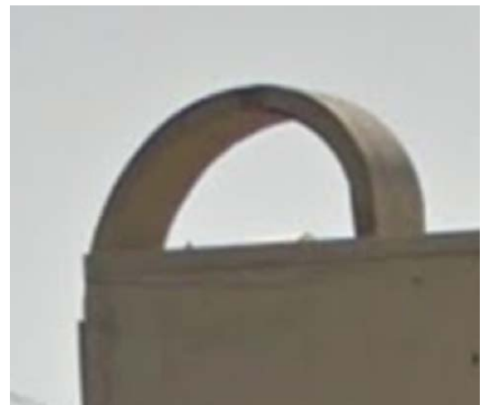
Photo on the right: Disfavored wide cable tray arc over parapet
