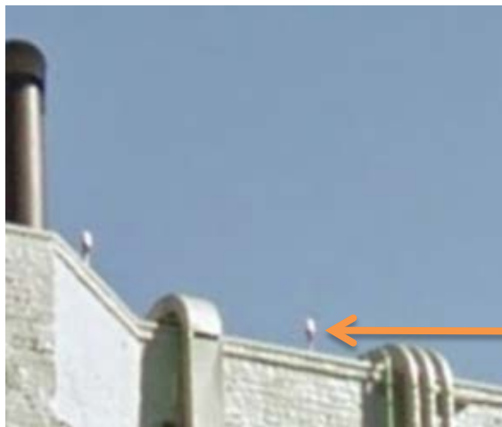
Example of visible GPS antennas (white elements) that should be moved away from roof edges
