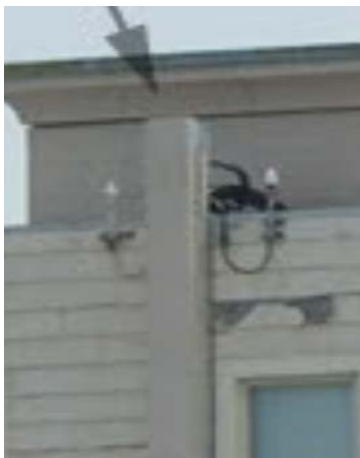
Photo on the left: Disfavored cable tray rising above parapet and visible GPS antennas
