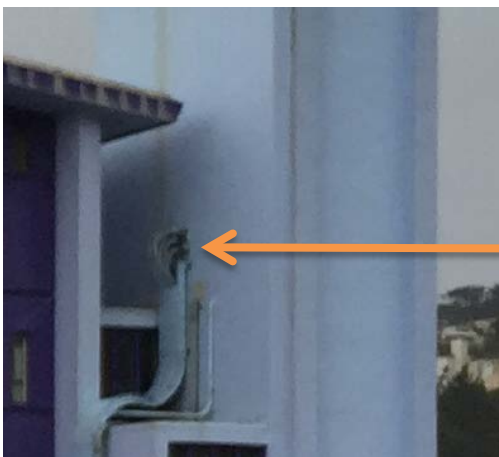
Disfavored example with cabling not shrouded at entry point
