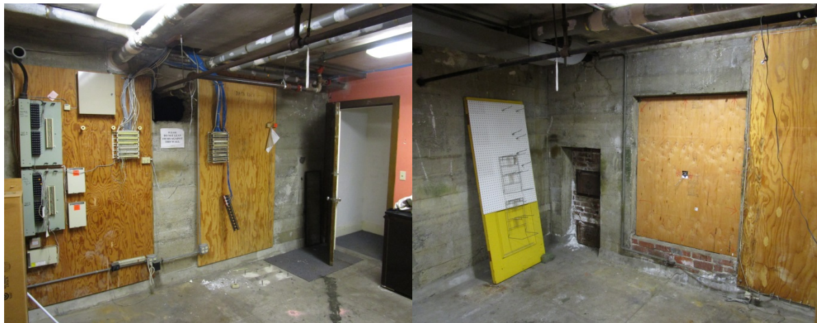
Basement mechanical rooms.
