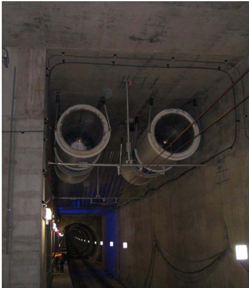
Figure 6: Example of Jet Fans near a Tunnel Portal
