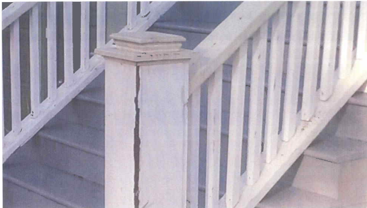
Detail of front steps to be repaired/replaced (scope 4)
