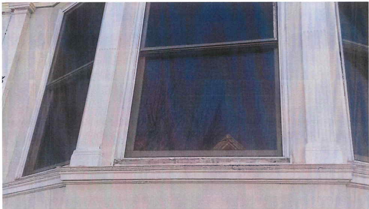
BELOW: Detail of lower vinyl windows to be replaced (scope 2)
