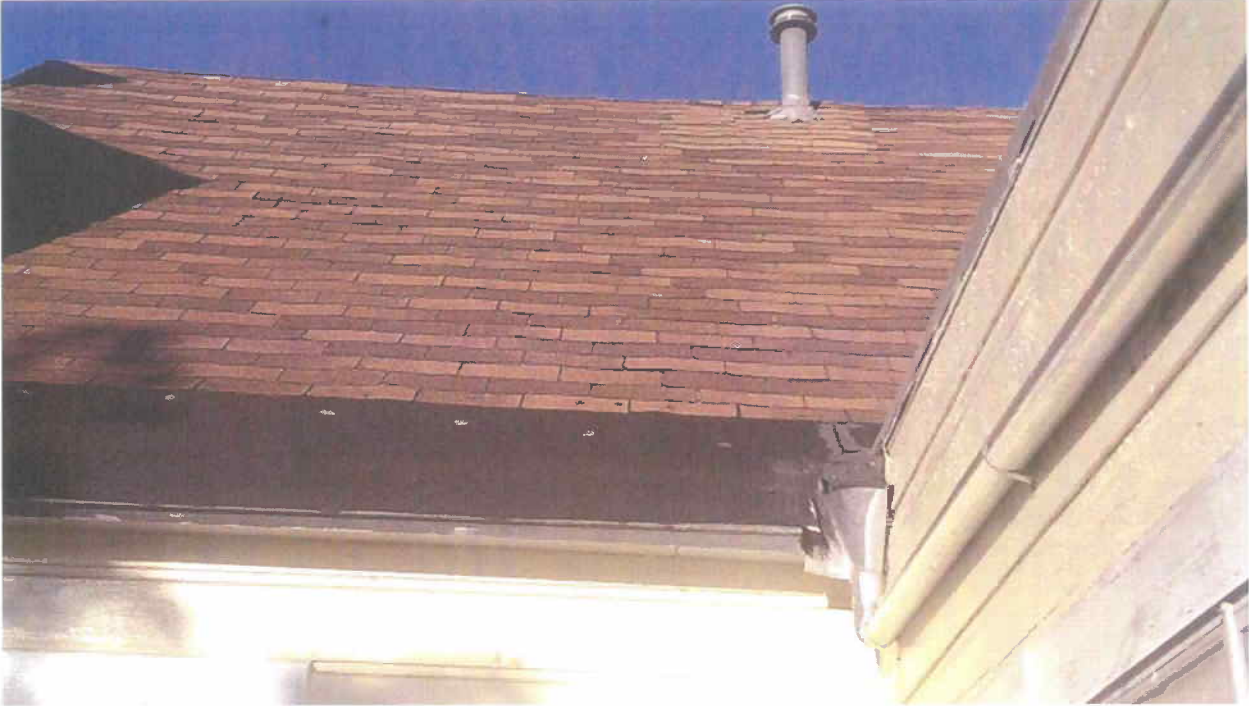
Detail of rear roof as well as repairs made to guttering under scope 1
