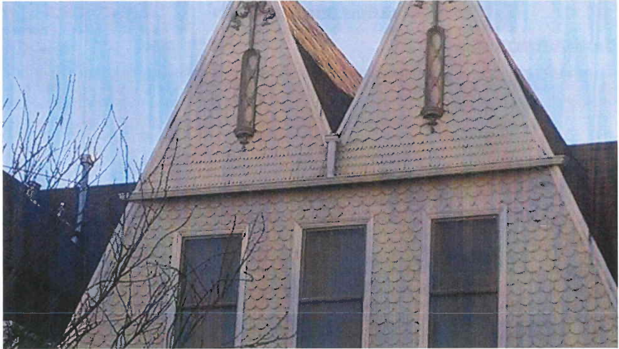
ABOVE: Detail of repaired guttering (scope 1) as well as upper vinyl windows to be replaced (scope 2)
