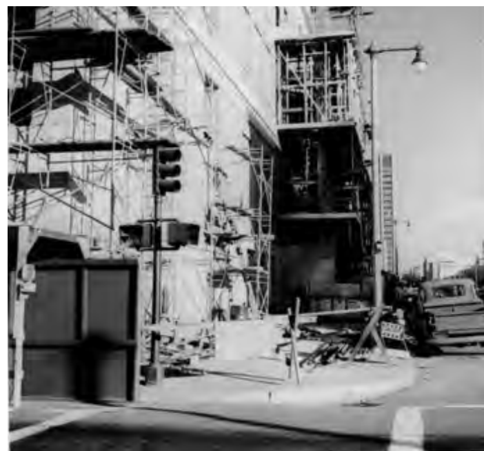
Figure 2.79 undated photo of work being completed on Civic Auditorium (San Francisco History Center, San Francisco Public Library)
