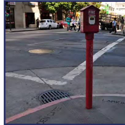
Fire box at Golden Gate Ave and Larkin St
