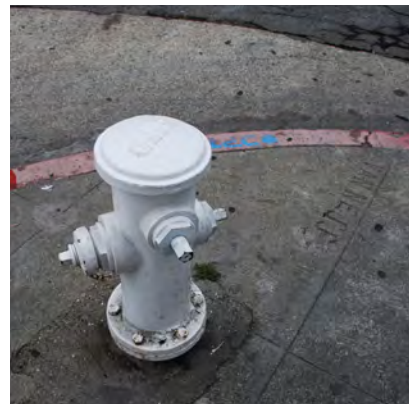
Low pressure hydrant at Redwood St
