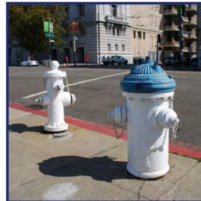
Low pressure fire hydrant and high pressure auxiliary water supply hydrant at Grove St
