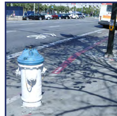
High pressure auxiliary water supply hydrant along Larkin St
