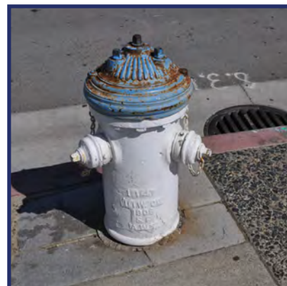
High pressure auxiliary water supply hydrant at Larkin St
