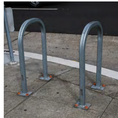
Bike rack - metal staple style, installed incorrectly along Grove St
