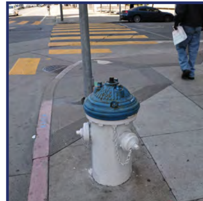
High pressure auxiliary water supply hydrant along Polk St
