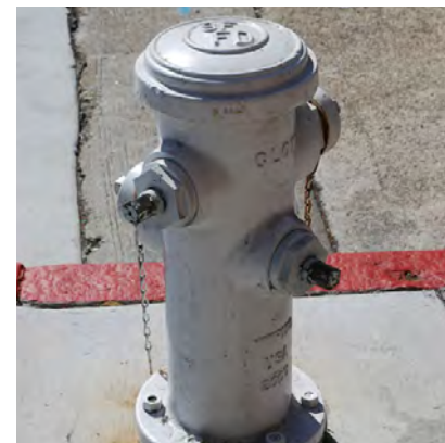
Low pressure hydrant along Franklin St
