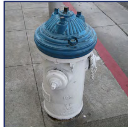
High pressure auxiliary water supply hydrant along Grove St
