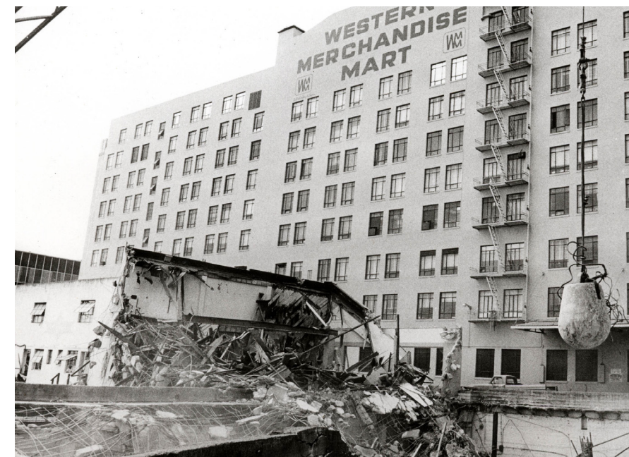
Demolition in preparation for Mart 2 construction with view of Stevenson Street facade, 1973 (Market Square Archives)
