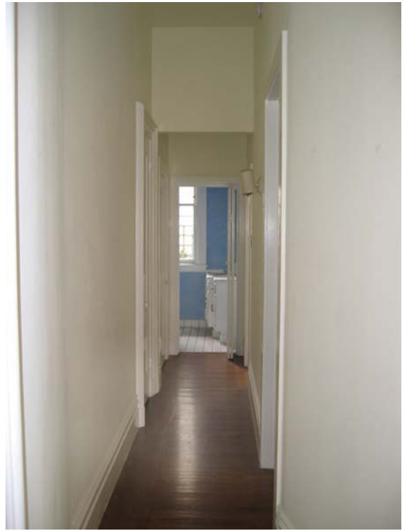
Wall at left of photo could be opened up to stair, making both stair and hallway much less claustrophobic. Hardwood floors with borders on lower level, softwood on upper, further indicating the units were originally two levels.
