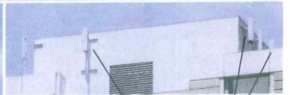
proposed replacement antennas
