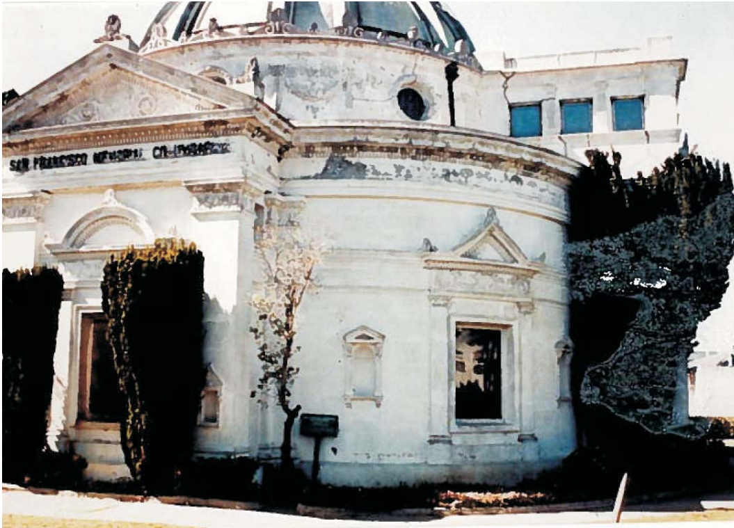
THE COLUMBARIUM in its dilapidated state prior to its purchase by the Neptune Society of Northern California
