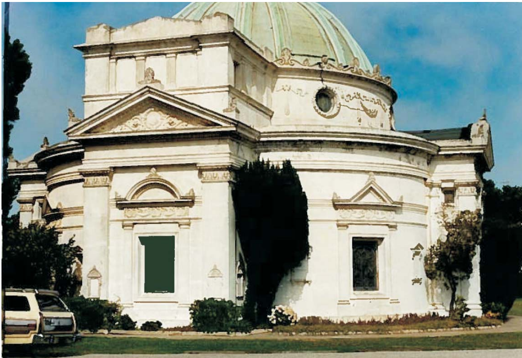
THE COLUMBARIUM in its dilapidated state prior to its purchase by the Neptune Society of Northern California
