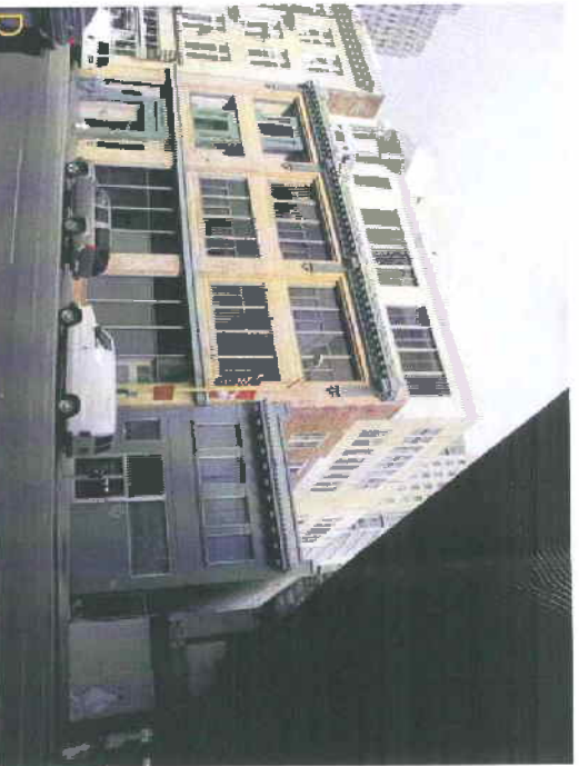
Photo D shows the Southeastern facade of 564 & 568 Howard, taken from across the street, under the Elevated Transbay Loop.
