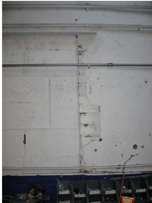
1661 Pacific Avenue, detail of concrete and masonry of east wall. Page & Turnbull, March 2008.
