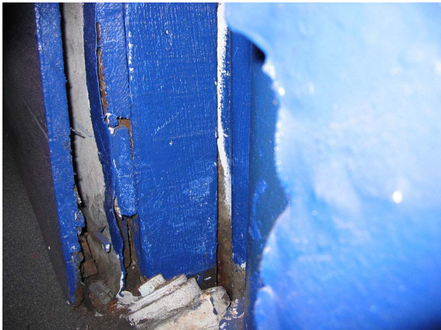
1661 Pacific Avenue, detail of wood framing of west wall. Page & Turnbull, March 2008.
