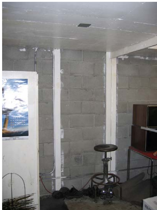
1661 Pacific Avenue, detail of concrete blocks of south wall. Page & Turnbull, March 2008.
