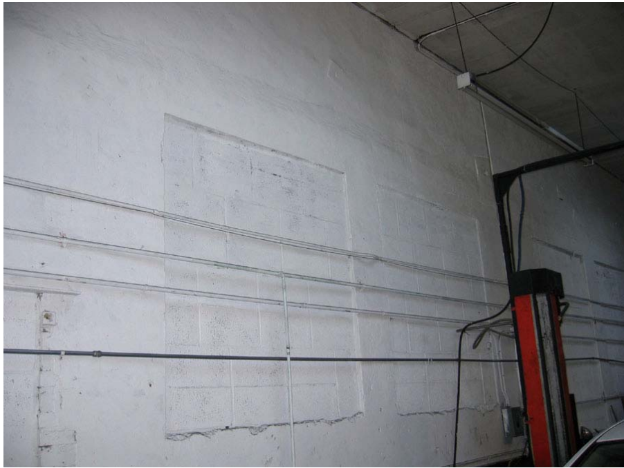
1661 Pacific Avenue, detail of east wall. Note: this wall is shared with the adjacent building at 1645 Pacific Avenue. Page & Turnbull, March 2008.
