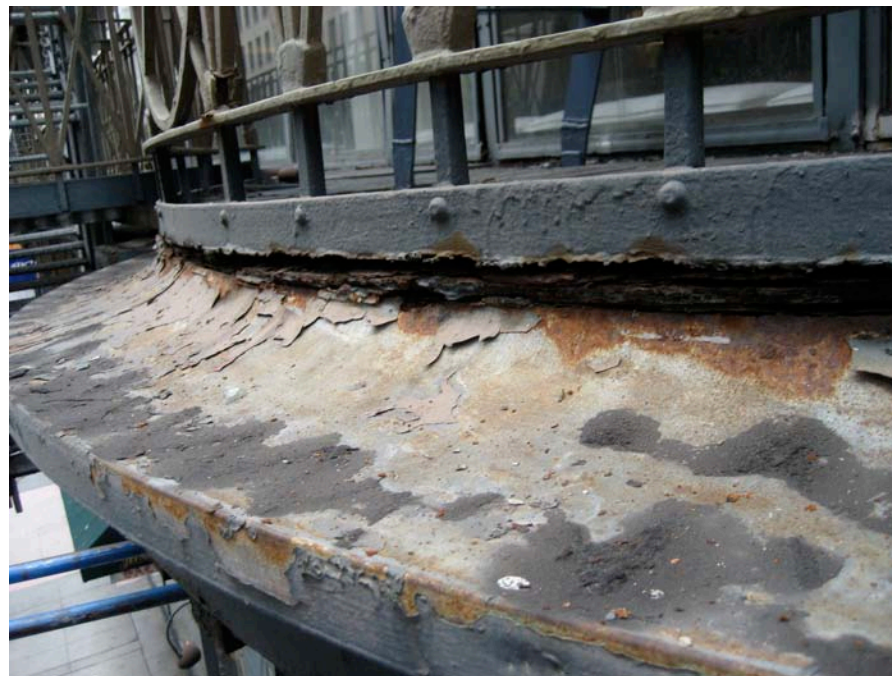
Deterioration at balcony
