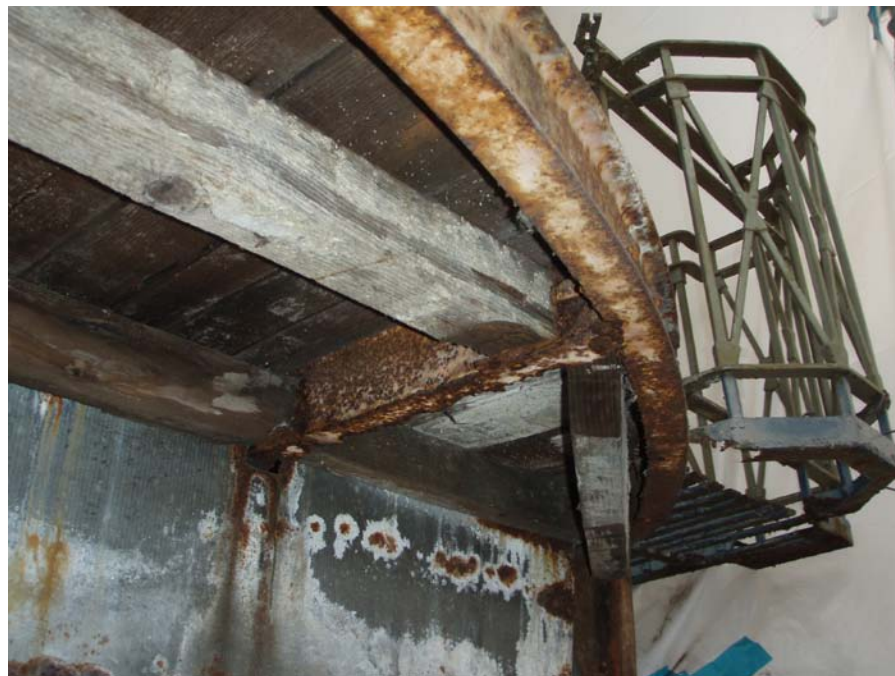
Deterioration at balcony
