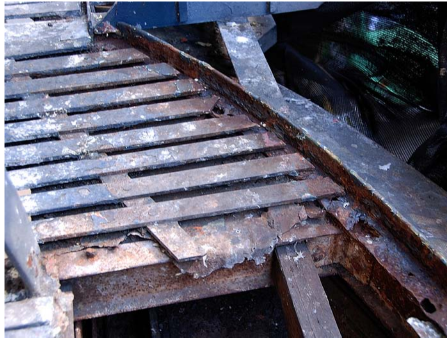
Deterioration at balcony
