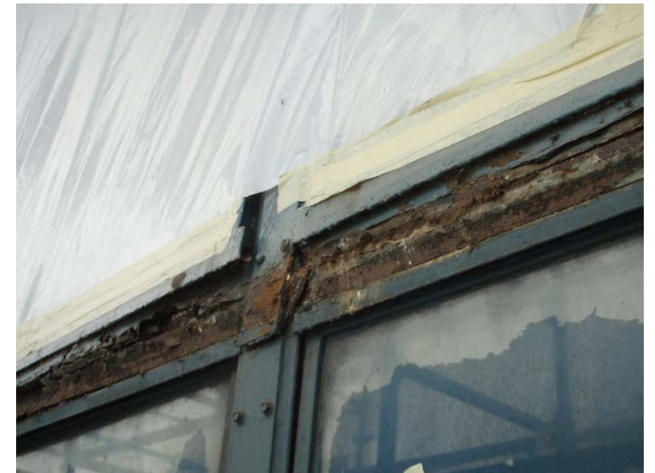
Deterioration at windows
