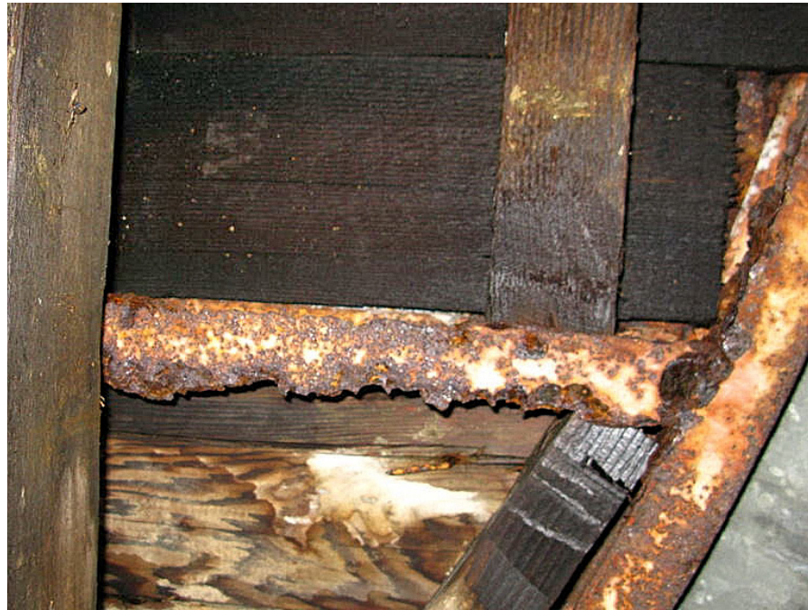
Deterioration at structural framework
