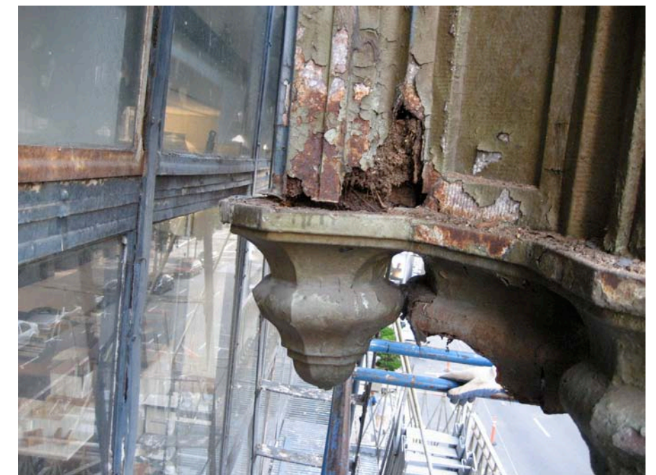
Deterioration at decorative sheet metal
