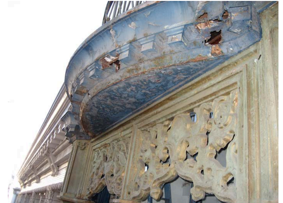
Deterioration at decorative sheet metal
