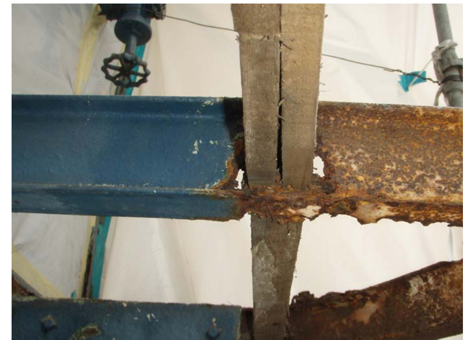
Deterioration of framing
