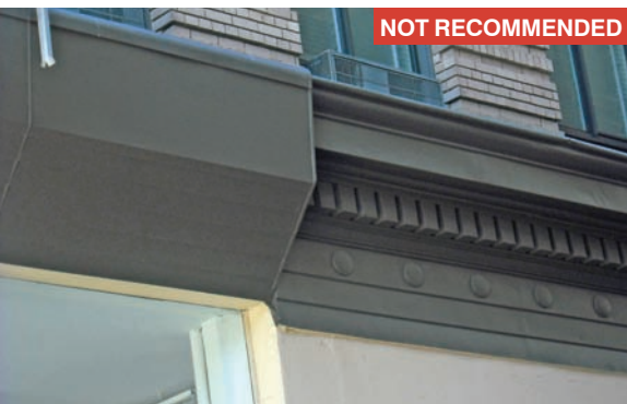
Removing, obscuring, or damaging historic features through installation of new features is discouraged, such as this historic cornice partially concealed with aluminum panels.
