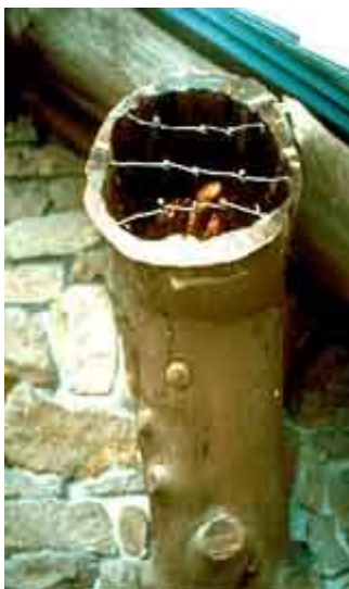
The core of a deteriorated wood outrigger was first drilled out. Photos (left and right): Courtesy, Harrison Goodall.
