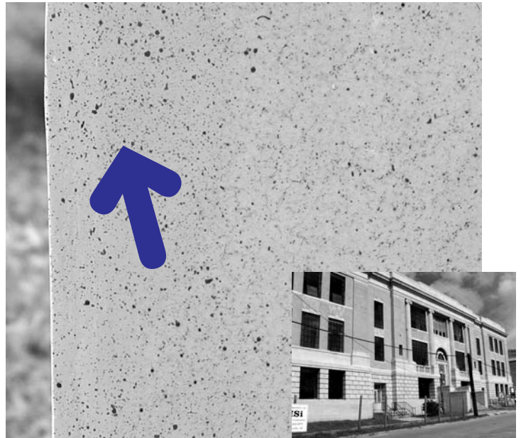
Where's the Repair? Glazed terra cotta spall, upper left corner, filled and smoothed using Thin-Fill 55 prior to glazing and speckling with Aquathane UA210 coatings, matched to original glaze colors. Project is an Historic school restoration in Charleston, SC.
