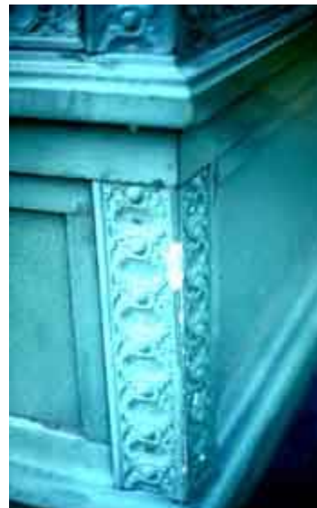
Substitute materials need to be located with care to avoid damage. The fiberglass column base has chipped, whereas the historic cast iron would have remained sound. Photo: NPS files.
