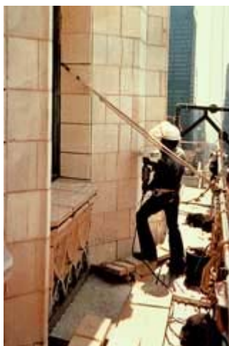
A worker cleans out mortar joints in preparation for repointing the architectural terra-cotta. Photo: NPS files.
