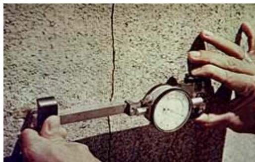
This crack is being measured. Structural cracking, whether static (nonmoving) or dynamic (moving) should be caulked to prevent water entry into the glazed architectural terra-cotta system. Photo: NPS files.
