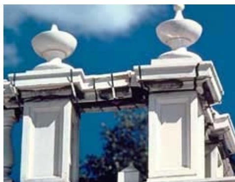
Exposed or freestanding terra-cotta detailing (parapets, urns, balusters, etc.) have traditionally been subjected to the most severe vicissitudes of deterioration as a result of freezing temperatures and water. Photo: NPS files.
