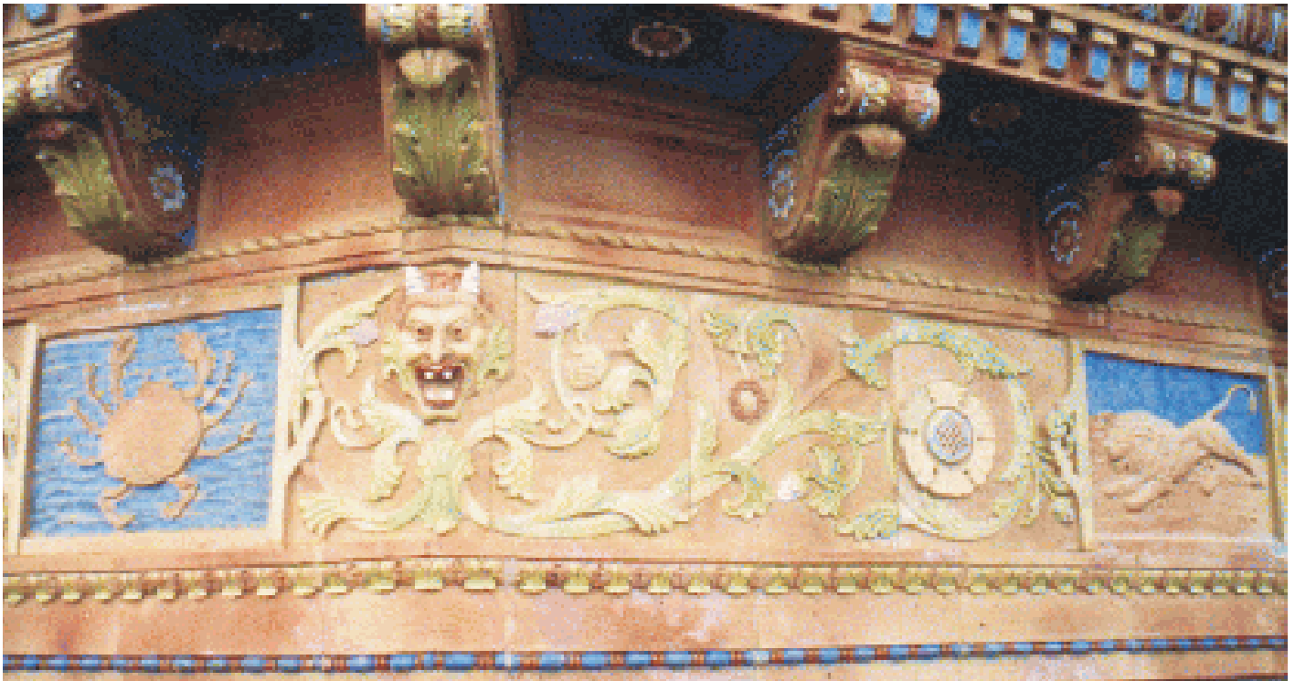
PHOTO, ABOVE: Dozens of custom Aquathane UA210 NCL colors were used to restore decorative terra cotta elements at this Florida museum.
