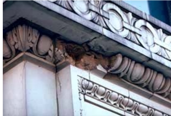
Material spalling is the result of excessive expansion of the porous tile body caused by water and freezing temperatures. This is a serious condition, often difficult to repair. Photo: NPS files.
