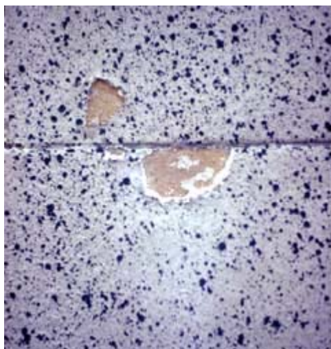
Blistering of the glaze, like crazing, is the result of the increase in water in the porous clay body and the subsequent destruction of the glaze as a result of water migration and pressure. Glaze spalling may also be caused by deterioration of metal anchors behind the terra-cotta unit. Photo: NPS files.
