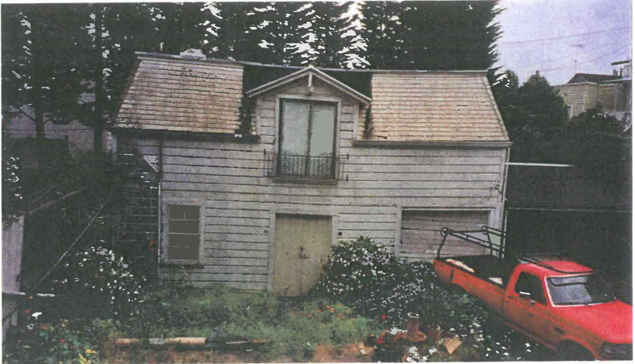
A. Front (Western) Facade of Carriage House (Note sag towards center of roofline.)
