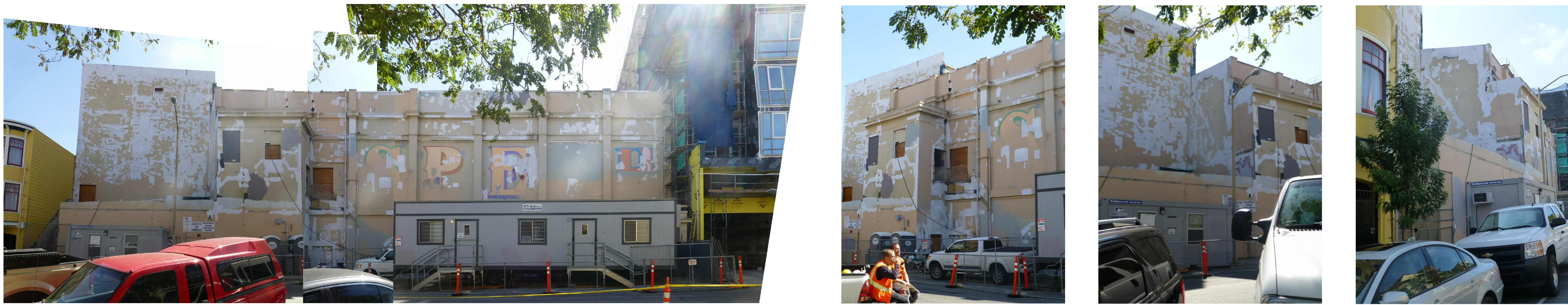
3 EXISTING CONDITIONS AT WEST (REAR) ELEVATION AT BARTLETT STREET NOT TO SCALE
