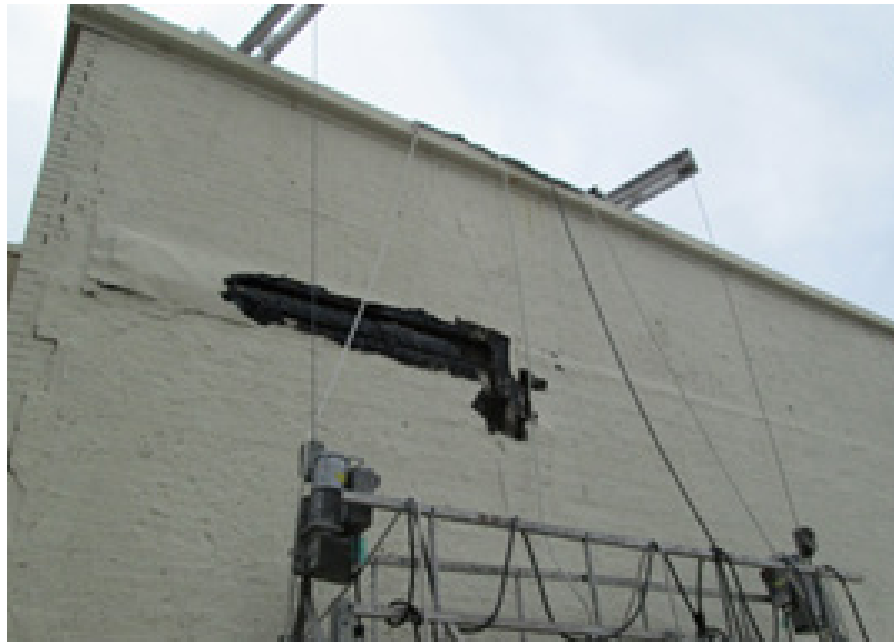
Previous repair at Annex Wall
