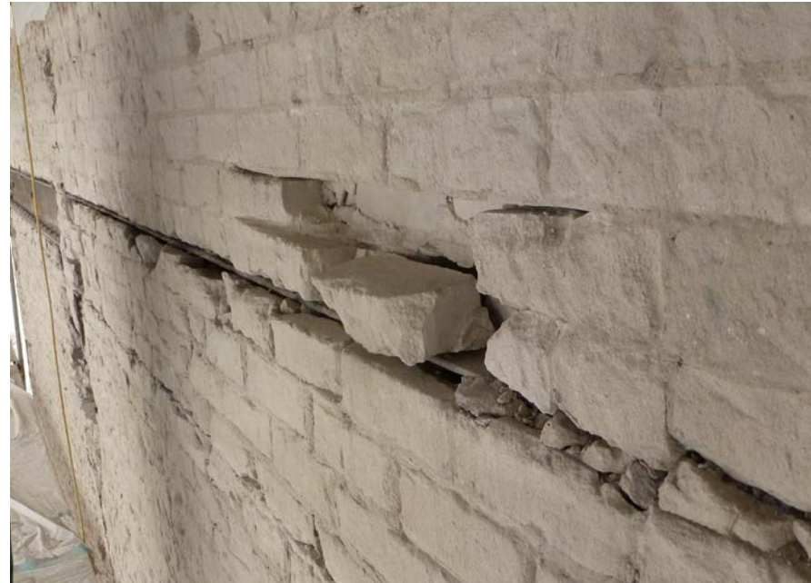
Photo of deteriorated brick at Annex wall
