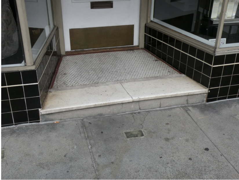
Figure 17 Original marble step and mosaic tile landing at 190 Gough Street. All five thresholds on the façade retain their original marble and tile finishes. Note the black tile with weather course that runs the length of the façade.
