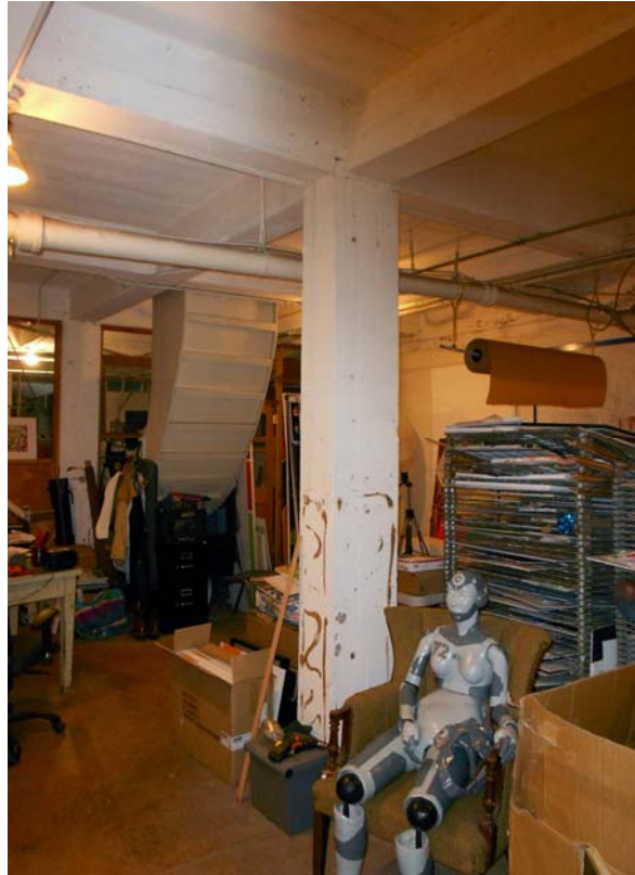
Figure 18. Interior view south in basement showing concrete clad steel post-and-beam construction. [No. 16.07.29] January 2014.
