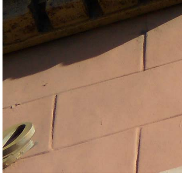
Figure 4. Detail of upper portion of façade showing flat terra cotta units imitating masonry blocks. [No. 17.21.19] February 2014
