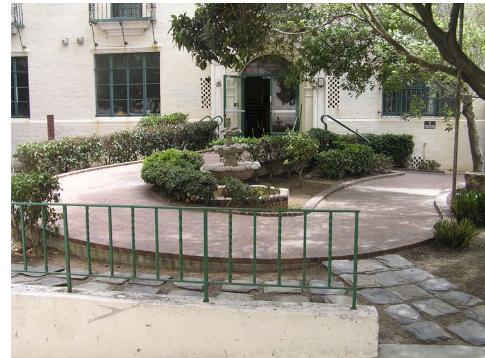
Existing non-compliant brick ramp with concrete stair at East Entry.
