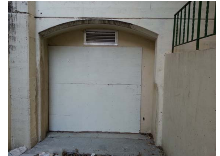
Image 11 – View of basement driveway opening with non-historic infill wall looking north at the north wing. (Knapp, 2013)
