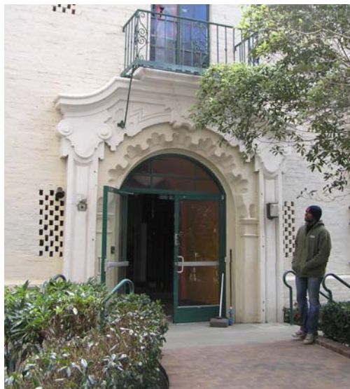
Image 8 – View of decorative arched entry at east wing looking east. The lower portion of original pilasters has been covered where the non-historic brick ramp and concrete steps were installed and interior steps were infilled with new floor to meet the ramp landing. (Knapp, 2013)
