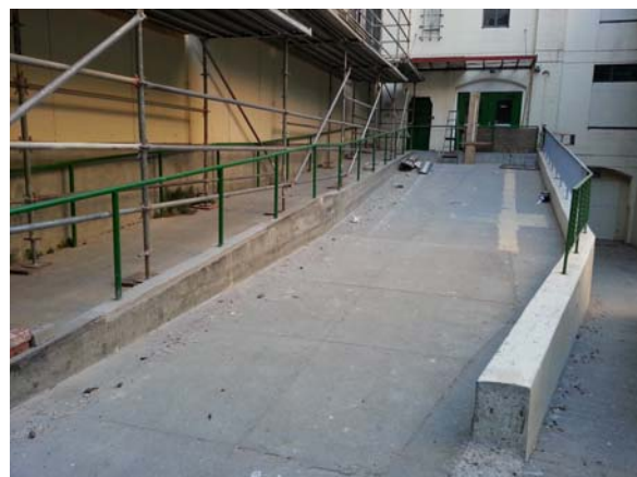
Images related to work under separate permits: Top row - repair of exterior brick and concrete at facades, steel sash windows, wrought iron (A36) and galvanized steel window grilles; Middle row - replacement of non-historic signage and replacement of exterior North Wing ramps at west side of courtyard; Bottom row - repair of historic main stair and finishes at East Wing Lobby.
