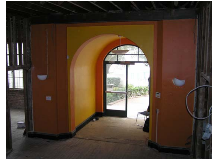
Image 9 – View of lobby entry at east wing looking southwest. Non-historic storefront assembly and infill flooring at modified entry. (Knapp, 2013)
