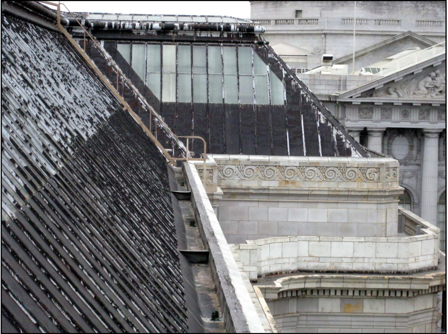
Veterans Building, View of Deteriorated Leaded-Cooper Roof Panels
