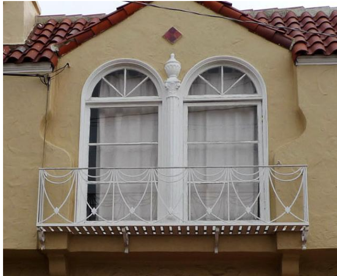
Detail of distinctive recessed windows and flanking sculpted wall projections at 2258 34 th Avenue. The building retains original fenestration and horizontal muntin pattern.
