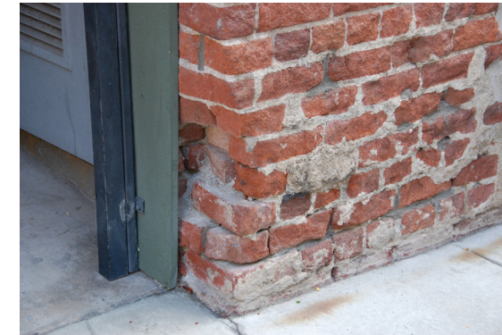
Brick damage at base
