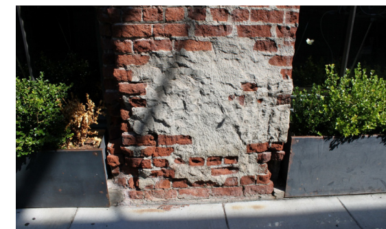
Area where cement plaster was not entirely removed
