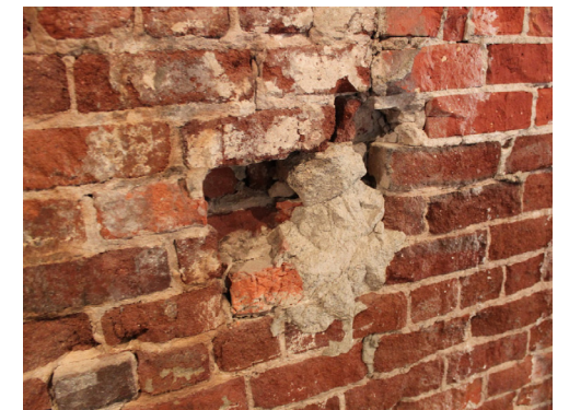
Missing bricks, hole shows double-width
