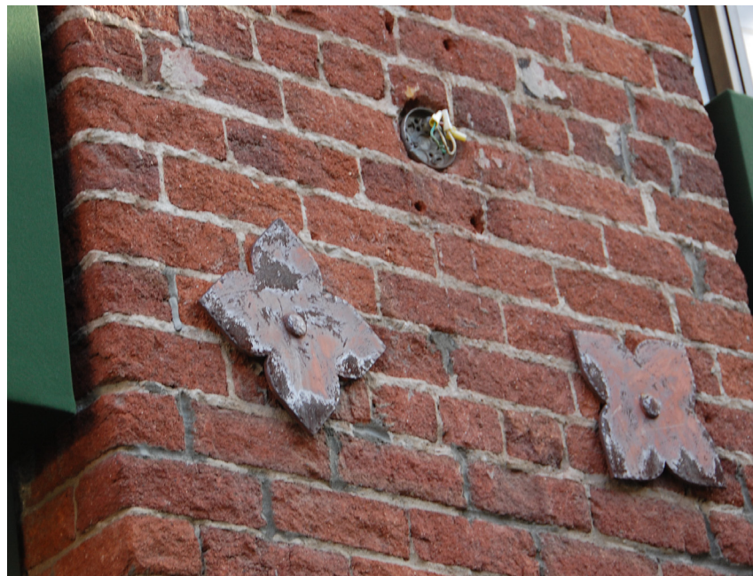
seismic ties to be repaired / painted, abandoned electrical boxes to be removed and patched
