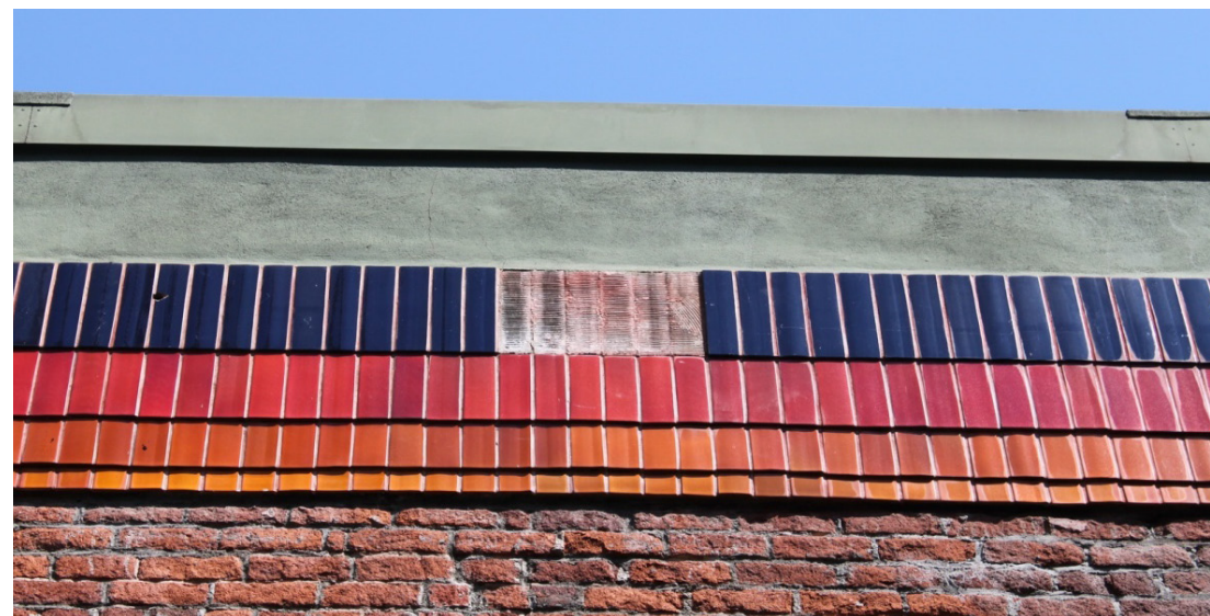
Non-historic ceramic tile/cement plaster parapet to be removed and replaced with brick to match existing. See elevation on page 25 for proposed design.
