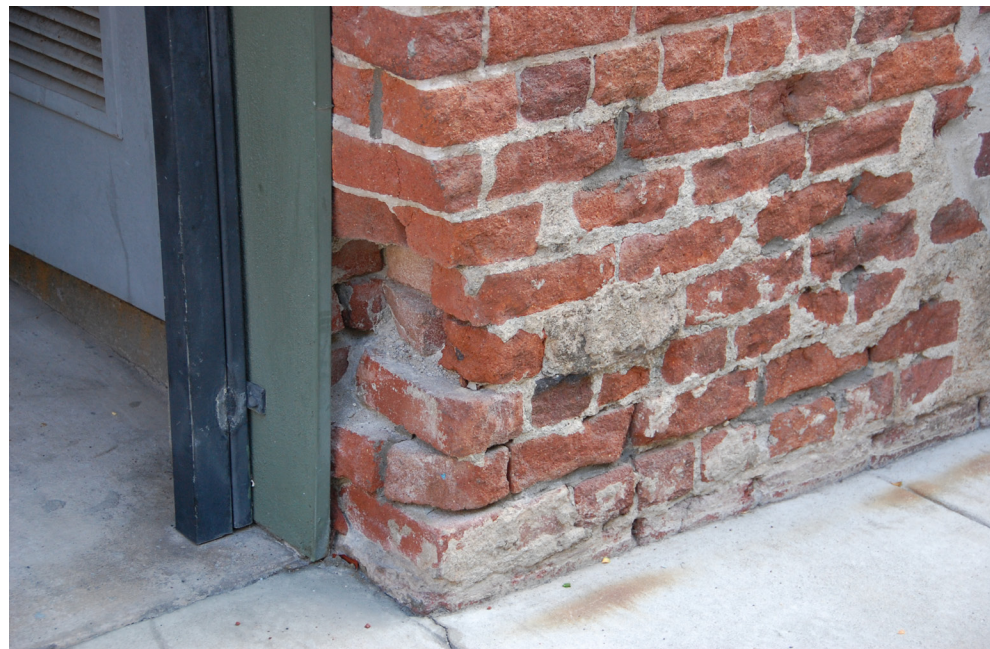
damaged bricks to be replaced
