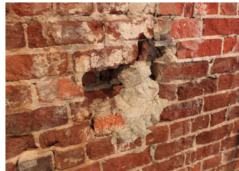
missing bricks to be replaced
