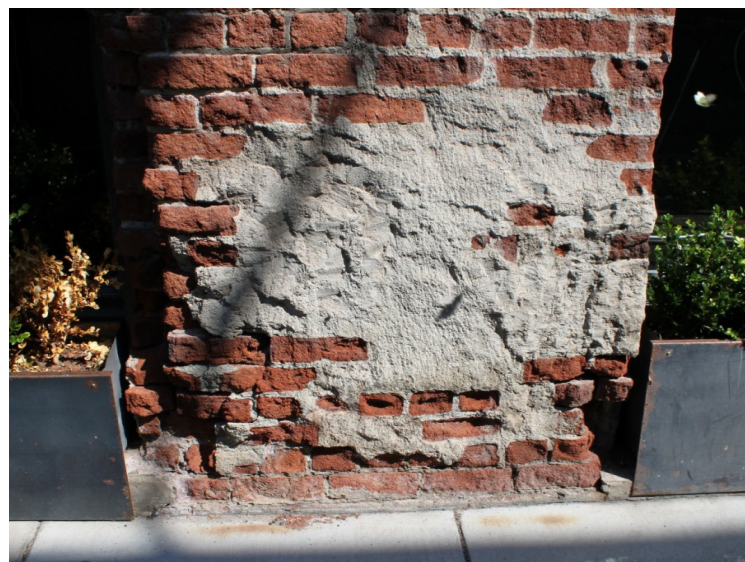
excess mortar and stucco to be removed, missing bricks to be replaced
