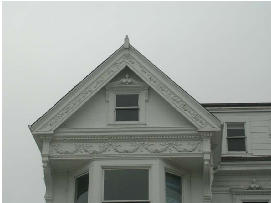
Image 22. The attic window with swan-neck pediment sits within the Queen Anne Style gable supported by an Ionic entablature with decorative festoons at the frieze. Knapp Architects, digital photograph, 2009.
