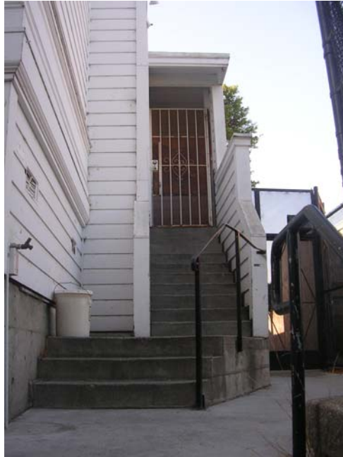
Image 13. South elevation, view of side entryway with stair and yard gate at right. Knapp Architects, digital photograph, 2009.
