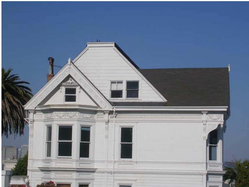
Image 6. West elevation, roof addition for expansion of attic adjacent to original ornamental gable at left. Knapp Architects, digital photograph, 2009.
