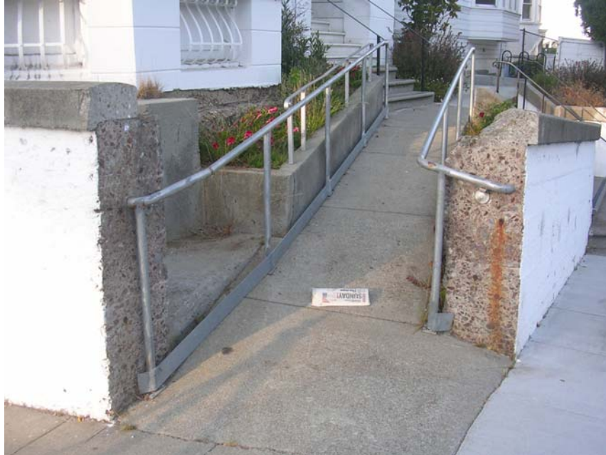
Image 15. Corner of Steiner and Grove Streets, view of original retaining wall that was cut to install a ramp along the south side of building. Knapp Architects, digital photograph, 2009.
