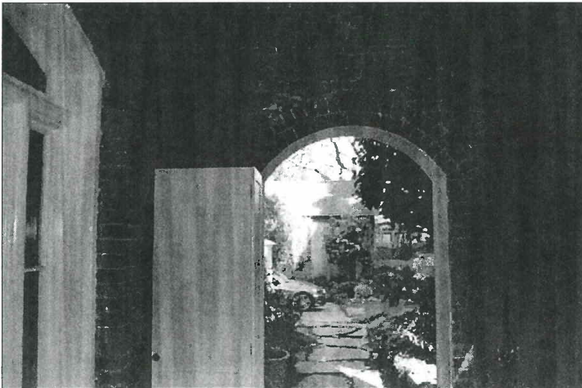
Photo 20. Burr House, 1772 Vallejo Street, 94123. Condition of URM underneath porch shows mortar has suffered from some water damage.
