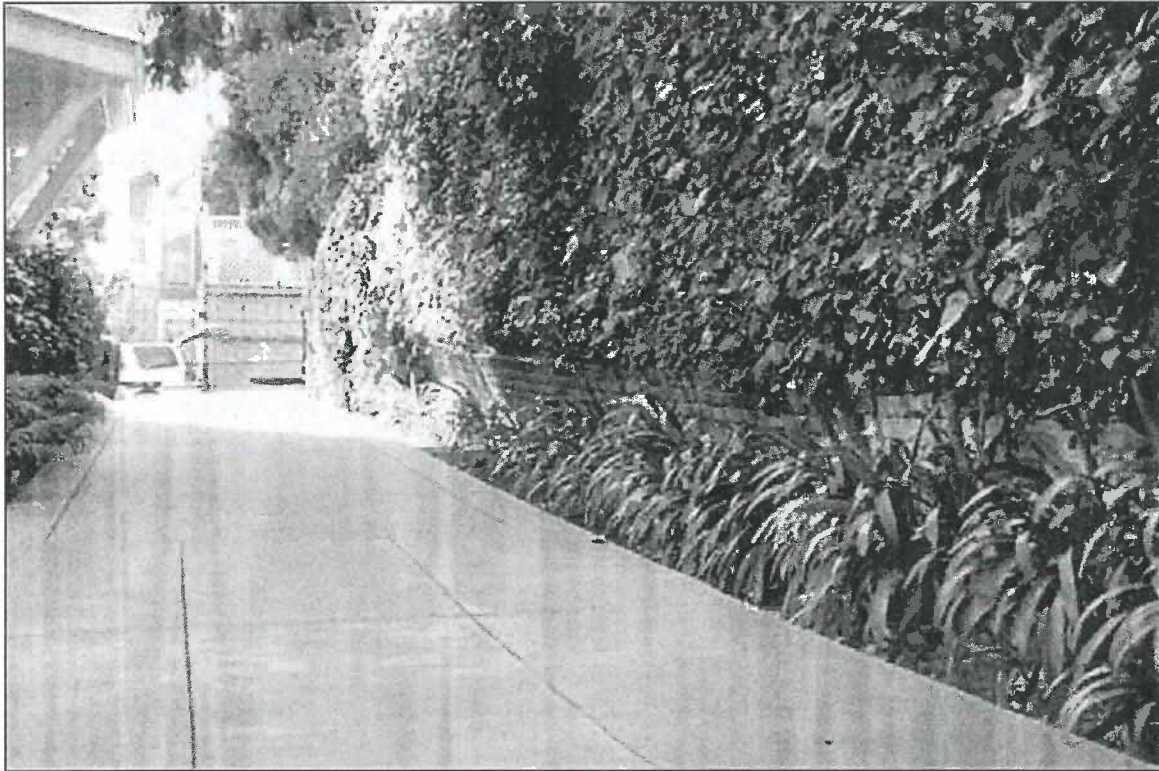
Photo 22. Burr House, 1772 Vallejo Street, 94123. Out of plane URM brick wall west of driveway.
