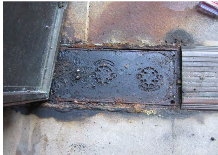
Corroded floor closer at Bronze Doors
