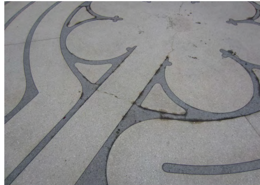
Existing Labyrinth Note: terrazzo cracking
