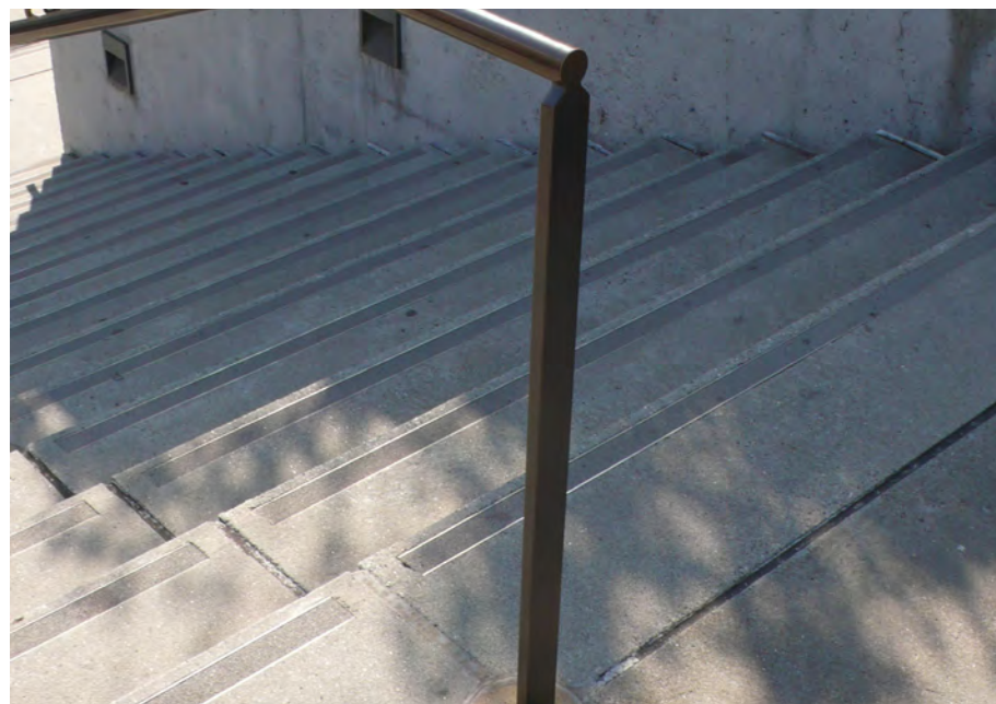
Existing Handrails at the concrete steps from 1995
