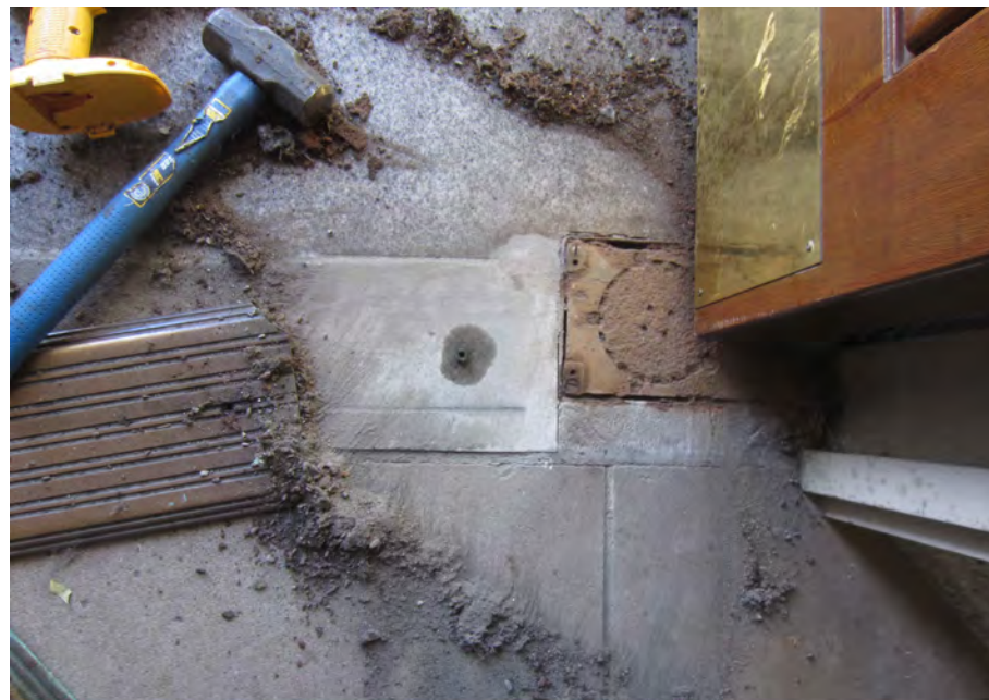
Corroded floor closer at Wood Doors
