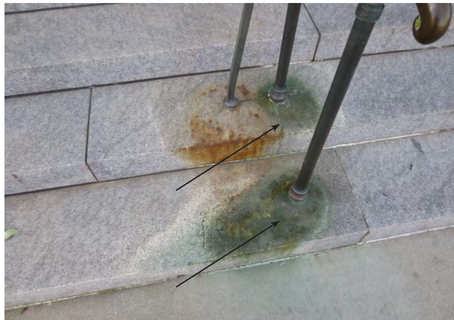
Existing Stone Steps Note: staining and cracking at handrails
