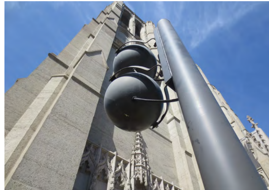
Existing south light fixture
