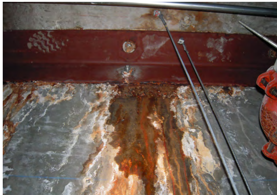
Water intrusion at Crypt Level
