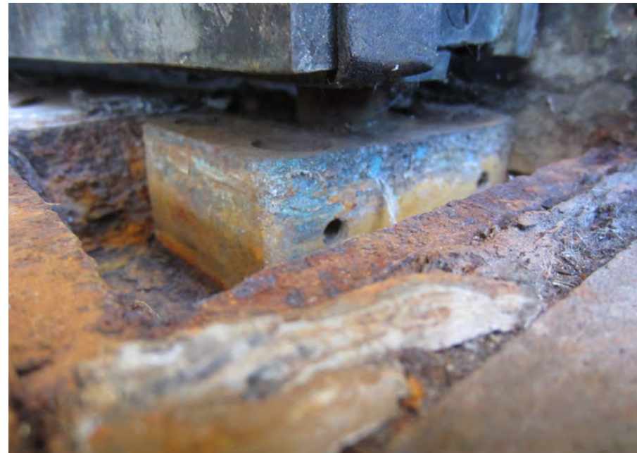
Corroded bronze pivot at Ghiberti Doors
