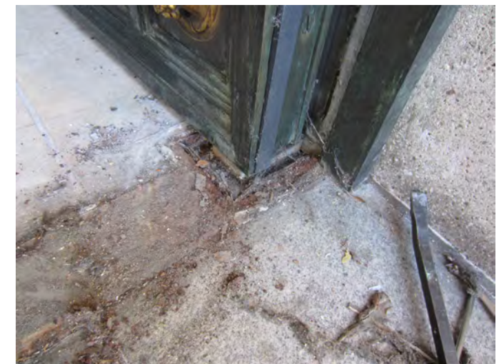
Ghiberti Door Pivot to be replaced
