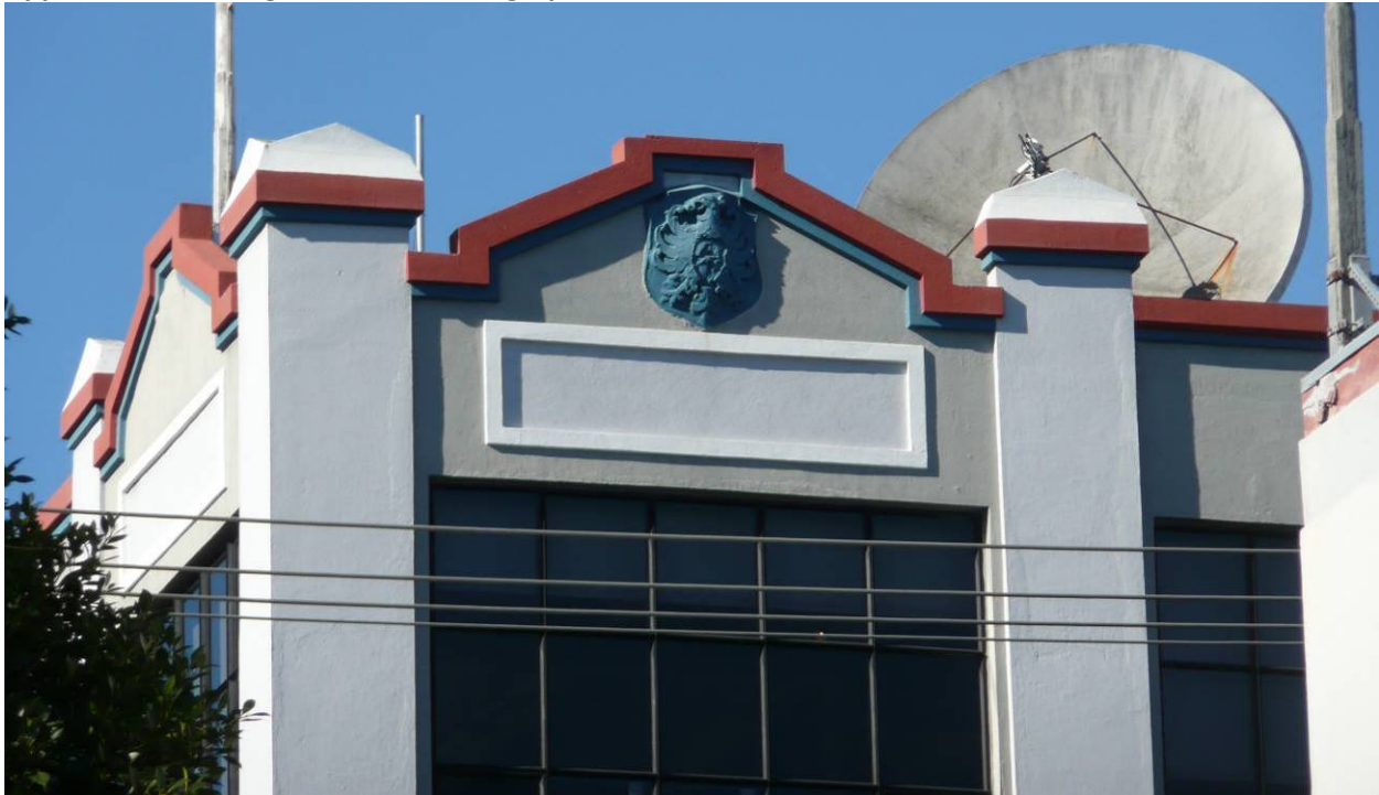
Figure A3. Detail of southeast corner of parapet, looking west (Architectural Resources Group, January 2013). Note the similarity between the heraldic eagle ornamentation and that shown below in Figure B4.
