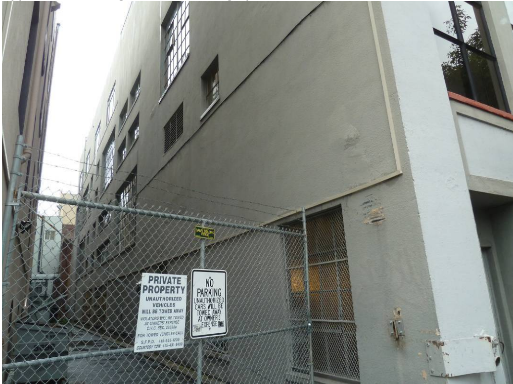
Figure A10. View of private alley along west elevation (Architectural Resources Group, January 2013).
