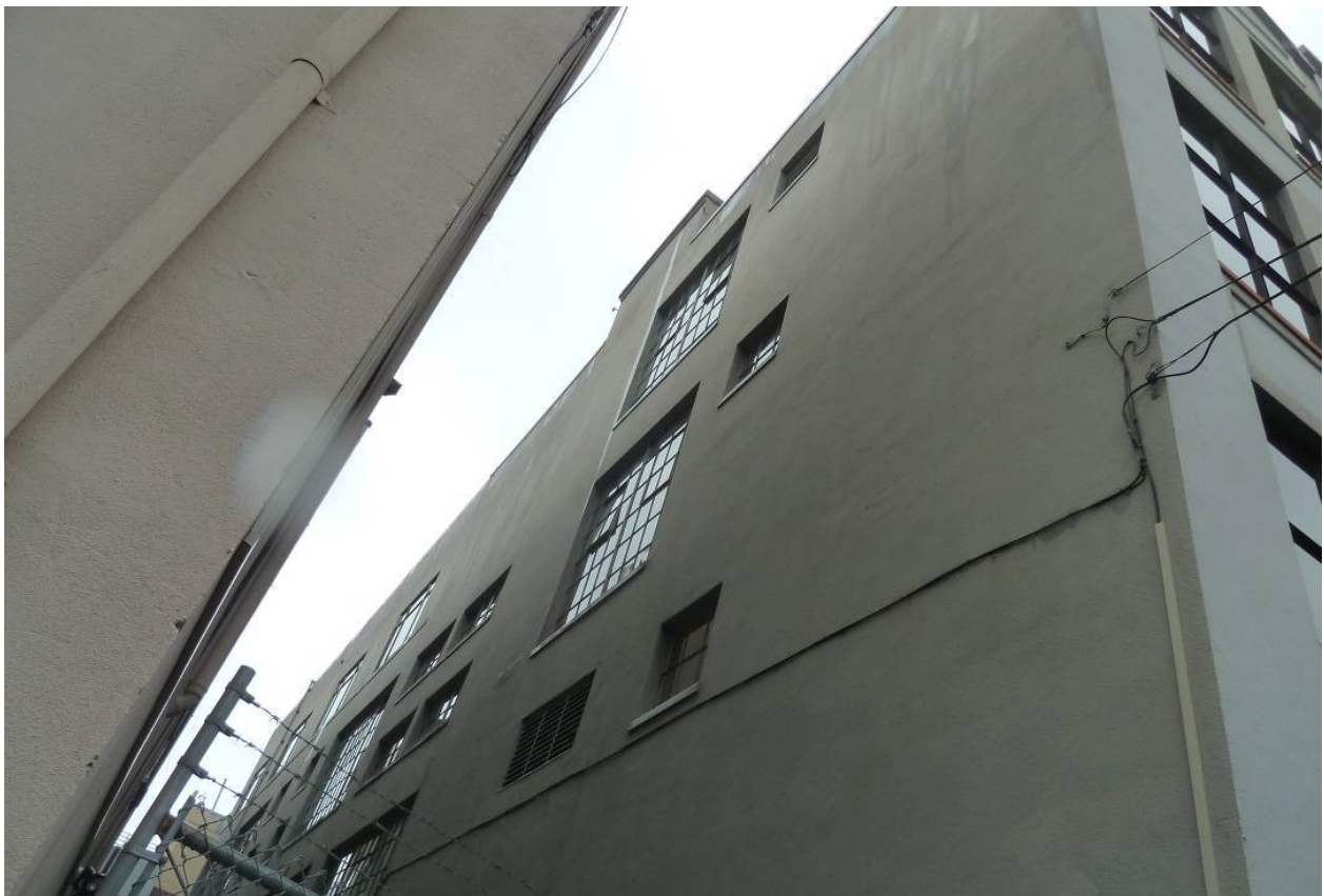
Figure 4. View of west elevation, where new exterior shearwall is proposed (Architectural Resources Group, January 2013).
