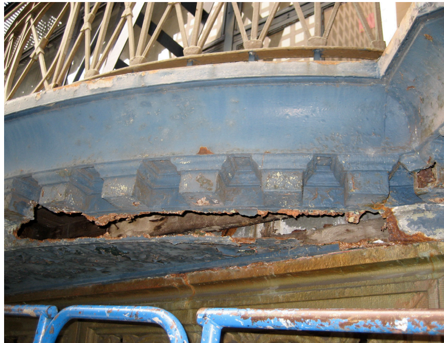
Balcony cornice prior to repairs
