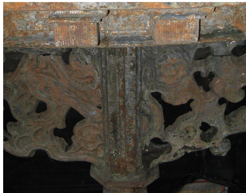
Frieze panel prior to repairs
