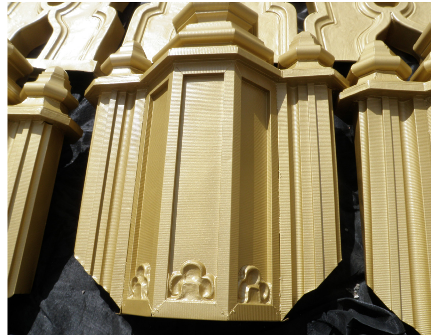
Repaired pendant prior to installation
