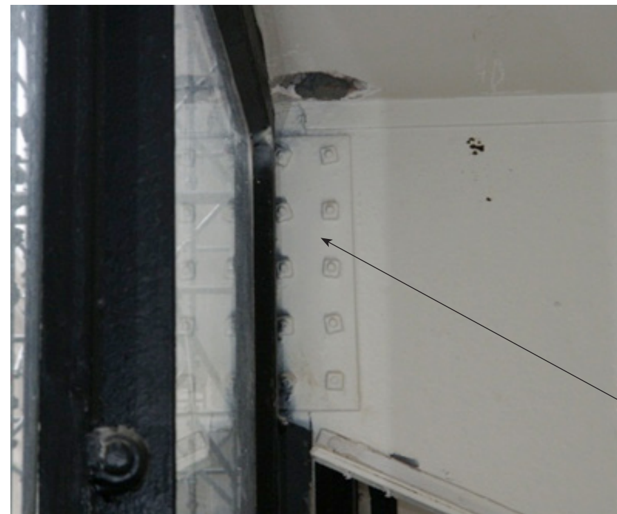
existing bolt plates connect T-mullion to outrigger plates; additional outriggers and bolt plates will match existing design
