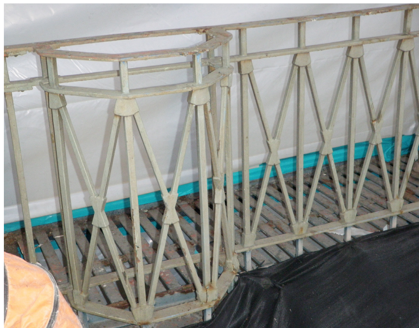
Railings prior to repairs
