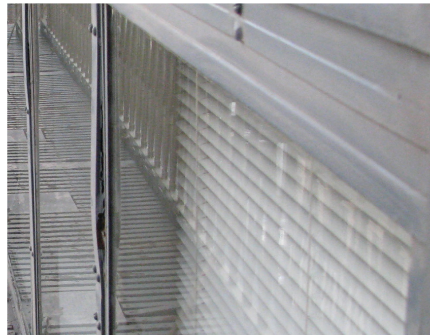
Close-up view of area where vertical plate has separated from windows
