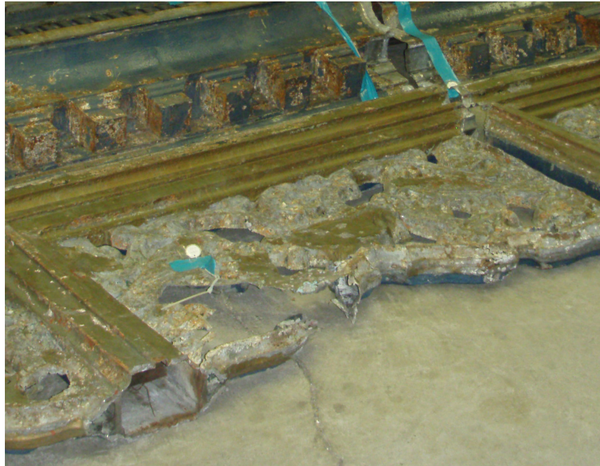
Frieze panel prior to repairs
