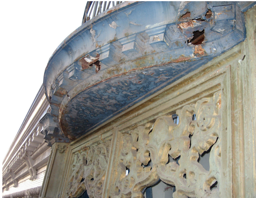
Balcony cornice prior to repairs
