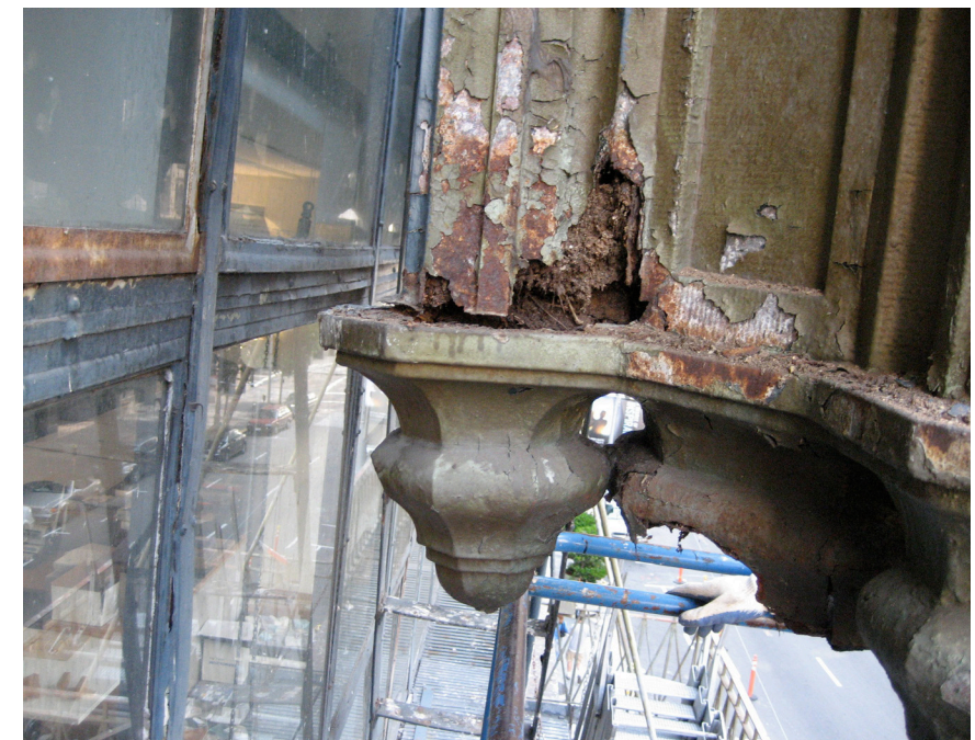
Large pendant prior to repairs
