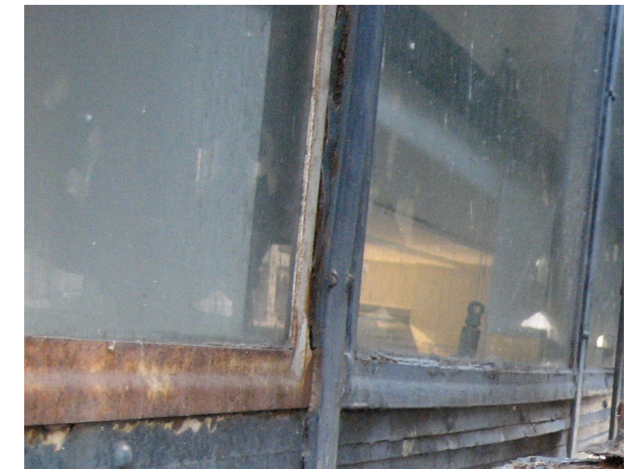
Rust at windows
