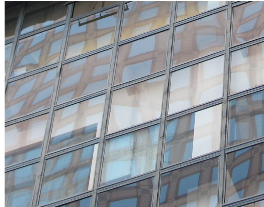
Close-up view of facade showing areas where vertical plate is warped
