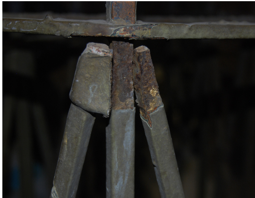
Deteriorated railing bracket ("bow ties")
