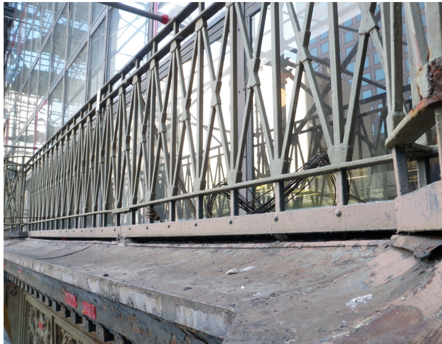
Railings prior to repairs
