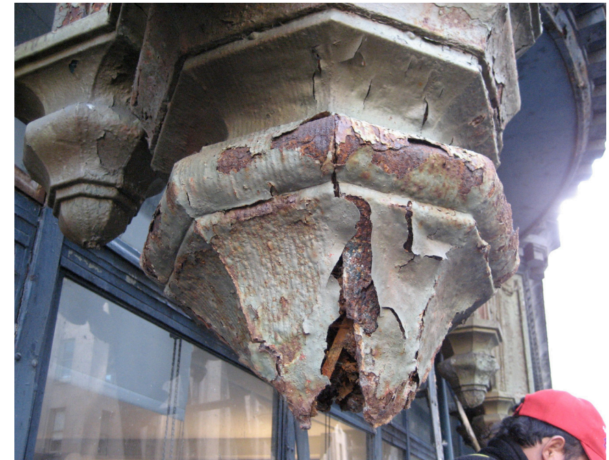
Large pendant prior to repairs
