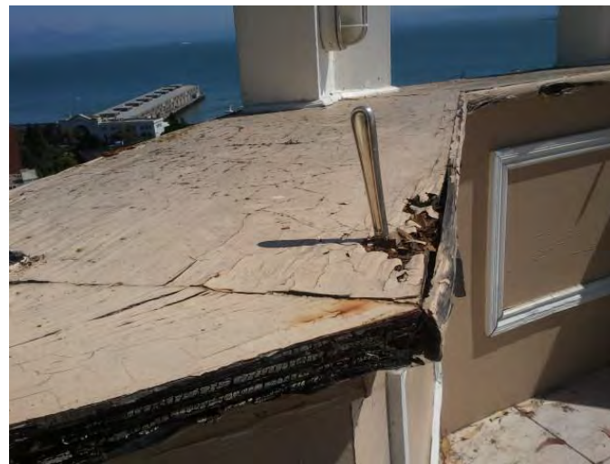
Figure 23 - Dry Rot and Cracking of parapet
