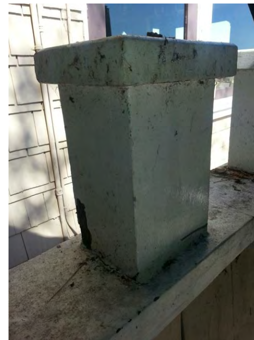
Figure 26 - Existing crenellation with dry rot
