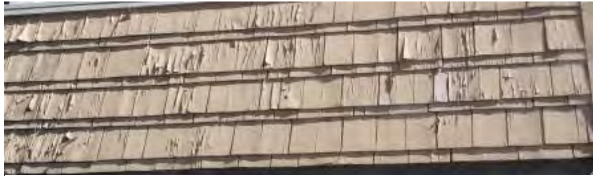
Figure 22 – Example of Shingles on South Side Requiring Repair/Repainting
