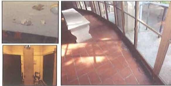
Top left: Flaking paint and blisters on ceiling; Bottom left: Restrooms; Right: Floor tiles at the first floor gallery
