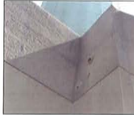
Concrete spalling at the northwest tower base
