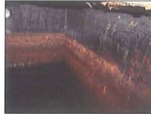
Interior of tank, showing low water level and corrosion
