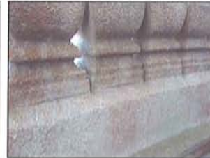
Detail of cracking at Belvedere Level balustrade
