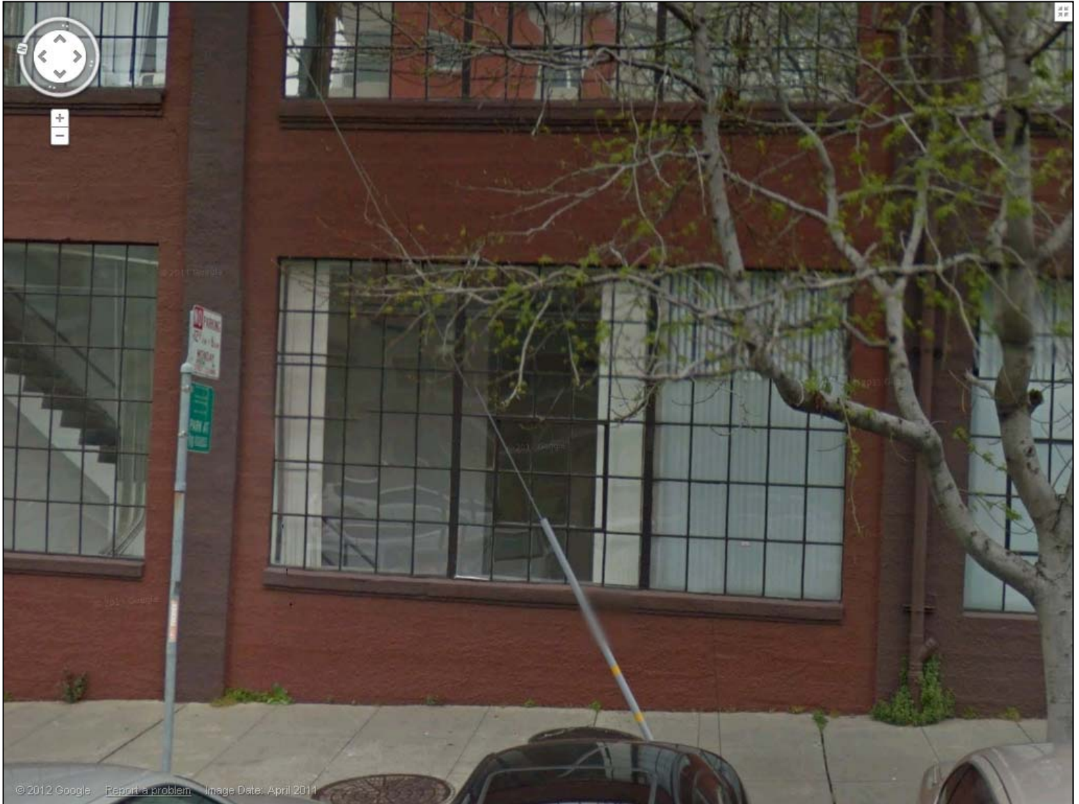
444 De Haro Street, View of original steel-sash windows on Rhode Island Street
