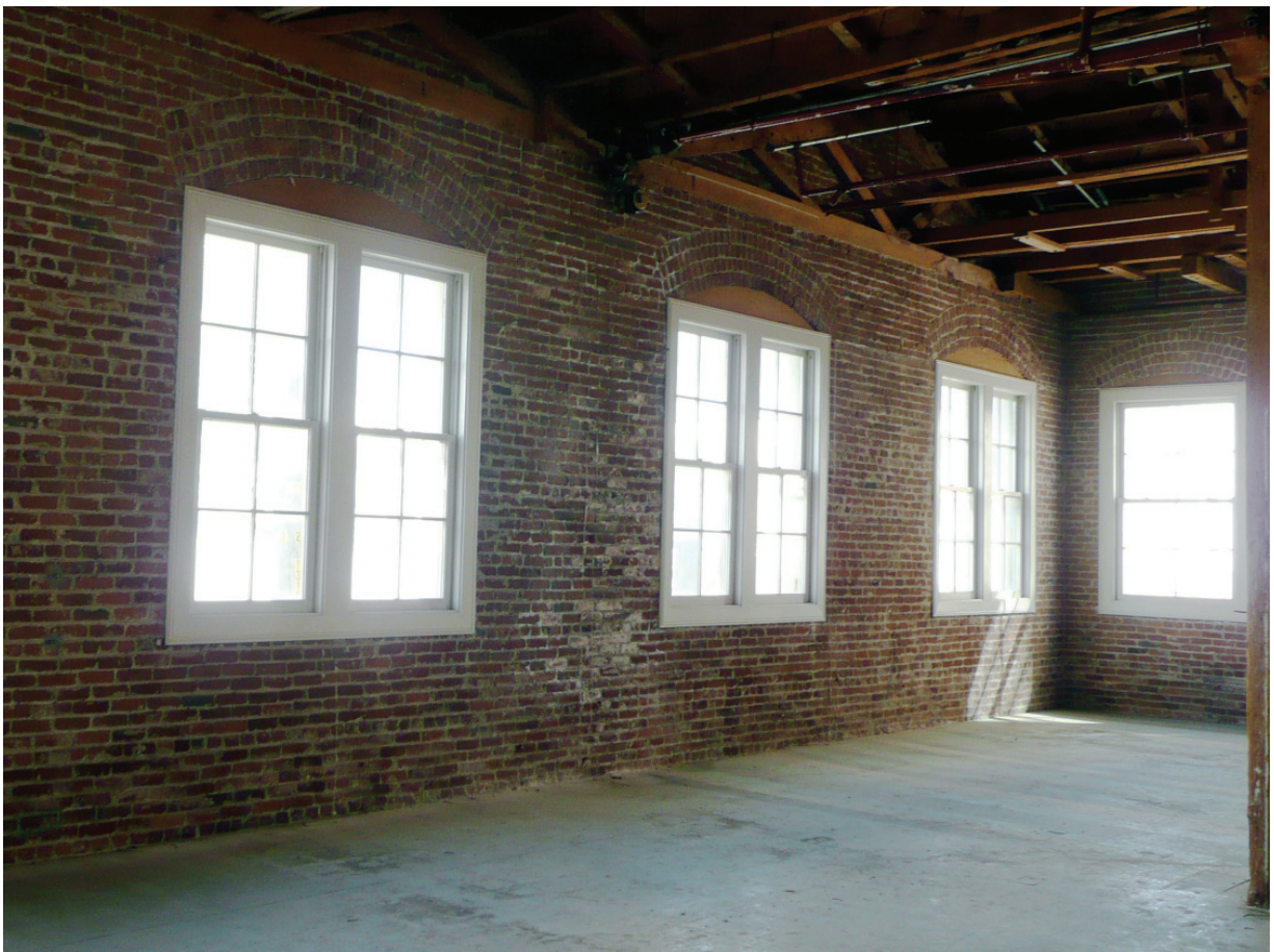
Figure A12. View of third floor interior, looking northeast (Architectural Resources Group, October 2011).
