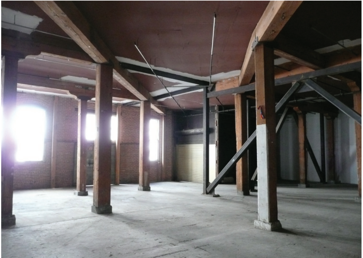
Figure A9. View of first floor interior, looking southeast. Note the diagonal beams along the former path of rail into the structure (Architectural Resources Group, October 2011).
