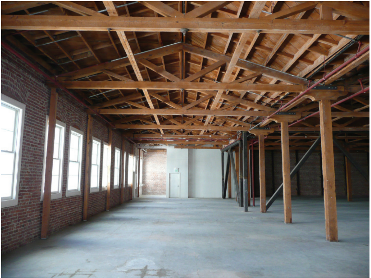
Figure A13. View of third floor interior, looking south (Architectural Resources Group, October 2011).
