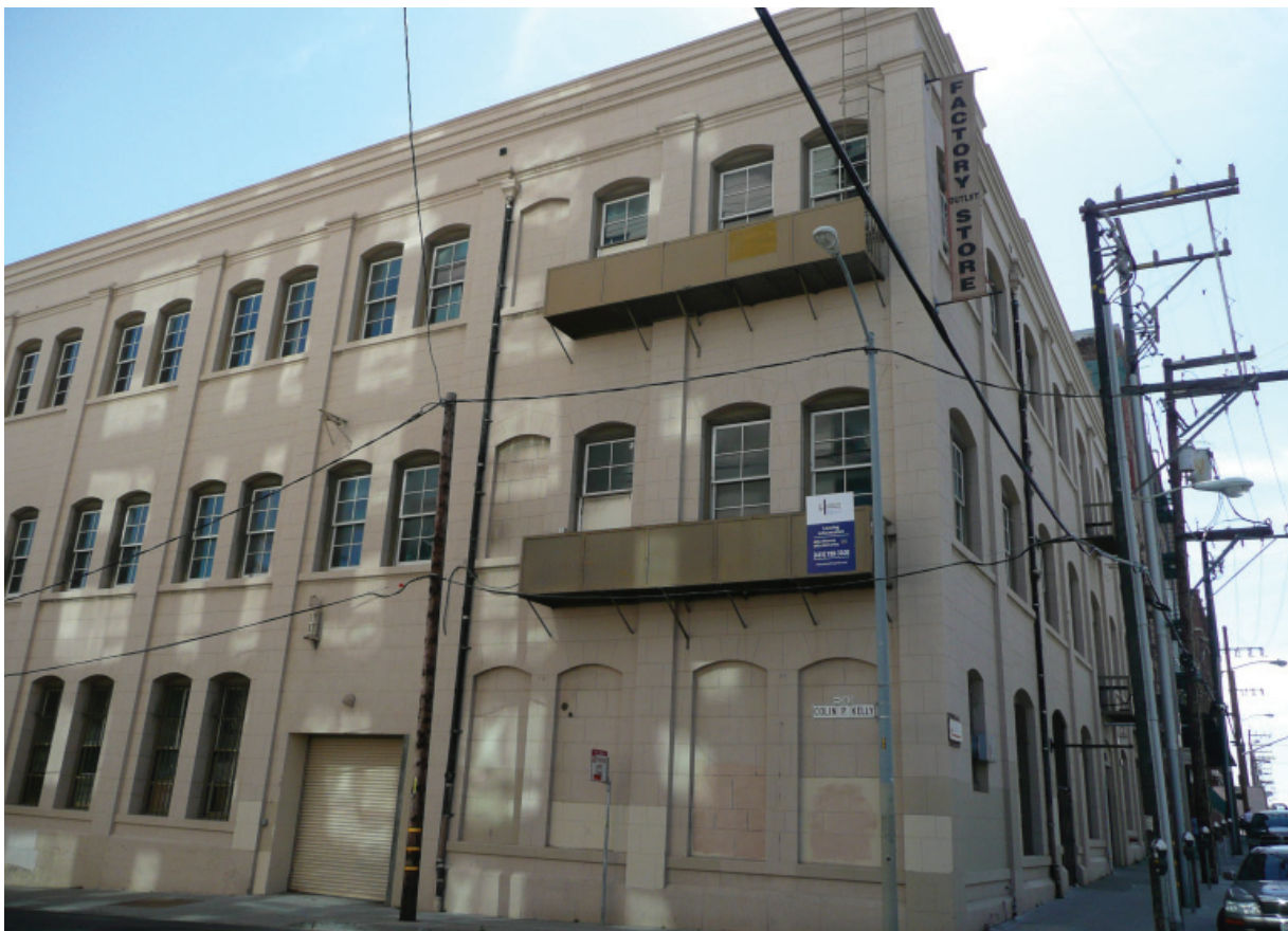
Figure A6. These window openings on the Colin P. Kelly Street side were filled-in originally or soon after the building's construction (Architectural Resources Group, October 2011).
