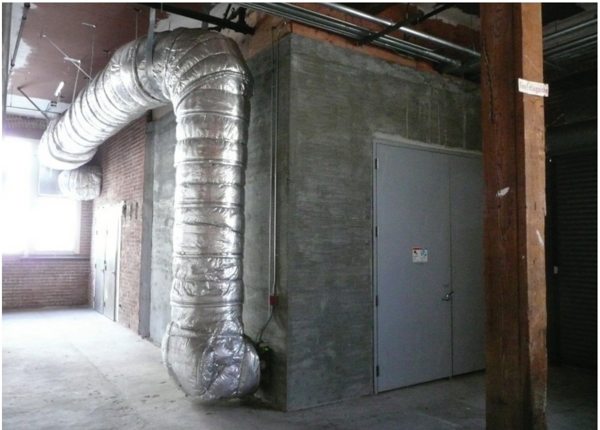
Figure A10. View of partition walls enclosing the utility transformer and switchgear at the building's northeast corner (Architectural Resources Group, October 2011).
