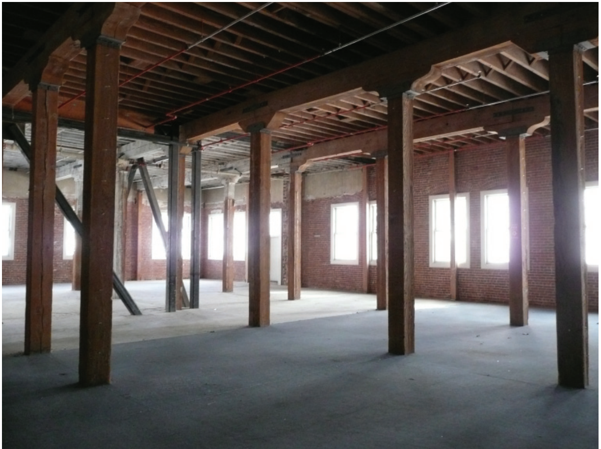
Figure A11. View of second floor interior, looking northeast (Architectural Resources Group, October 2011).
