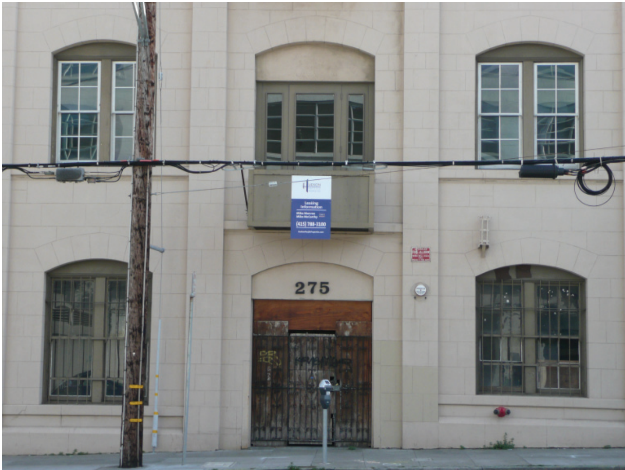
Figure A3. Detail of middle three bays along main façade (Architectural Resources Group, October 2011).
