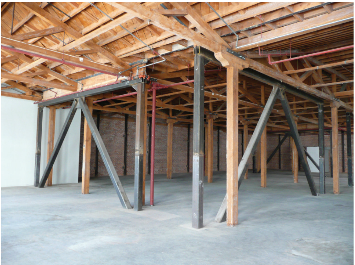
Figure A14. Partial view of seismic bracing at third floor (Architectural Resources Group, October 2011).
