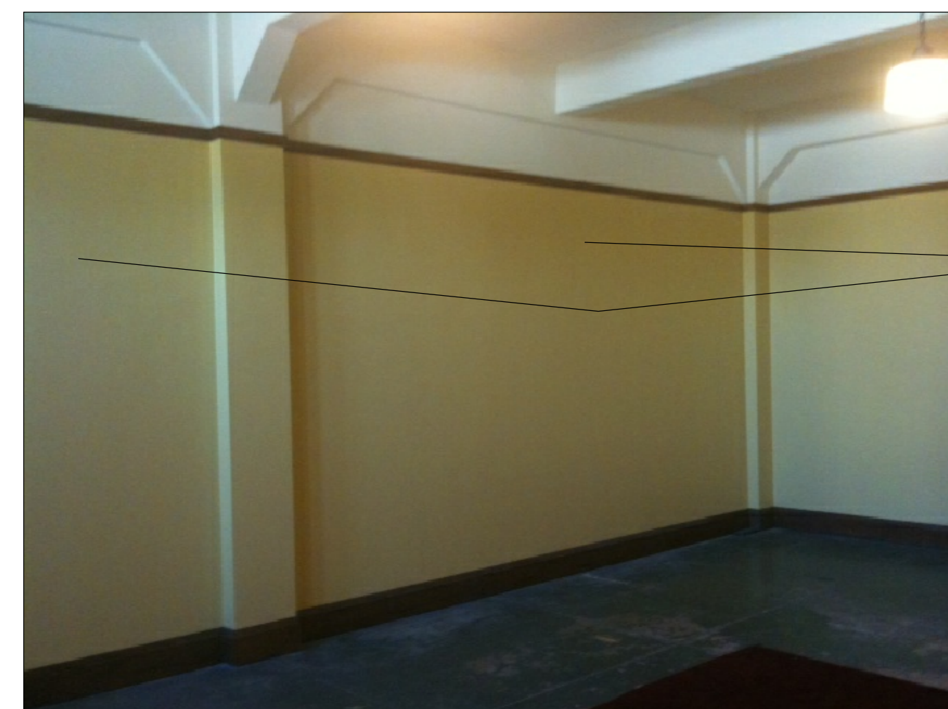
INTERIOR OF FORT - THIRD FLOOR TYPICAL INTERIOR WALLS TO BE REMOVED BETWEEN COLUMNS
