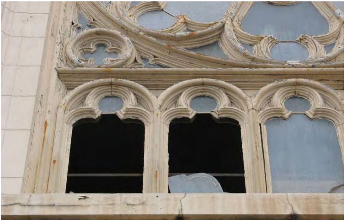
Figure 7c. West transept rose window, showing paint loss and missing glazing.
