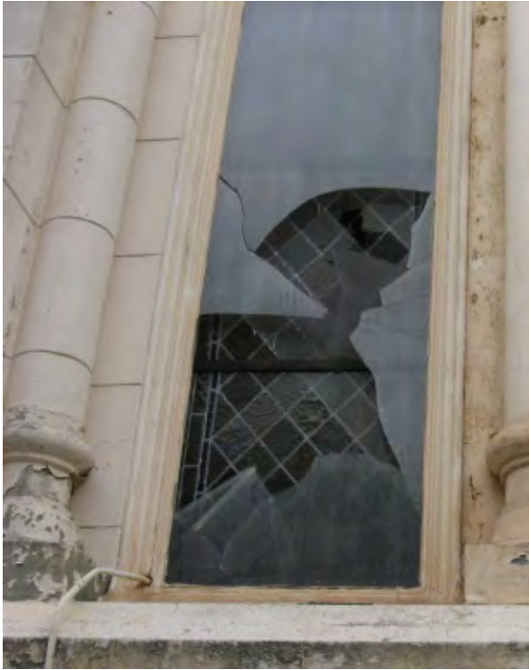
Figure 7a. West tower, north window, showing broken protective glazing.
