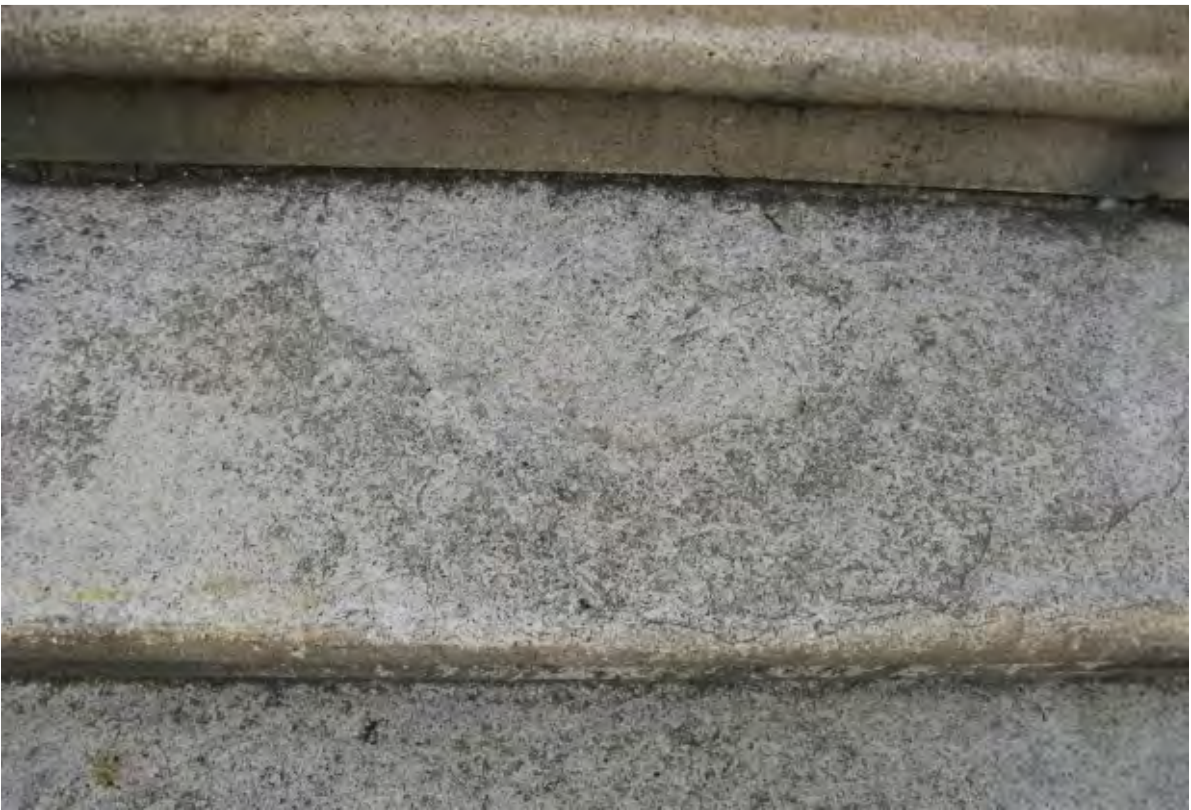
Figure 2e. Detail, south portal steps, spalled surface of granite tread.
