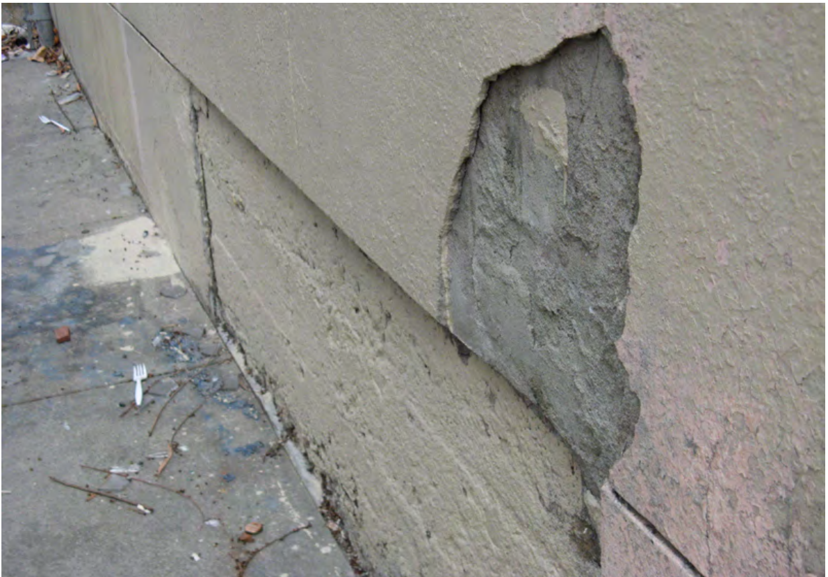
Figure 3b. East tower, north façade, showing loss of stucco at ground level.
