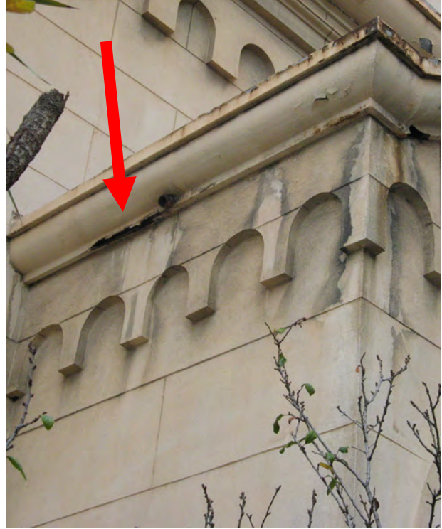
Figure 6b. Cornice above north portal, east transept, showing perforation (arrow) of the metal due to corrosion.
