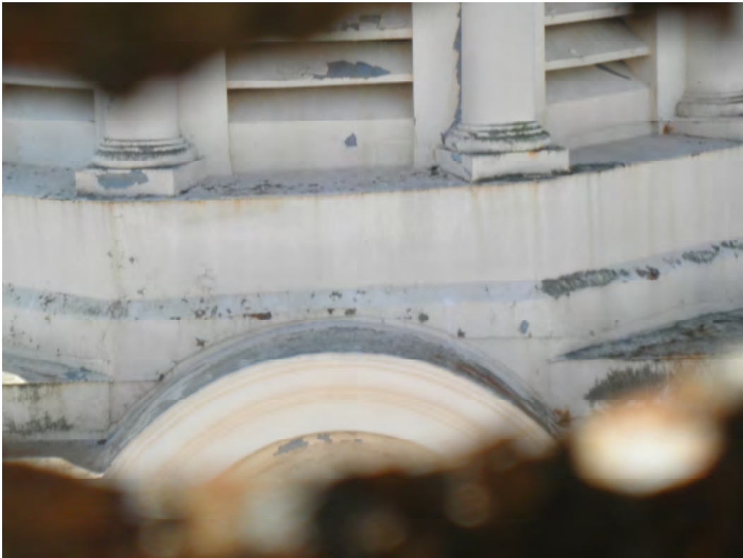
Figure 5a. Detail, rust-through at painted sheet metal cupolas.
