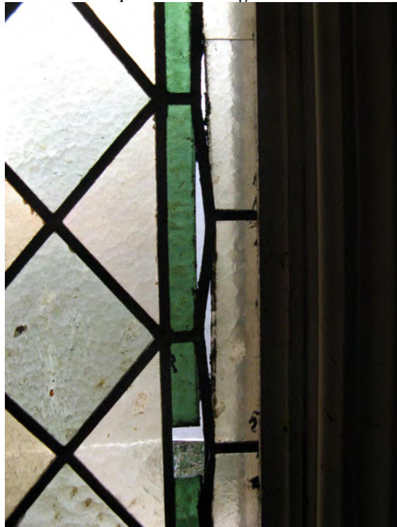
Figure 11c. Breakage and loss of colored glass panes due to distortion of lead cames.
