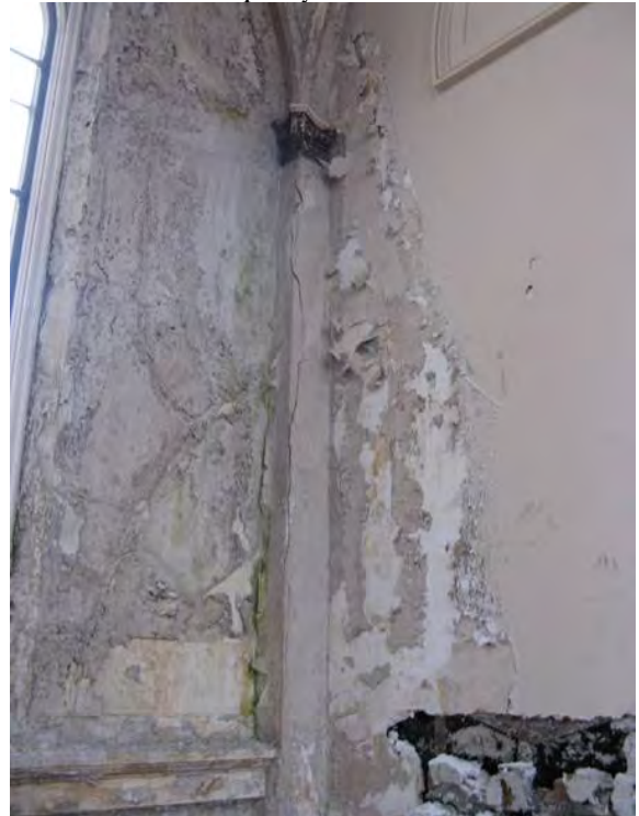
Figure 9d. Structural cracking and separation of plaster details from masonry substrate caused by moisture from blocked drains.
