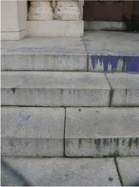
Figure 2a. Main portal steps, showing soiling, paint stains and vertical joints without mortar.
