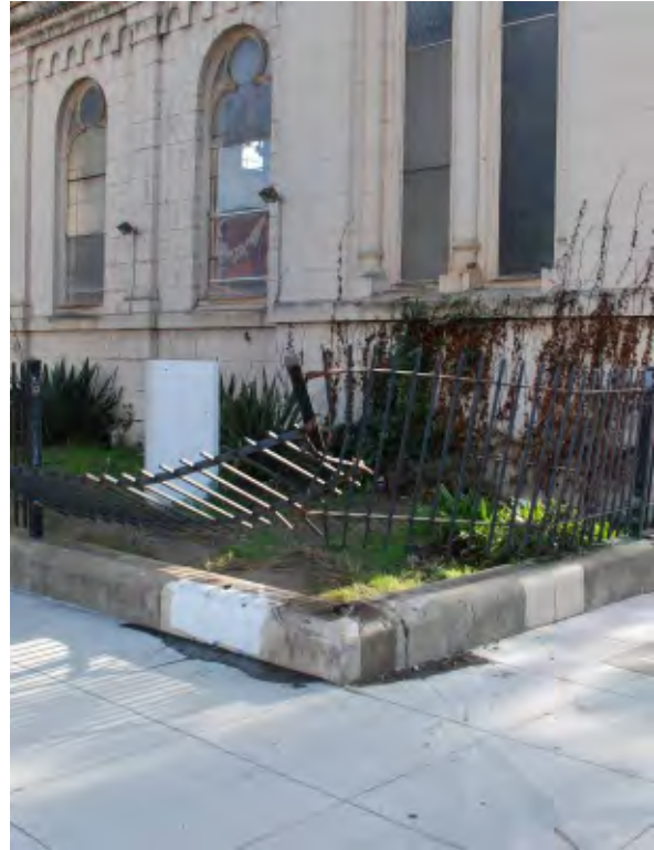
Figure 1b. Damage to metal fence at northeast corner of property.
