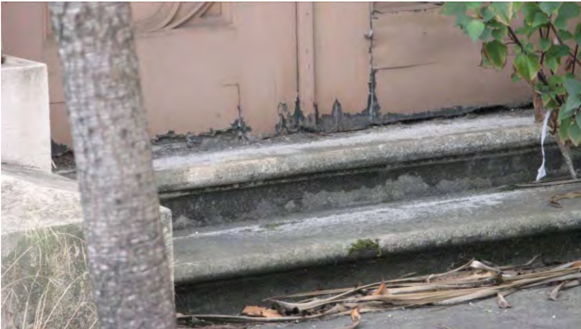
Figure 2c. East transept, north portal steps, showing decorative bull nose with biological growth and soiling.
