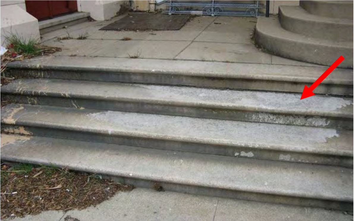
Figure 2d. West transept, south portal steps, showing paint stains (left), soiling and spalling surface (arrow).
