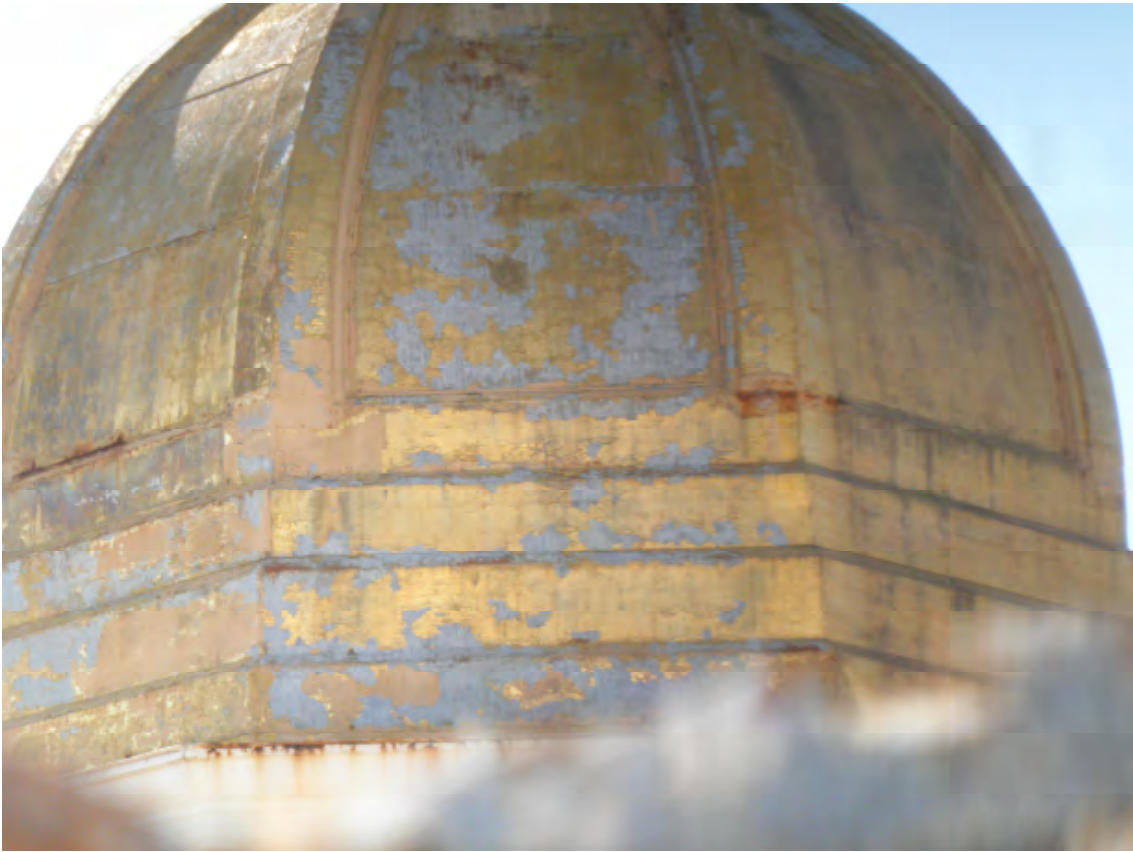
Figure 5c. Detail, corrosion and loss of paint and gilding at domes.
