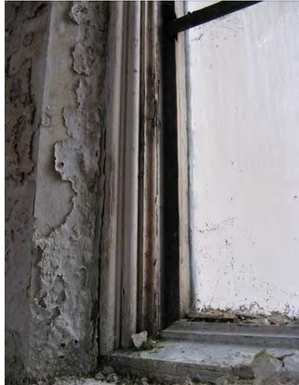
Figure 9b. Deterioration of plaster caused by moisture from poorly sealed window.
