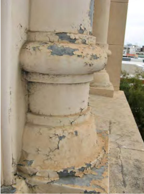
Figure 6a. Column base, south side of east tower, showing flaking and loss of protective paint layer.
