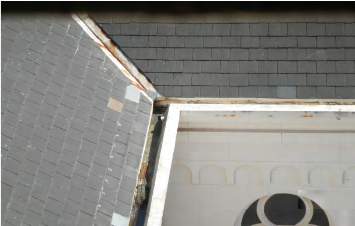
Figure 5d. Broken, loose, and missing slate tiles at main roof.
