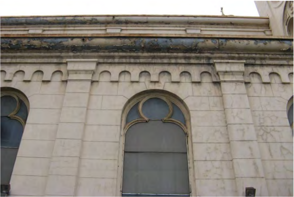
Figure 3a. East nave façade, showing soiling, water staining and hairline cracking of stucco.
