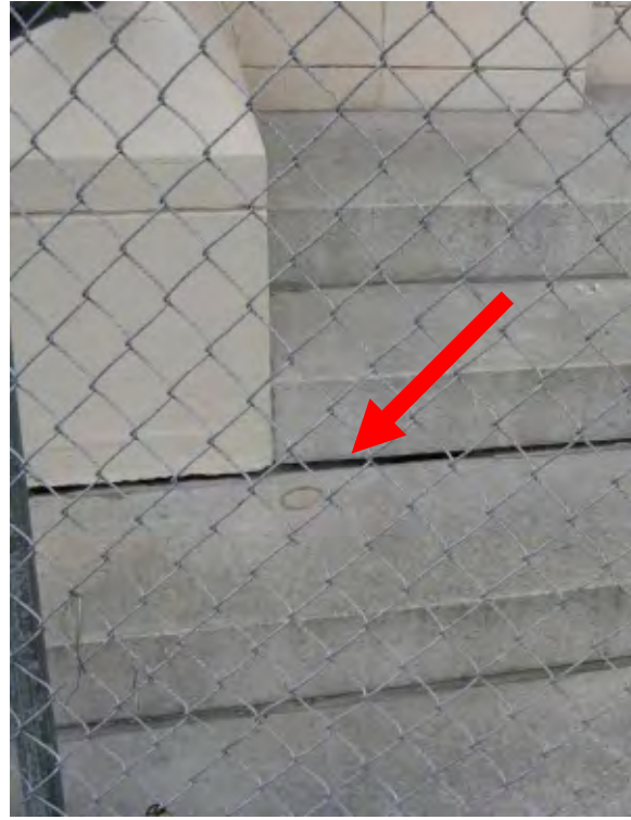
Figure 2b. Detail, east side of main portal steps, showing gap between blocks (arrow) due to uneven settling.
