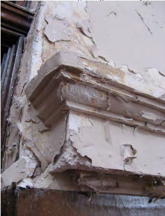
Figure 9c. Softening and deterioration of decorative plaster elements caused by moisture from faulty roofing.
