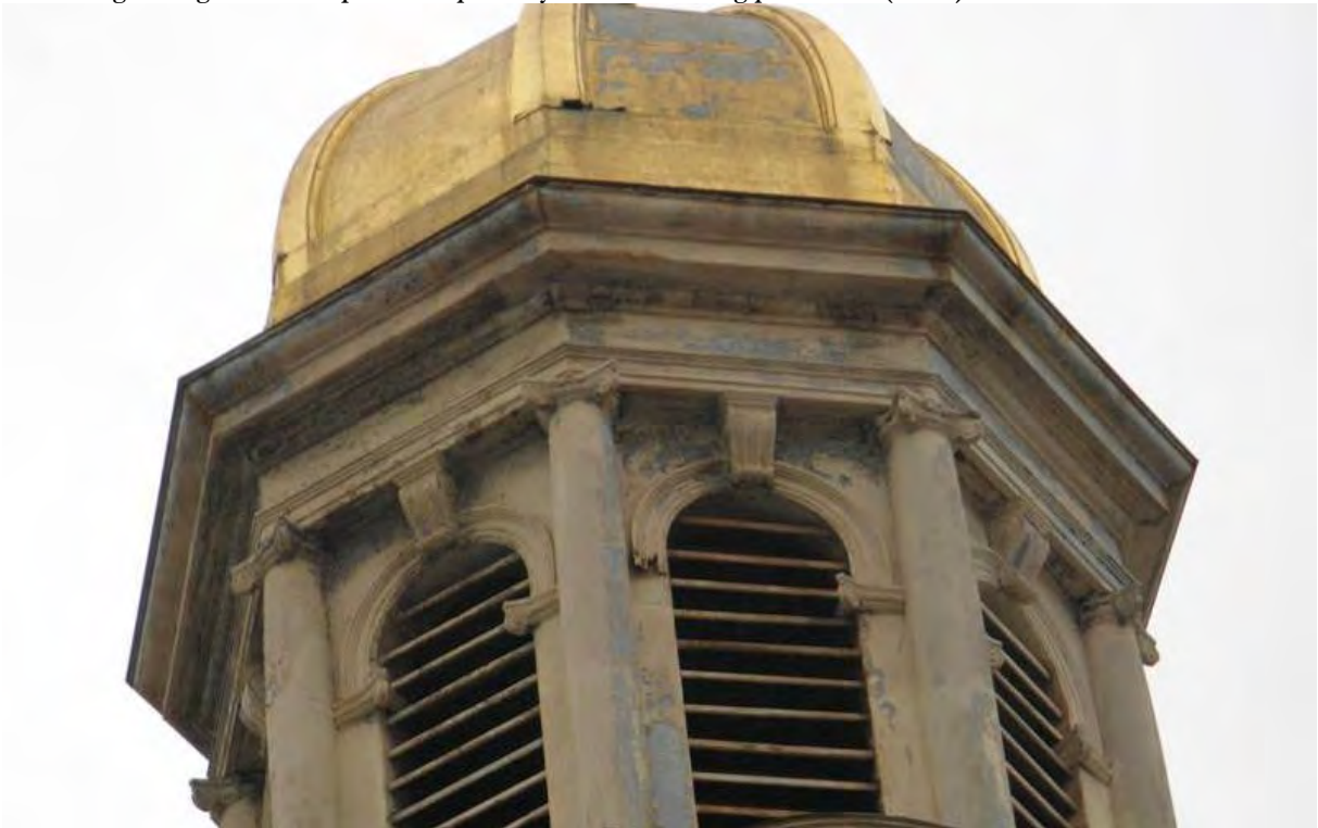
Figure 6c. East tower detail, constructed entirely of pressed sheet metal, showing missing architectural detail, loss of gilding and protective paint, and corrosion stains.
