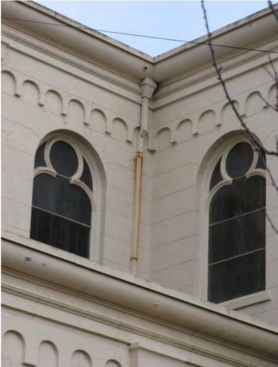
Figure 9a. West façade, showing blocked or perforated drainage which is causing damage to interior plaster.
