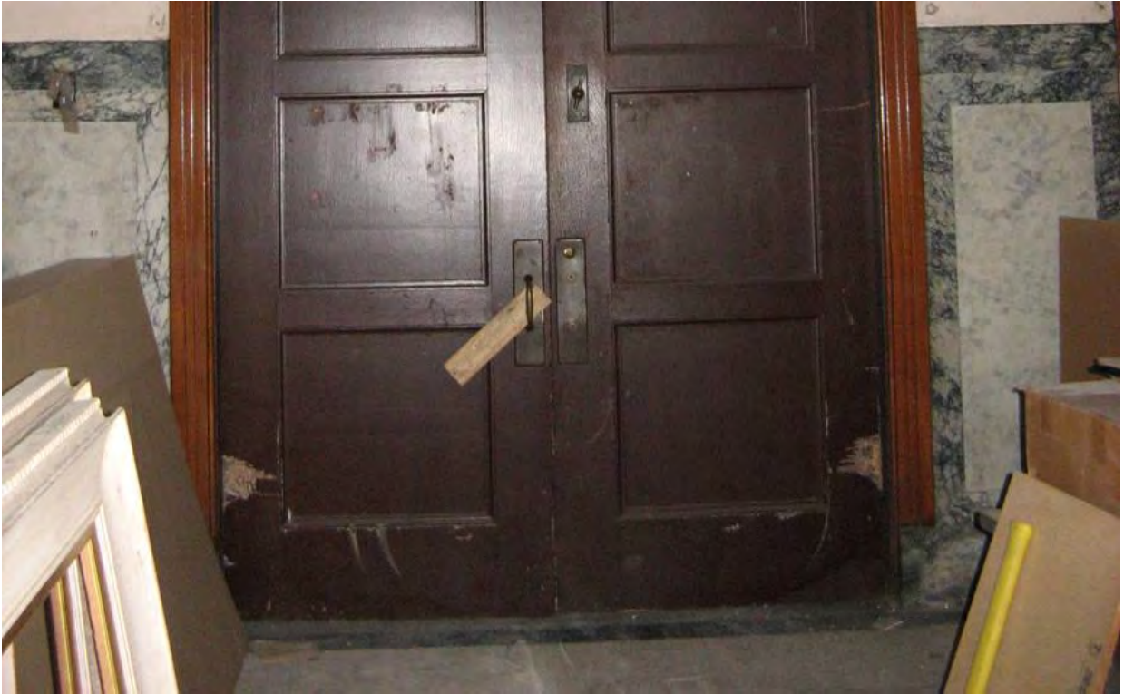
Figure 8a. Marble wainscoting of the narthex, showing soiling of the baseboard, wear of polished surface, and adhered tape.
