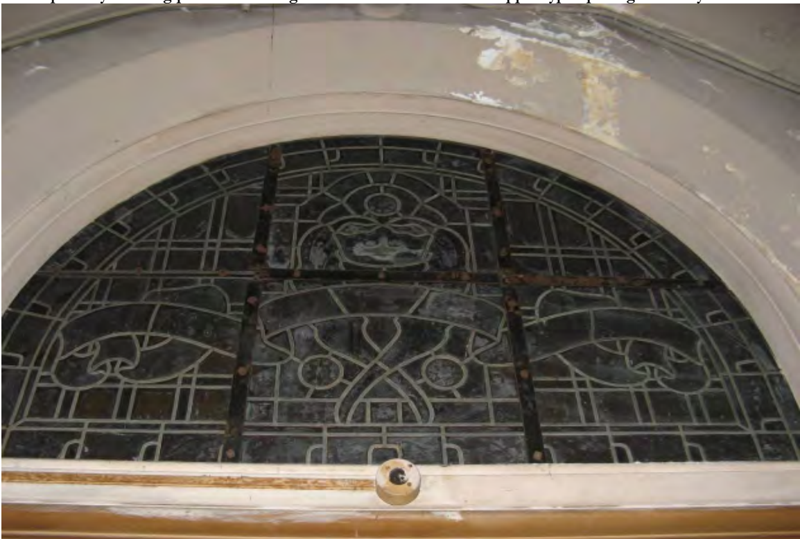
Figure 11a. North-east transept portal, showing blocked figurative stained glass window with heavy soiling and corrosion of steel frame
