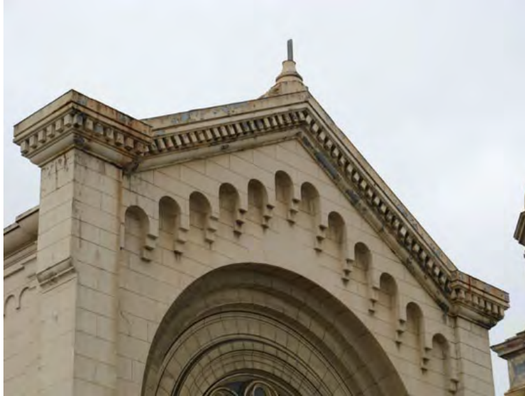
Figure 4. Detail of corbel table and cornice on east transept. Source: Page & Turnbull, November 2007.
