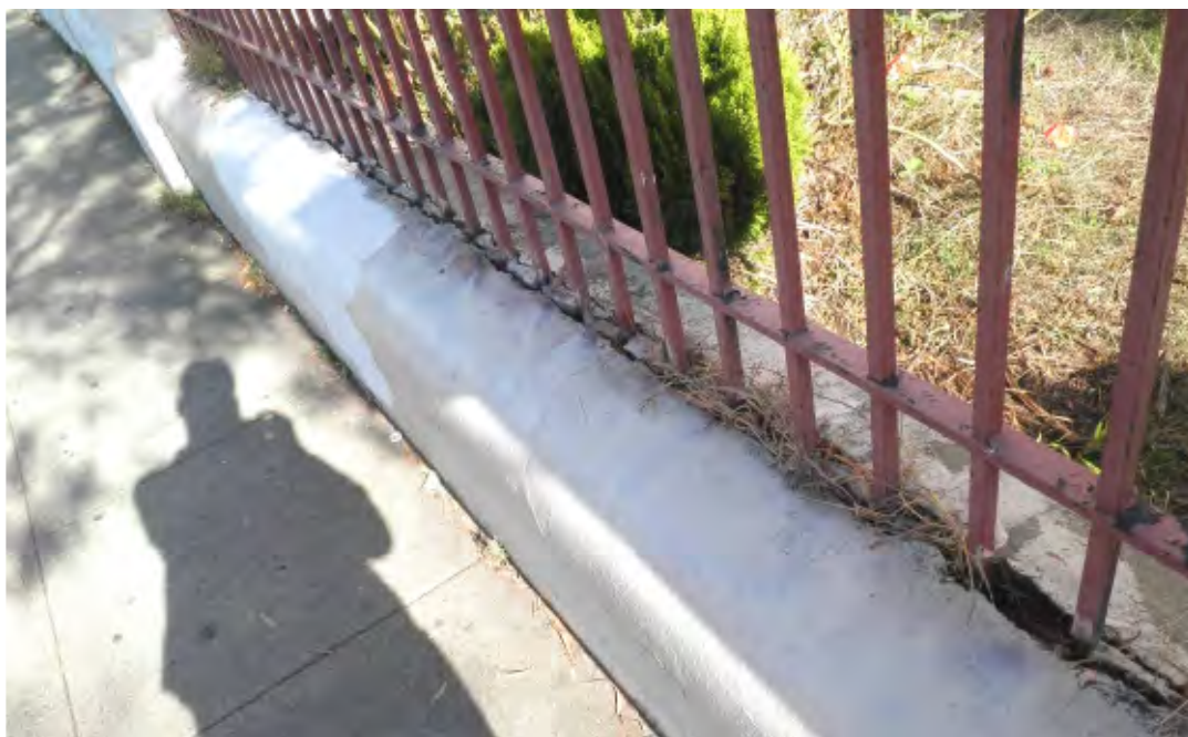
Figure 1c. Low brick wall along Howard Street, showing gaps and voids, corroded metal fence, and graffiti (painted over with mismatched paint).
