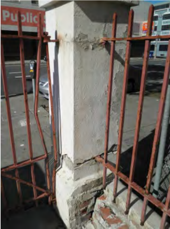
Figure 1a. Pier near west tower, showing large cracks and displaced areas of brick (arrow) and corroded metal fence.
