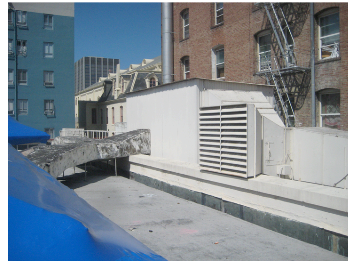
A: View of existing mechanical penthouse to be removed along with ductwork. New north stair penthouse in this location.
