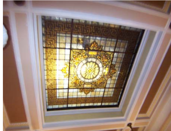
Figure 41. Detail of skylight in Waiting/Reception Room (S-9) located on the second floor south. Source: KVP 2009.
