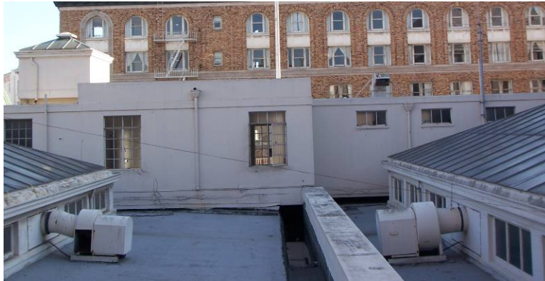
Figure 18. Roof, view south. Note the skylight diffusers at left and right and the penthouse in the background. Source: KVP 2009.
