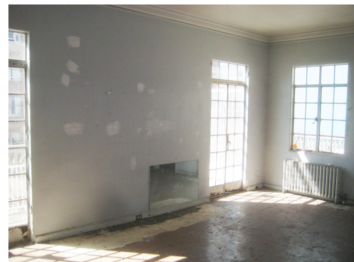
E: View of Penthouse Room to be repaired and renovated. Original steel windows to be replaced with steel single panel French doors.
