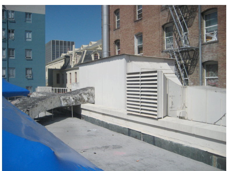
C: Looking northwest at existing mechanical penthouse. Hotel Boyd is at right with fire escape that is over Hibernia property line and uses north exit alley for its exiting.
