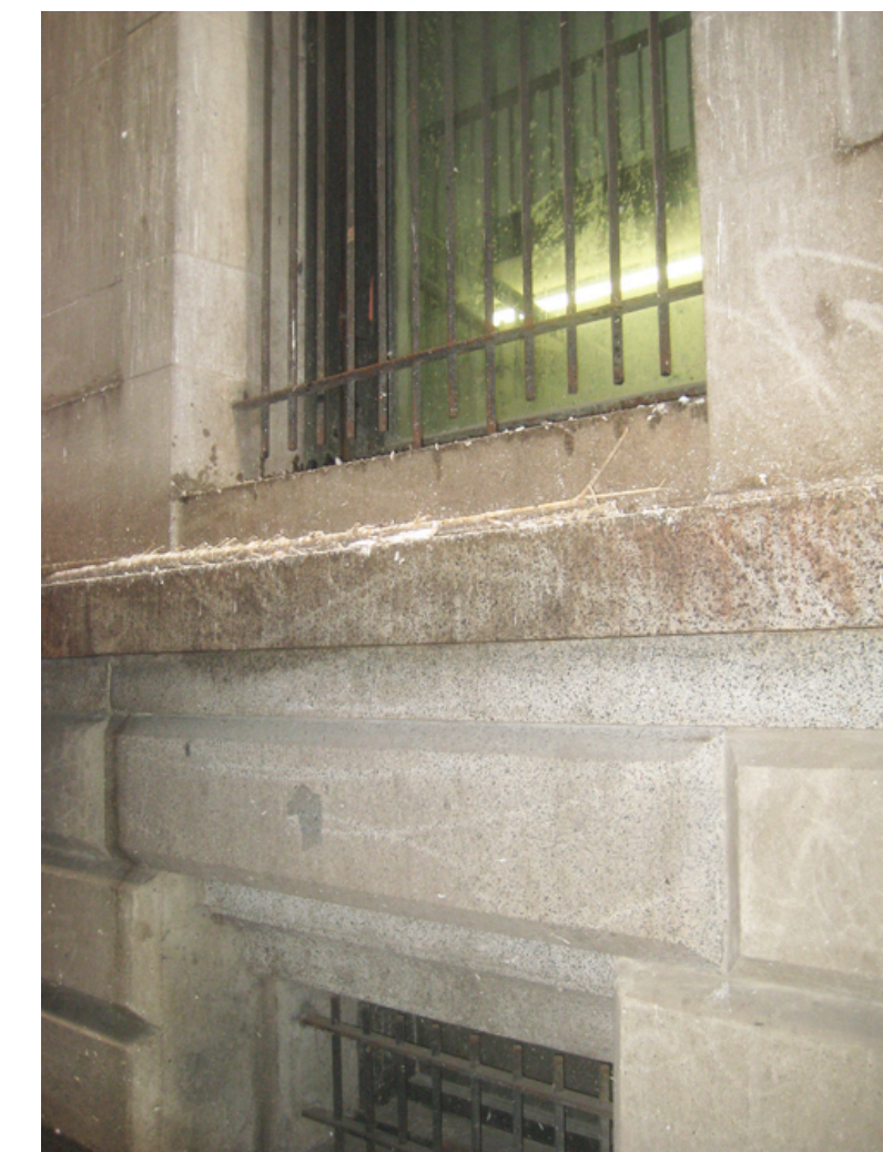
B: View of window to become west exit door from north stair hall
