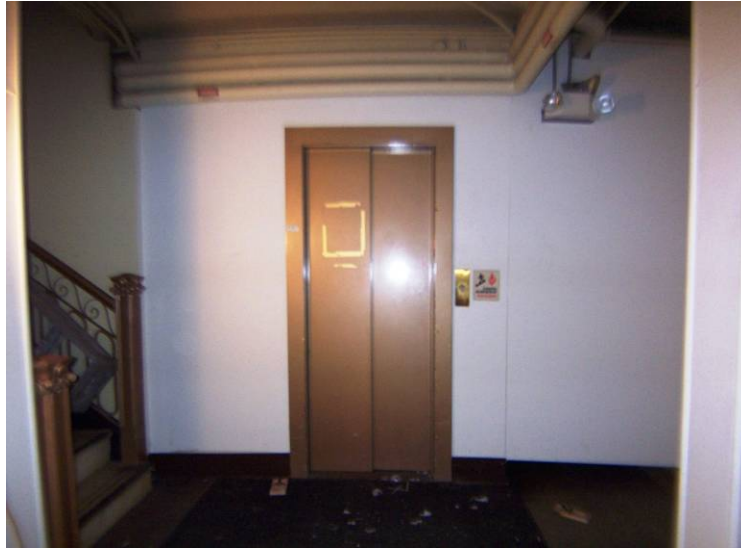
Figure 26. Elevator Lobby and Stairs at left (B-25) located in the basement. Source: KVP 2009.
