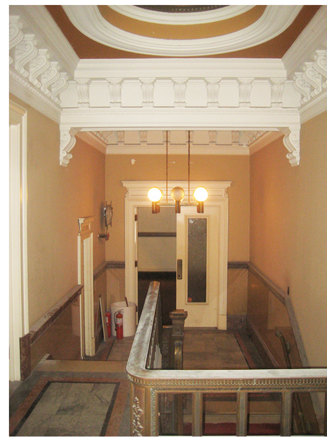
A: View of South stair hall with door to new South stair at left.
