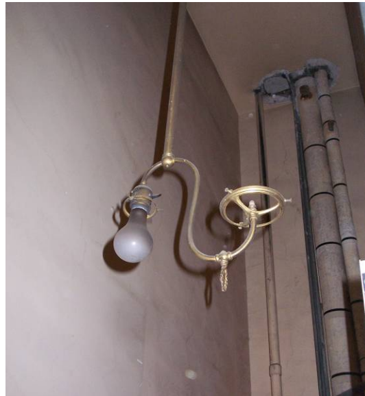
Figure 50. Gas-electric light fixture that appears to date from the 1907 reconstruction. Source: KVP 2009.
