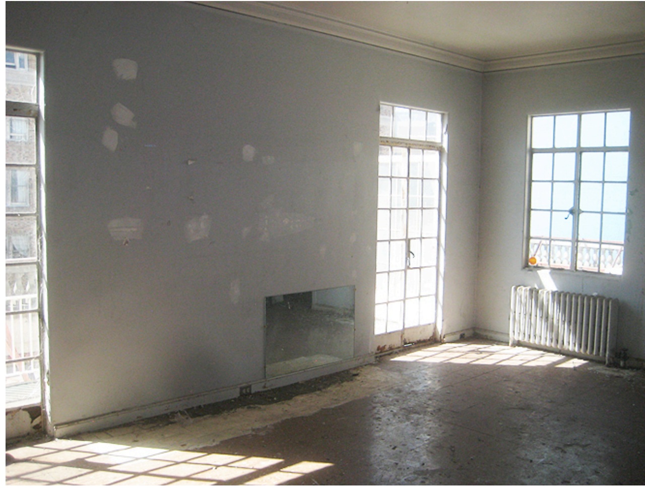
A: View of existing southern side of penthouse where existing pair of doors will be replaced by single exit door.
