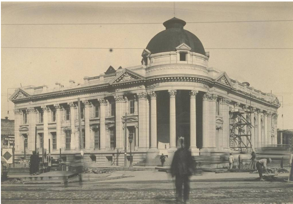
Item 19. Hibernia Bank Building during reconstruction, n.d. Source: Bancroft Library, University of California, Berkeley.
