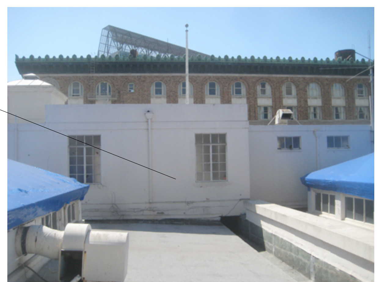
A: View of existing northern side of penthouse where window will be converted to exit door.
