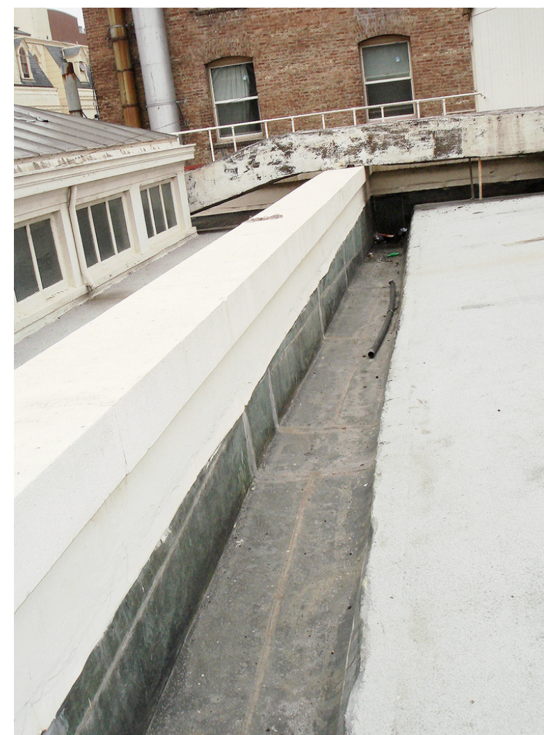
C: Detail of typical roof gutter. All gutters to be inspected and repaired.
