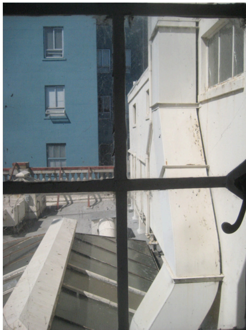
B: View along existing southern side of penthouse where an addition will house new bathrooms.
