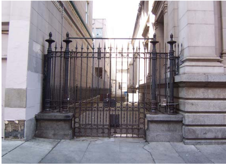
Figure 11. Cast iron and wrought iron security gate located just west of the building. Source: KVP 2009.
