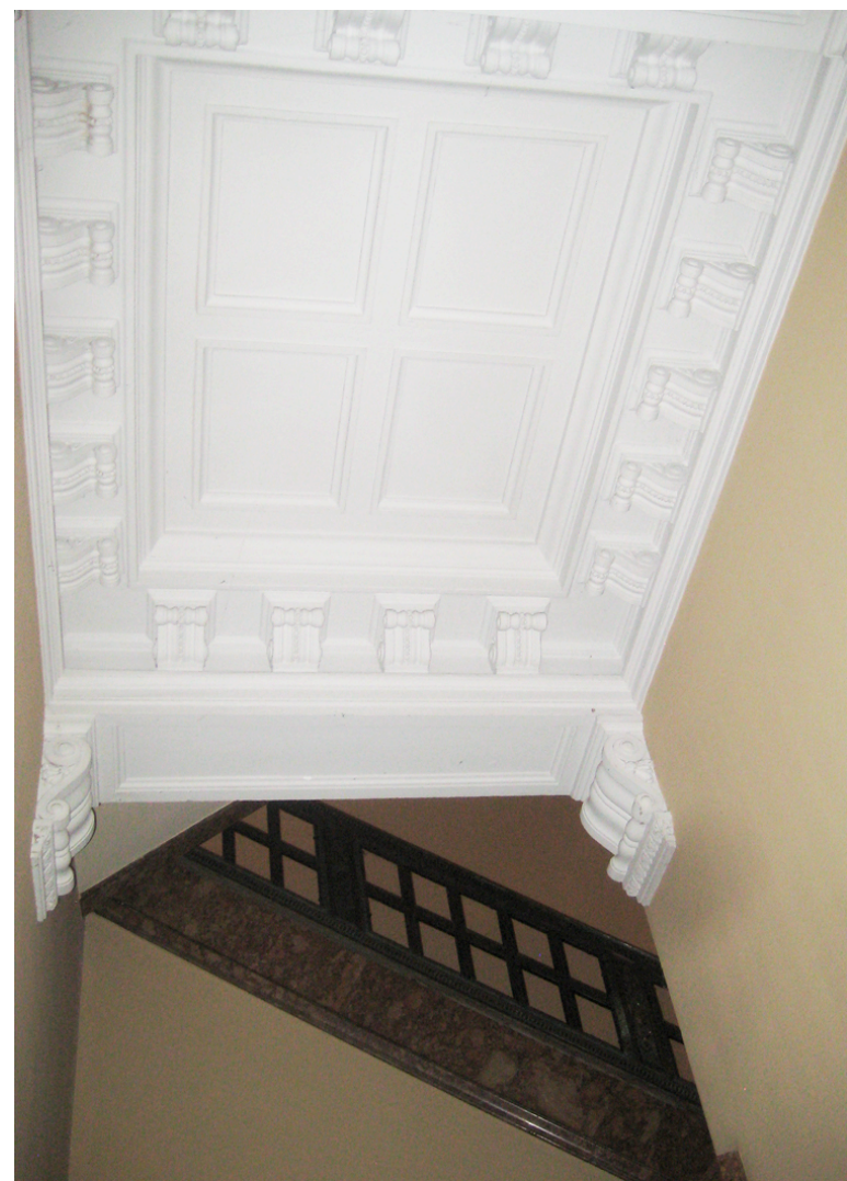
D: View of ceiling in in South Stair. Sprinkler head to be located at center point of coffers.
