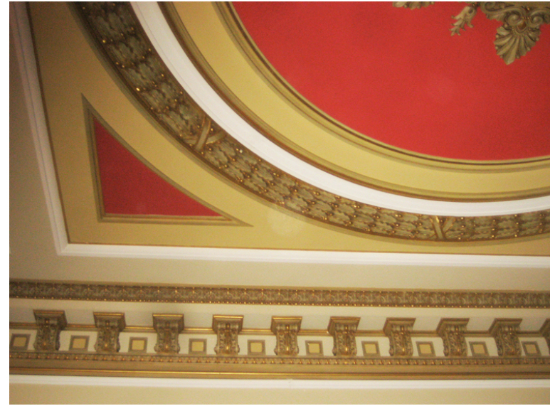
B: View of ceiling of SW Meeting Room. Sprinkler heads to be located at center point of triangular panels at corners of central circular panel.
