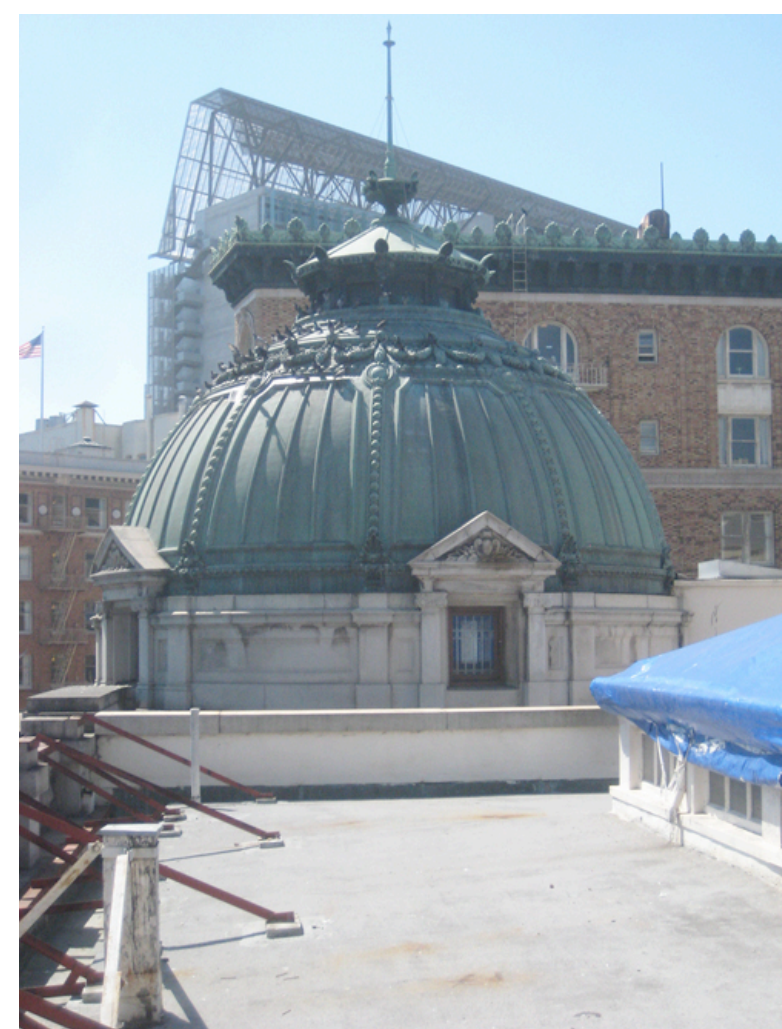
A: View of dome looking south with skylight enclosure on right. Parapet bracing on left.
