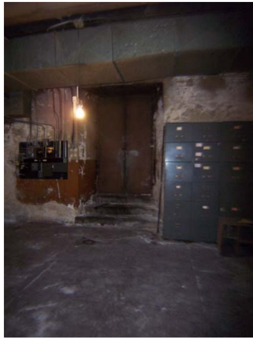
Figure 48. Mechanical Room (B-15) in the basement shows signs of bubbling and spalling plaster concentrated around the window and door openings. Source: KVP 2009.
