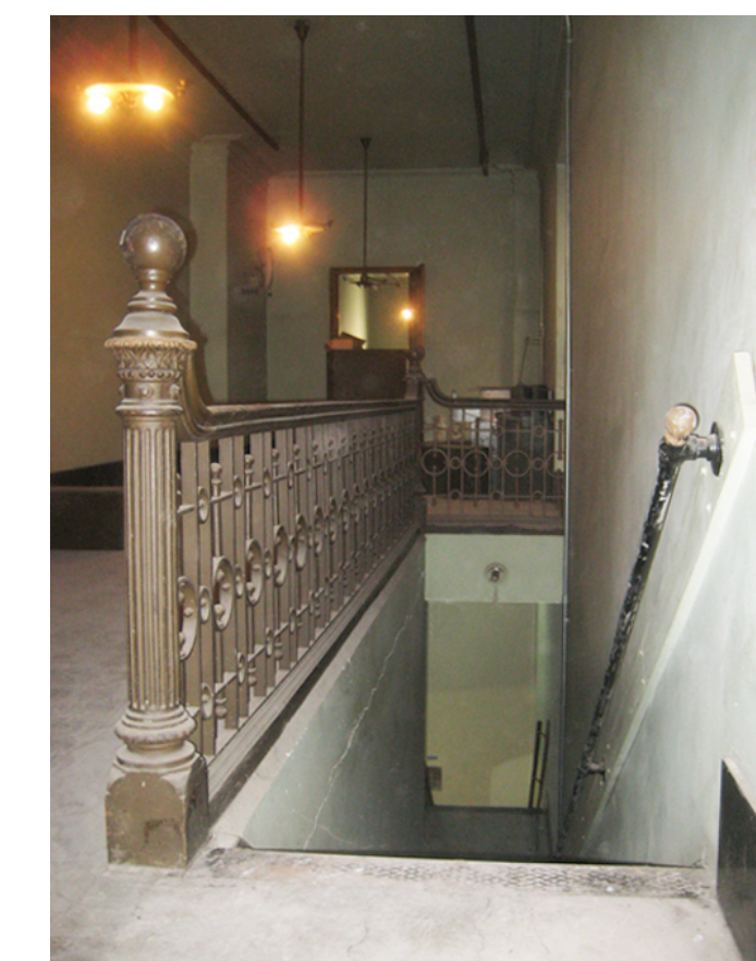
E: View of file storage room. New door at the base of stair to be relocated from demo'd bathroom at south side of 2nd floor.
