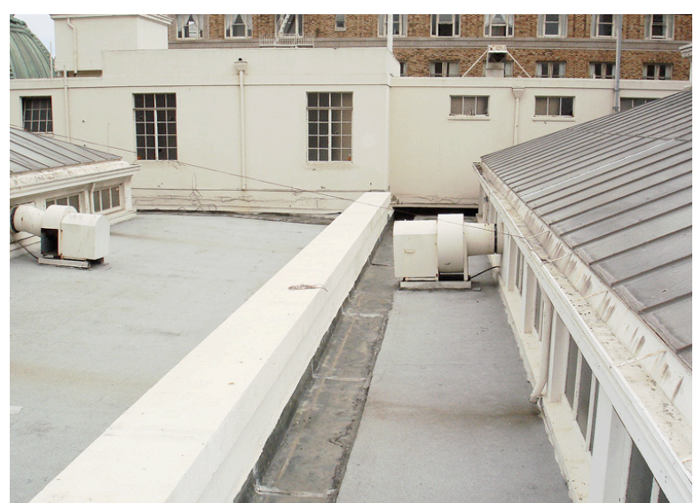
B: Looking south at Penthouse. Parapet at center is the structural line between the original building (on left) and the 1905 addition (on right).
