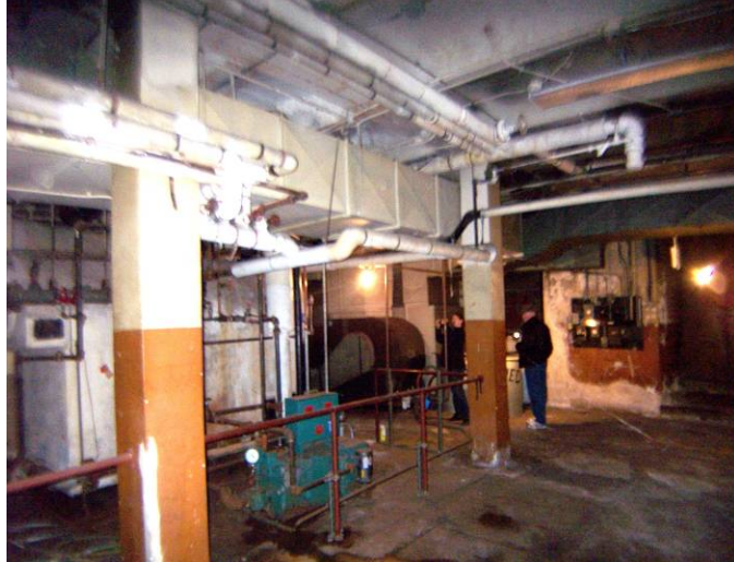
Figure 24. Mechanical Room (B-15) located in the basement. Source: KVP 2009.
