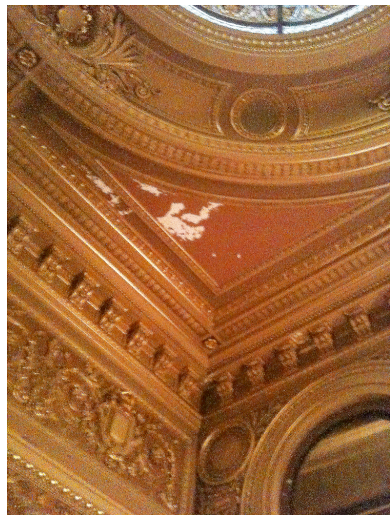
D: View of corner of Banking Hall ceiling in 1905 addition. Sprinkler heads to be centered in corner flat panels. No heads to be located within ornamental panel or trim.
