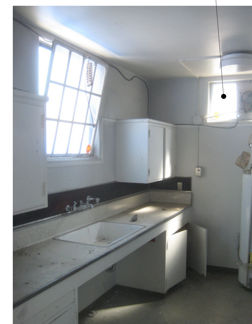
C: View of window on western wall to be enlarged to match adjacent window size
