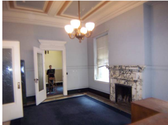
Figure 45. Chairman's Office (S-15) located on the second floor south. Note historic light fixture. Source: KVP 2009.
