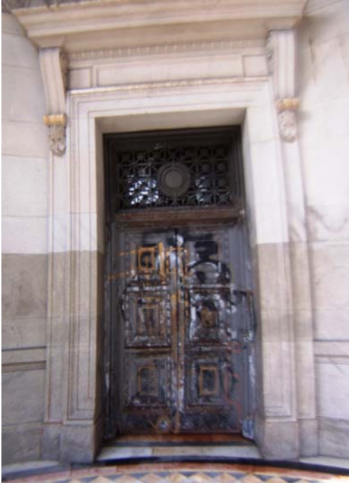
Figure 54. Bronze-plated steel outer door at the private entrance. There are similar doors at the main and Jones Street entrances. Source: KVP 2009.
