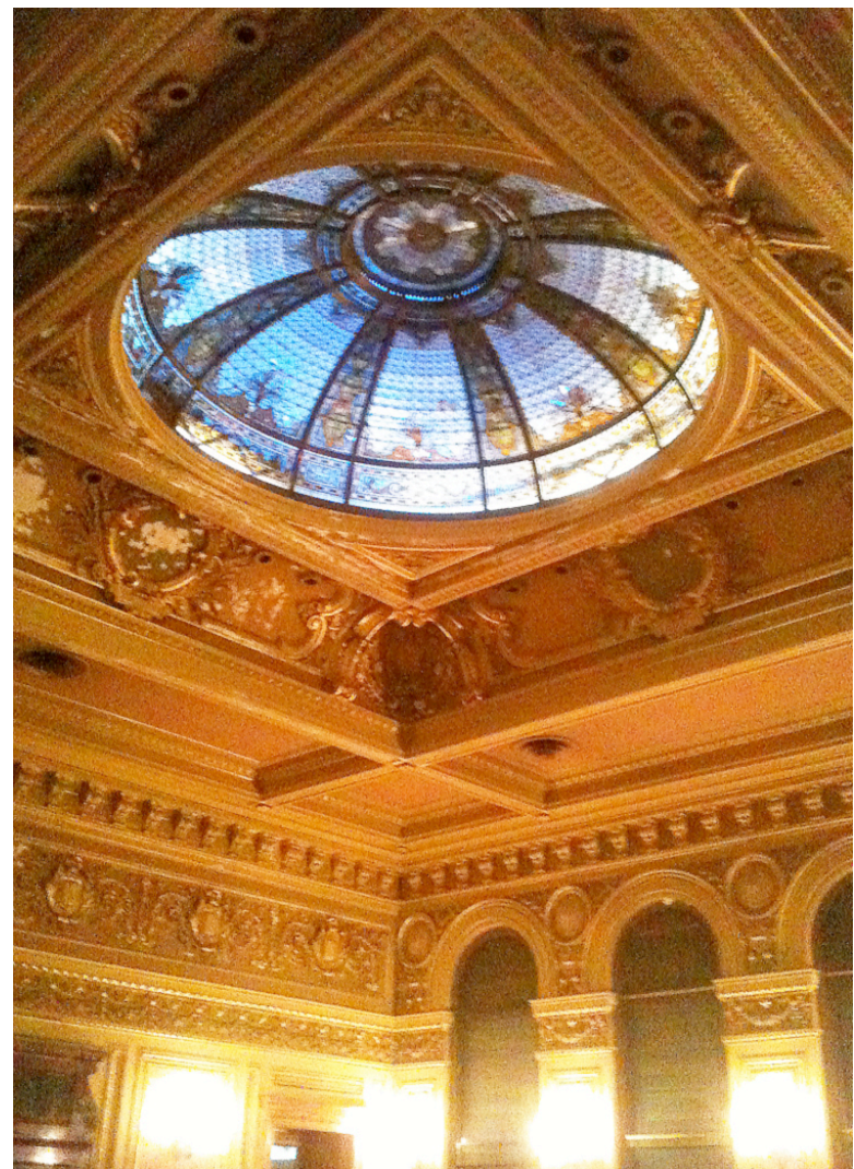
E: View of Banking Hall ceiling in original building. Sprinkler heads to be located only in flat panel areas. No heads to be located within ornamental panel or trim.
