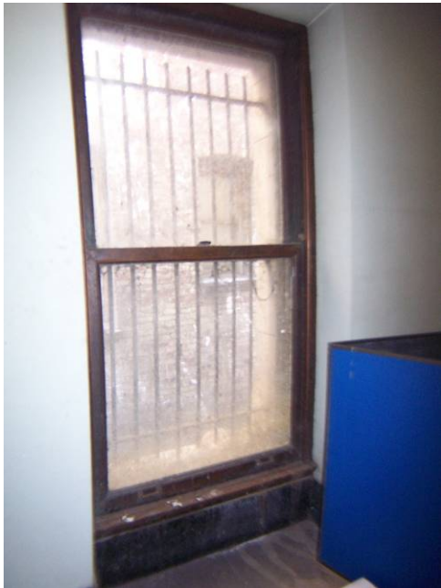
Figure 53. Typical double-hung, sheet bronze over steel sash window that dates from the 1907 reconstruction. Source: KVP 2009.
