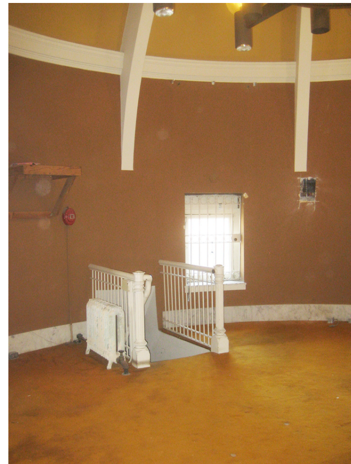
C: View into Dome Room showing existing stair to be removed. Renovations to room from 1977 to be removed.
