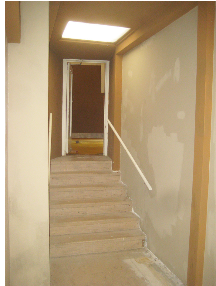
B: View of hall at Dome Room. Ceiling to be raised 2'-0" and foreground of picture to be inside new South stair exit.
