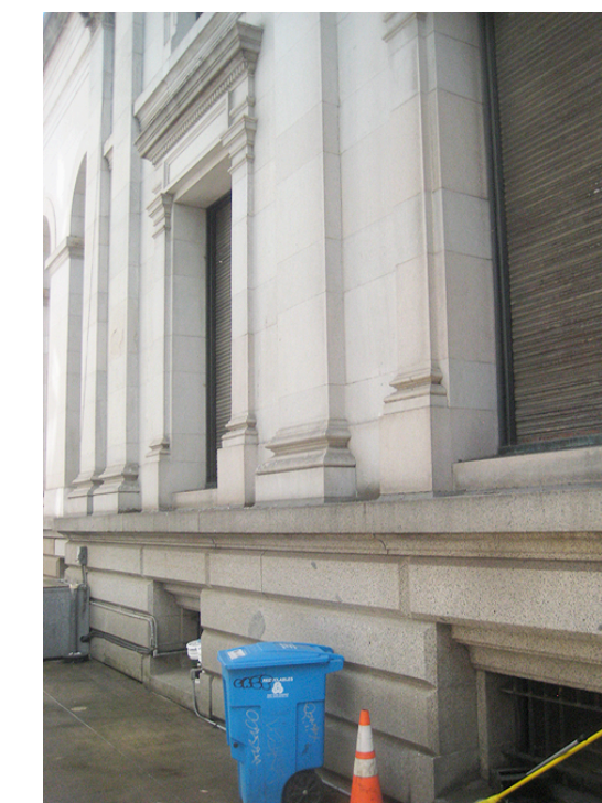
A: View of window to become west exit door from main space.
