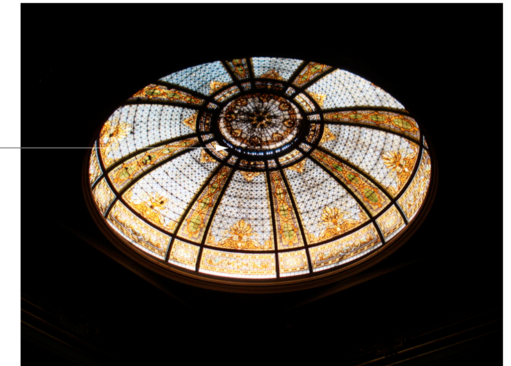
F: View of skylight dome located in the original portion of the Banking Hall. Sprinklers to be located behind circular vent grille to be able to protect glass and leading by bathing surface with water to keep dome intact.
