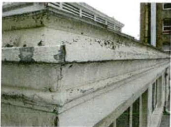
B: Detail of skylight enclosure. Metal to be repaired and repainted.
