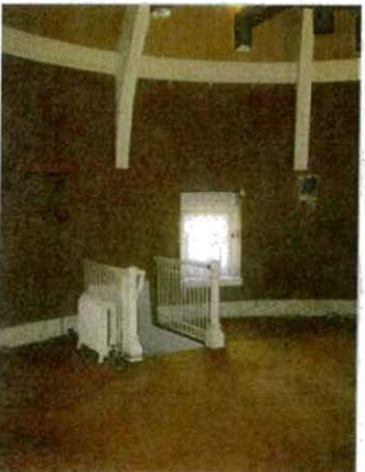
C: View into Dome Room showing existing stair to be removed. Renovations to room from 1977 to be removed.
