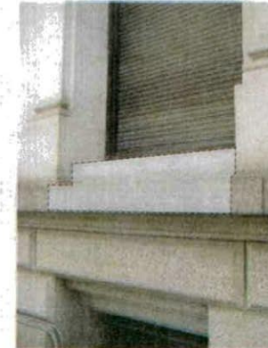
B: AREA OF MATERIAL TO BE CUT FOR NEW WEST EXIT. MATERIAL TO BE RETAINED ON SITE FOR POSSIBLE REUSE. SEE PAGE 6 FOR STORAGE LOCATION.
