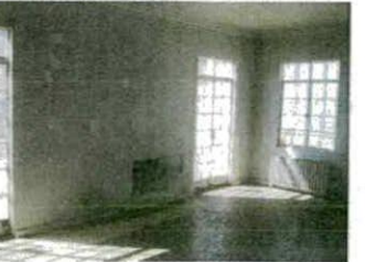
E: View of Penthouse Room to be repaired and renovated. Original steel windows to be replaced with steel single panel French doors.
