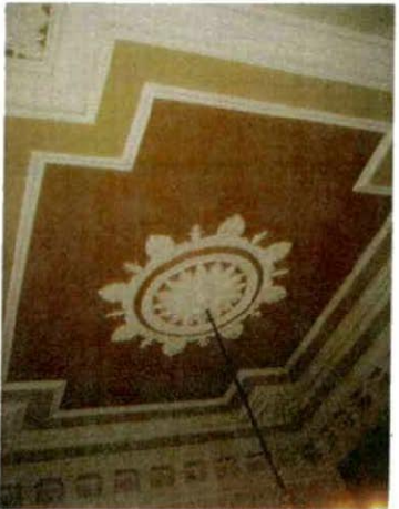
C: View of ceiling in Middle Office. Sprinkler heads to be located on either side of central rondel.
