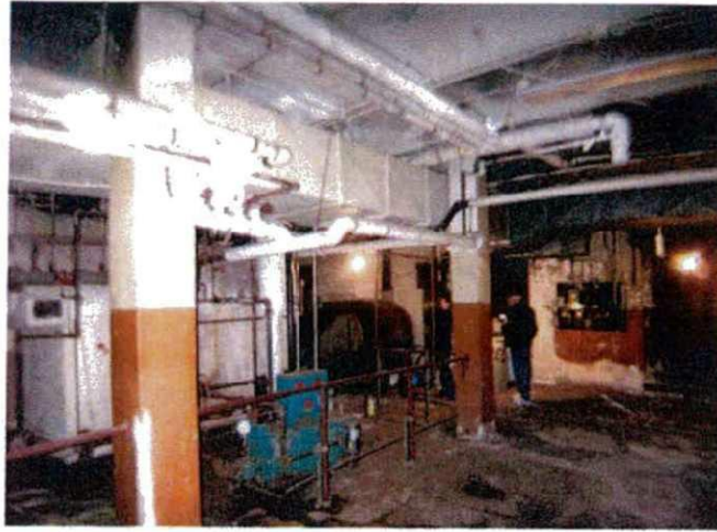
Figure 24. Mechanical Room (B-15) located in the basement. Source: KVP 2009.
