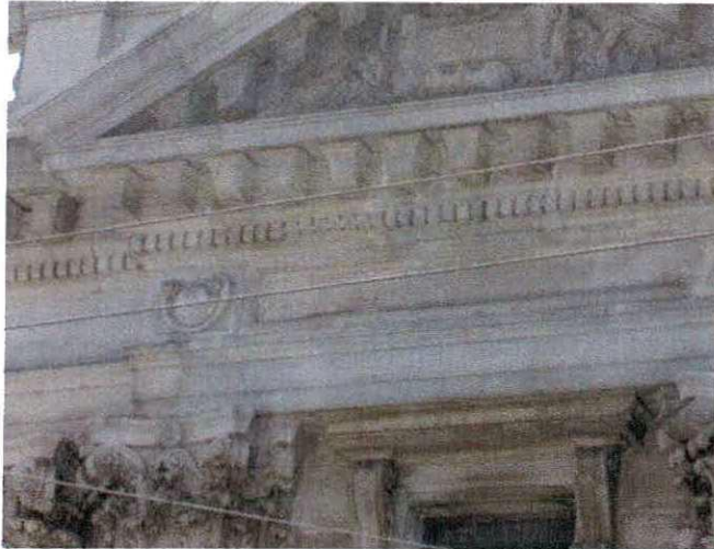
Figure 19. One of two areas of broken dentil molding on the east facade
