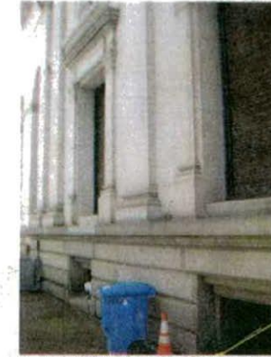
A: VIEW OF WINDOW TO BE MODIFIED FOR NEW EXIT AT CUSTOMER WAITING AREA. MATERIAL TO BE CUT IS IDENTIFIED.
