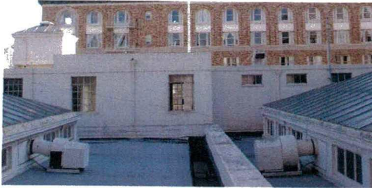
Figure 18. Roof, view south. Note the skylight diffusers at left and right and the penthouse in the background. Source: KVP 2009.
