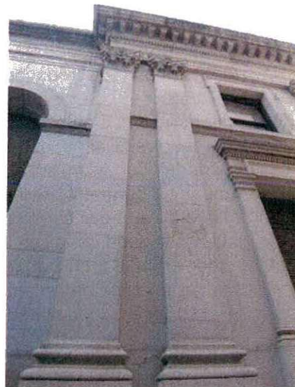
Figure 20. Spalling granite on west facade. Source: KVP 2009.
