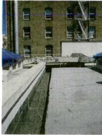
A: View across roof to mechanical penthouse. New metal walkway and north stair penthouse to be built in this location.
