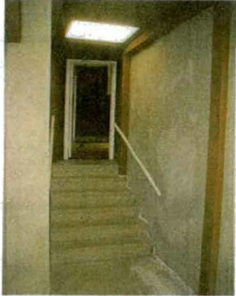
B: View of hall at Dome Room. Ceiling to be raised 2'-0" and foreground of picture to be inside new South stair exit.
