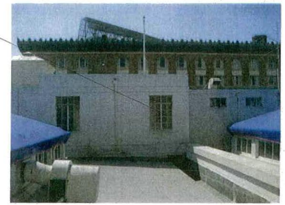
A: View of existing northern side of penthouse where window will be converted to exit door.
