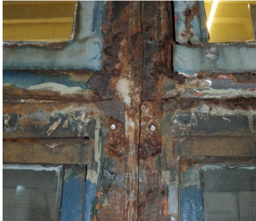
Corrosion beneath cover plate
