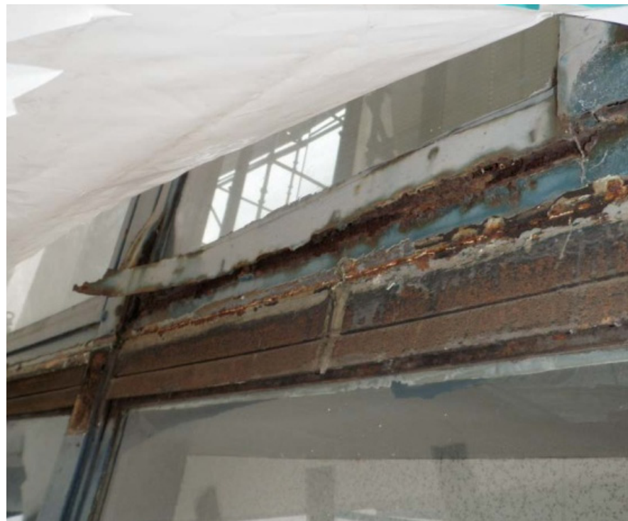
Corrosion at window
