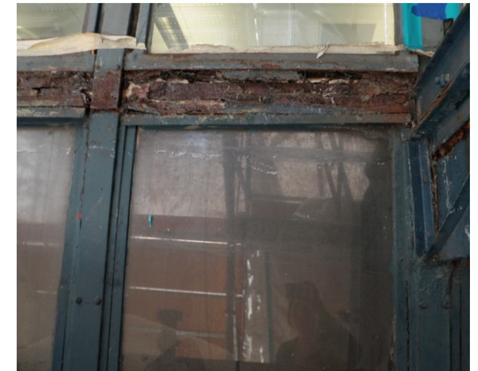
Corrosion at curtain wall
