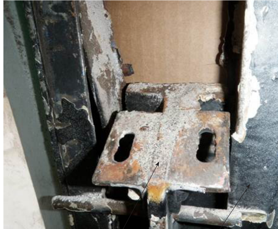
existing T-mullion at vertical spans of curtain wall existing windows on each side
