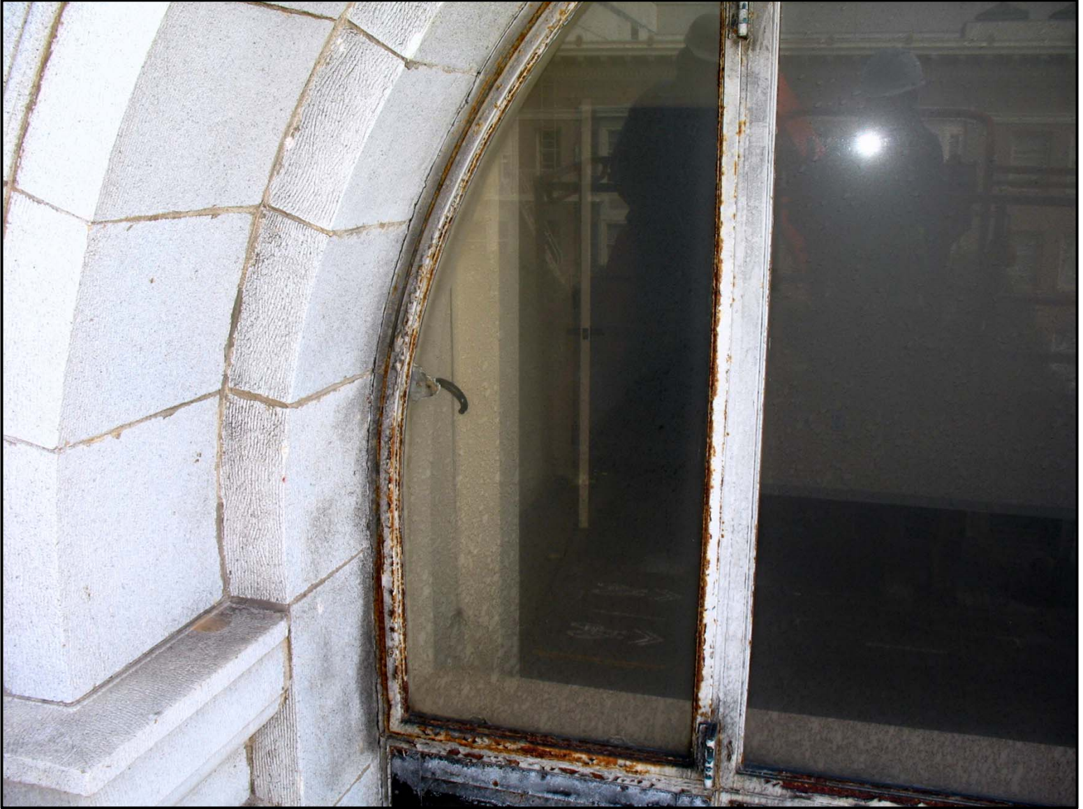
Veterans Building, View of Deteriorated Window Frame
