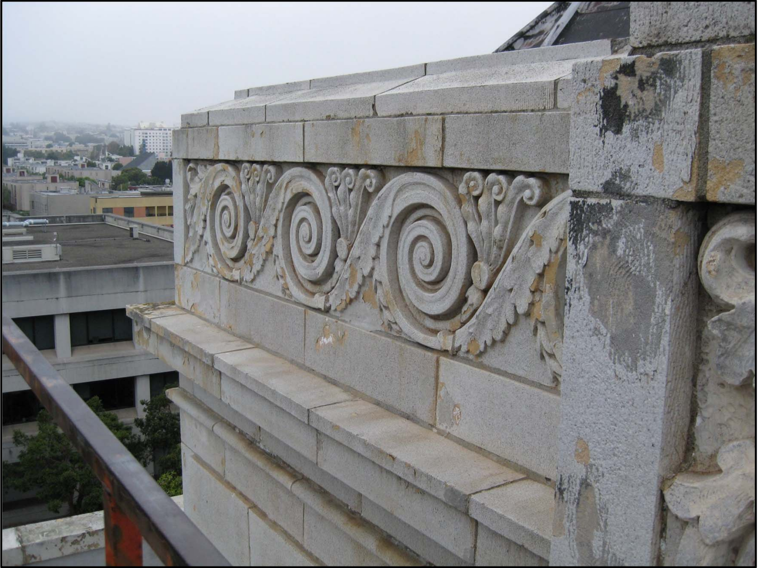
Veterans Building, View of Glaze Spalling in Frieze
