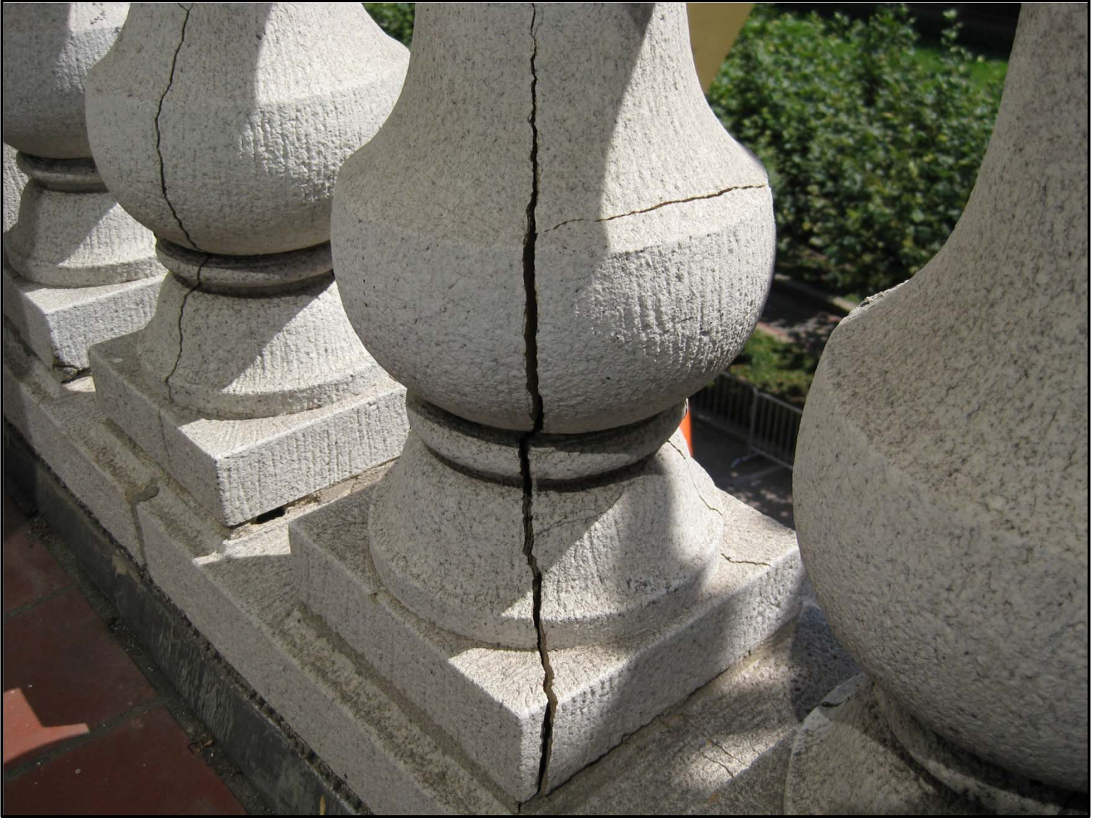
Veterans Building, View of Cracked Balustrade
