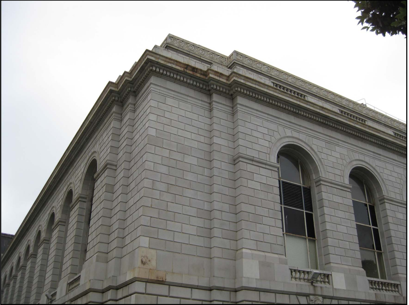
View of Veterans Building, Northwest Corner, Rust Staining
