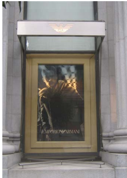
Existing window with film to receive new film. Dark window frame to be repainted, stainless steel elements to be repainted in gloss black. Source: Page & Turnbull
