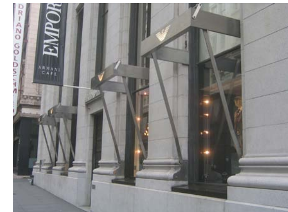
Dark window frame to be repainted, stainless steel elements to be repainted in gloss black. Banner to be replaced, banner support elements to be repainted in gloss black. Source: Page & Turnbull
