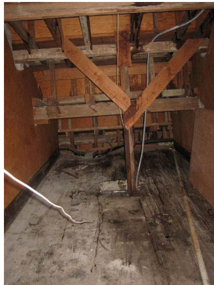
Figure 23. Wood supports under balcony. View from second floor hallway. Source: Page & Turnbull, Oct 2007.
