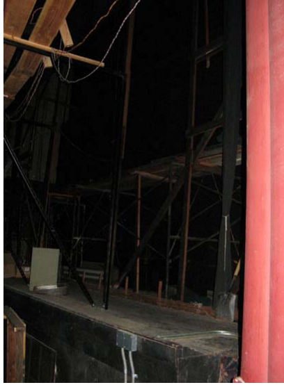
Figure 14. Backstage area. Detail of stage, old screen support trusses, and 1941 proscenium. Source: Page & Turnbull, Oct 2007.
