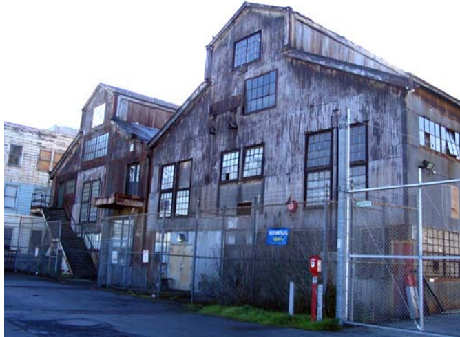
Figure 13. Building #21 at Pier 70, built in 1900, “was probably originally constructed by Pacific Rolling Mills.” Source: Port of San Francisco web site, 2011.
