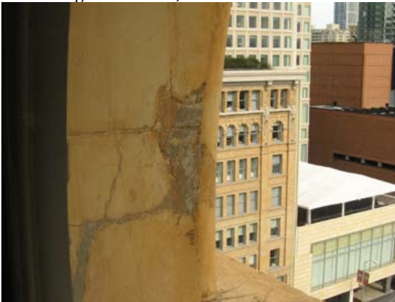
Figure 56. Previous repair. Source: Page & Turnbull, March 2010.
