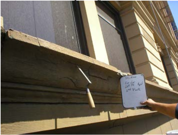
Figure 50. Cracking of sandstone. Source: Rainbow Waterproofing, 2006.
