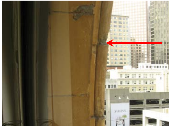
Figure 53. Shallow bisque spalls at joints. Source: Page & Turnbull, March 2010.
