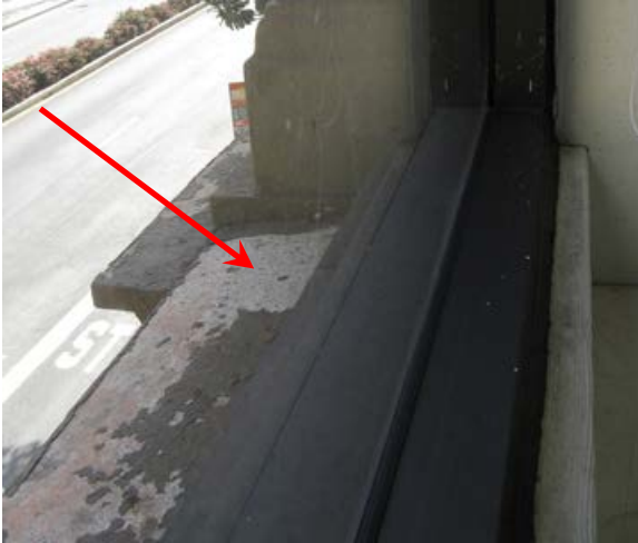
Figure 62. Area of exposed cast iron with no paint. Source: Page & Turnbull, March 2010.
