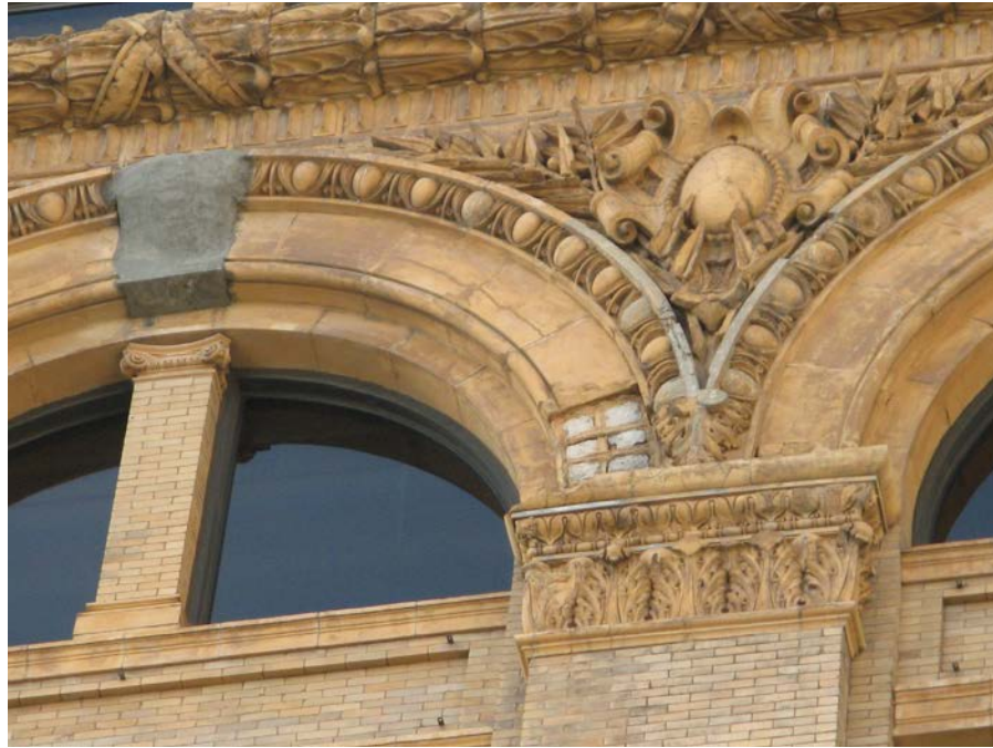
View of temporary terra cotta repair
