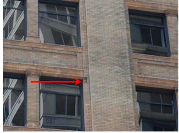
Figure 59. Missing brick. Source: Page & Turnbull, March 2010.
