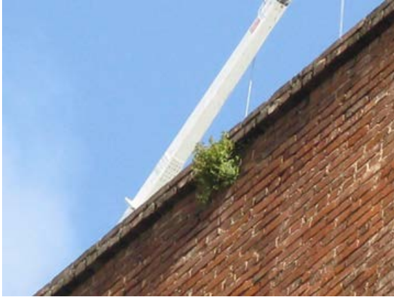
Figure 37. Weeds growing out of a parapet wall. Source: Page & Turnbull, March 2010.
