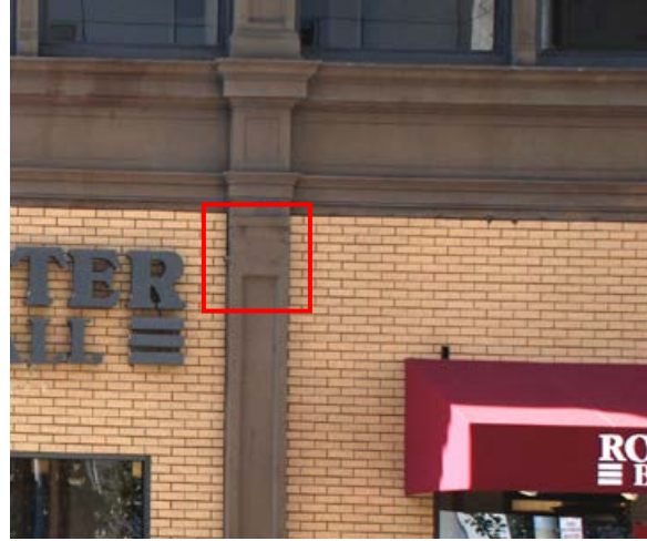
Figure 63. Missing scroll at column capital on 3 rd Street facade. Source: Page & Turnbull, March 2010.
