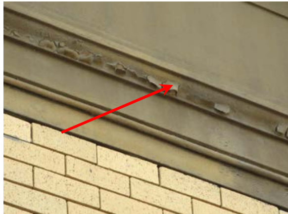
Figure 61. Delaminating paint. Source: Page & Turnbull, March 2010.
