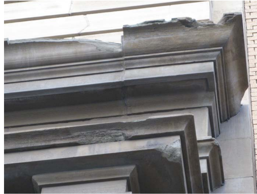
View of deteriorated colusa sandstone
