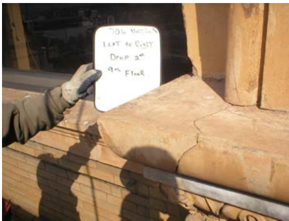
Figure 44. Cracking at cornice. Source: Rainbow Waterproofing, 2006.
