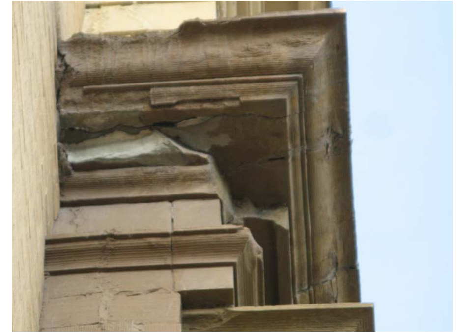
View of deteriorated colusa sandstone
