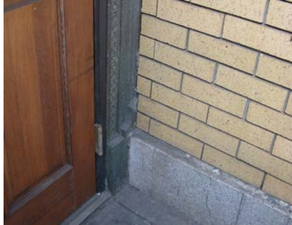
Figure 65. Corrosion of bronze frame. Source: Page & Turnbull, March 2010.
