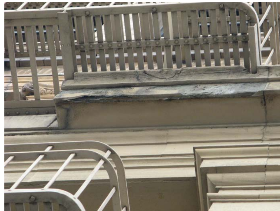
View of deteriorated colusa sandstone
