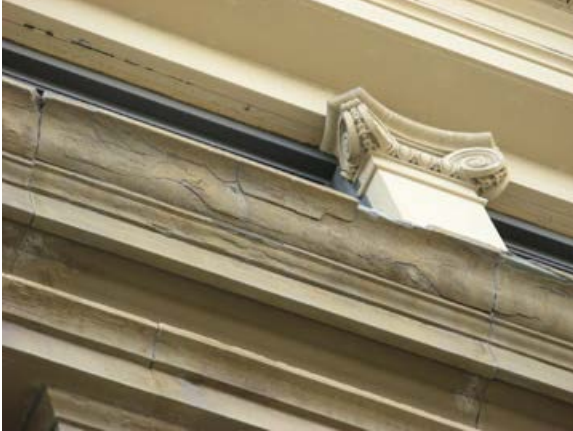
Figure 39. Cracking and spalling of sandstone at edge. Source: Page & Turnbull, March 2010.
