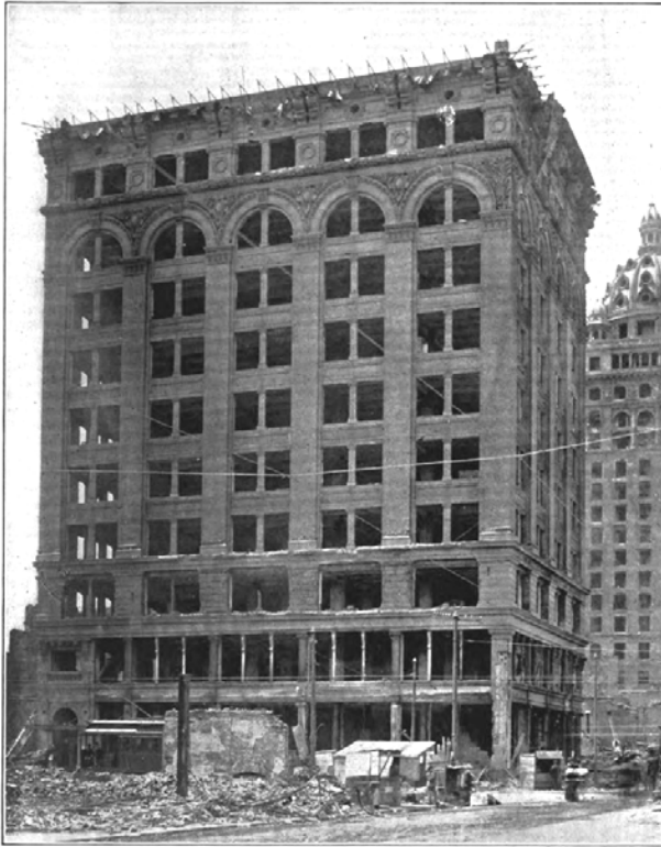
Figure 12. The caption to this 1906 newspaper photo reads: "ARONSON BUILDING. Northwest Corner Third and Mission Streets. The facades for the three lower stories consist of Colusa sand-stone, which is badly spalled and damaged. The upper stories of buff terra cotta pressed brick, with terra cotta ornaments, are but slightly injured, the terra cotta being spalled and cracked in a few places. The metal cornice is completely wrecked. The rear walls of common brick were considerably racked and damaged by the earthquake. All the walls remain practically plumb. Columns in the basement, first, fifth, eighth and tenth stories have buckled on account of the failure of the hollow tile protection. The Roebling concrete floors, with crimped wire lath and cement plastered soffit protection, remain in first-class condition throughout, notwithstanding the warped condition of the steel work, due to the buckling of the columns. The 4" hollow tile partitions are badly wrecked throughout, about 80 percent of the entire work having fallen down. The failure of the hollow tile partitions totally wrecked the cast-iron and marble tread stairways." Source: Unknown (clipped file).
