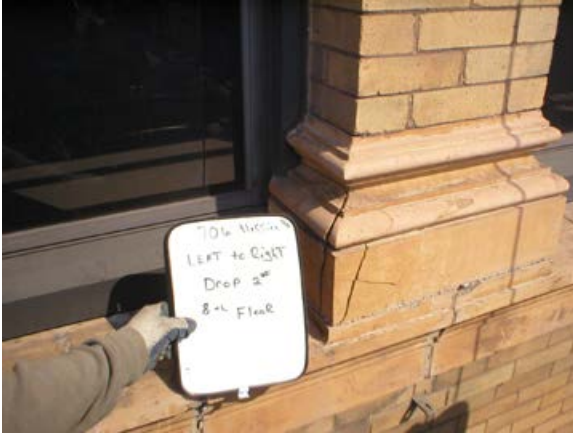
Figure 46. Cracking at column base. Source: Rainbow Waterproofing, 2006.
