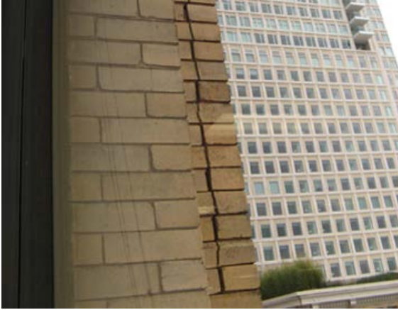
Figure 58. Cracking at column corner. Source: Page & Turnbull, March 2010.
