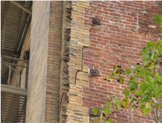
Figure 35. Cracking at terra cotta to brick interface. Source: Page & Turnbull, March 2010.
