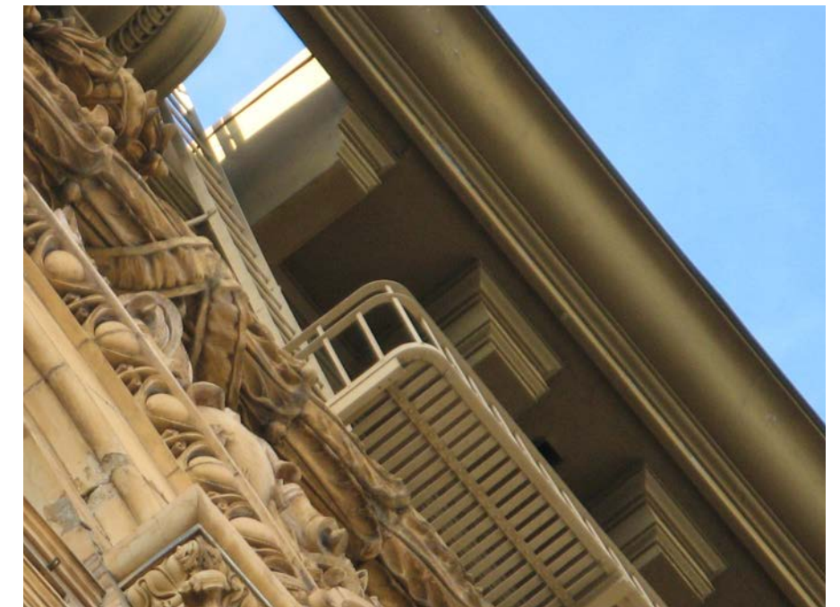
View of area where fire escapes will be removed, sheet metal cornice to be repaired
