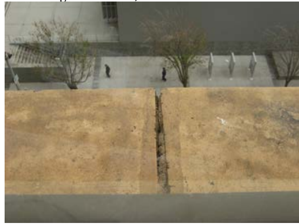
Figure 57. Cracking and missing mortar at sill joint. Source: Page & Turnbull, March 2010.
