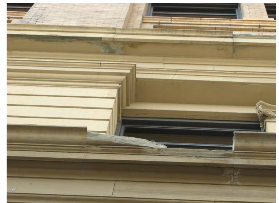
View of deteriorated colusa sandstone
